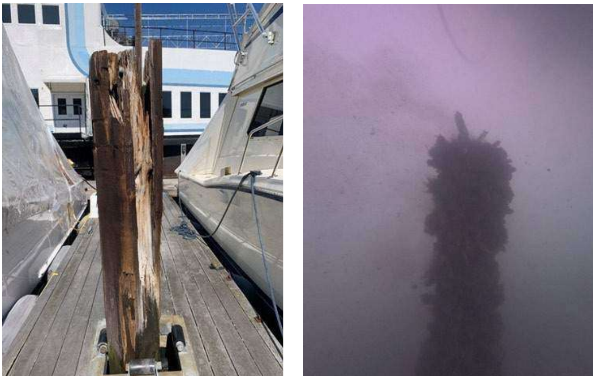
Figure 3-4. Additional examples of rot/deterioration and cut off timber pile beneath float
