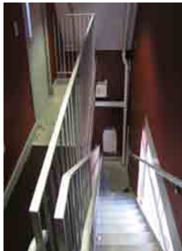
Stair tower is in need of attention
