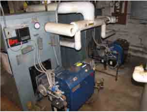
Gas fired heating units
