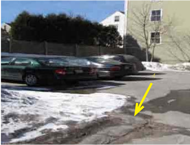
Missing and cracking curbing for this curbed area
