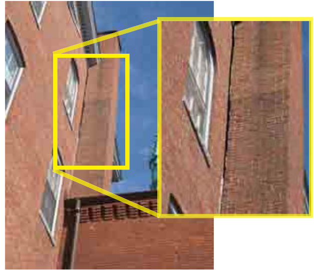
The chimney appears to be pulling away from the main structure.
