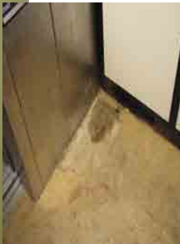
Moisture damage present floor repair needed and investigation into source of moisture recommended.
