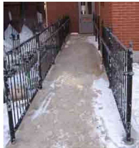
Ramp in good shape and meets ADA needs, but in need of re-painting.
