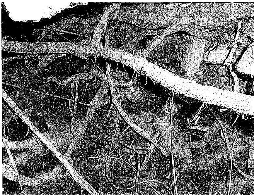
Photo 4 – Root Growth in Void
