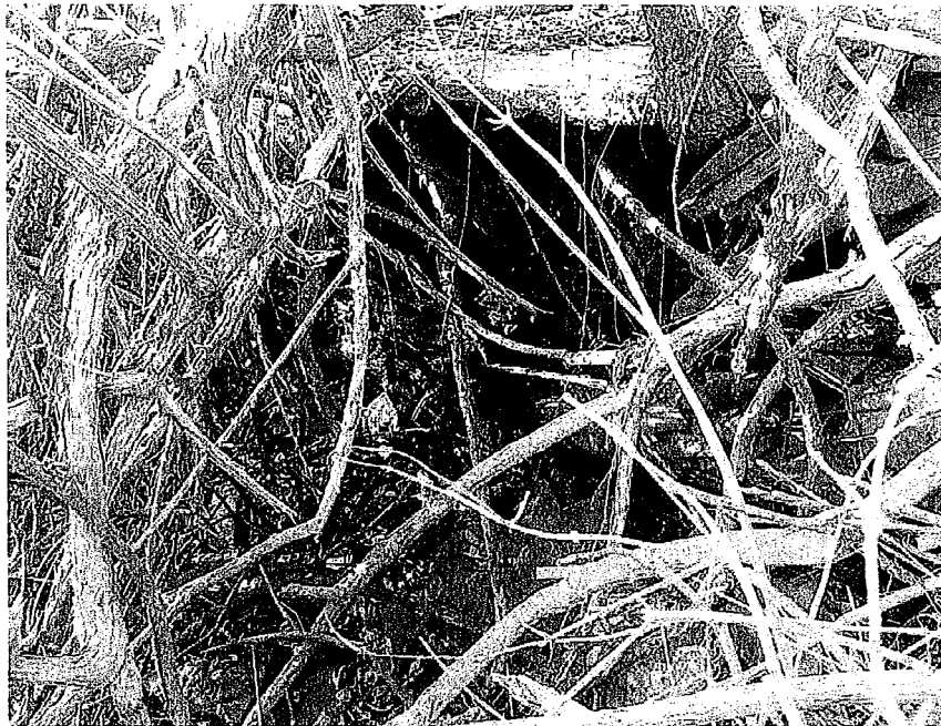
Photo 3 – Partially Collapsed Section and Void
