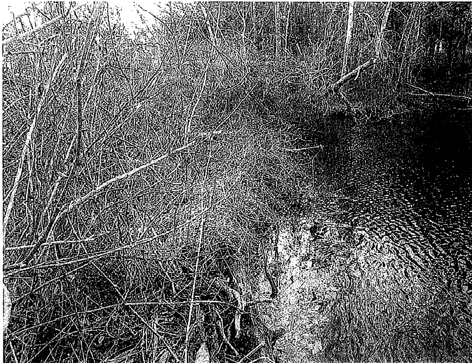
Photo 7 – Overgrown and Deteriorated Crest Above Void
