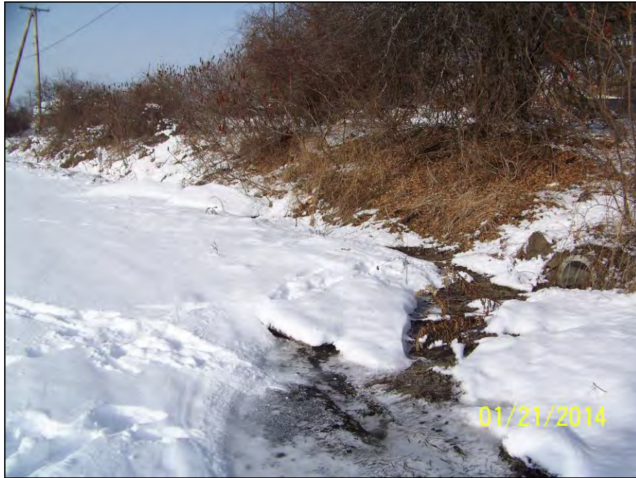
Figure 6 – Picture of drainage feature from Commercial Street. Pipe outlet is to the right and water flow from the pipe is evident by melted snow and ice.
