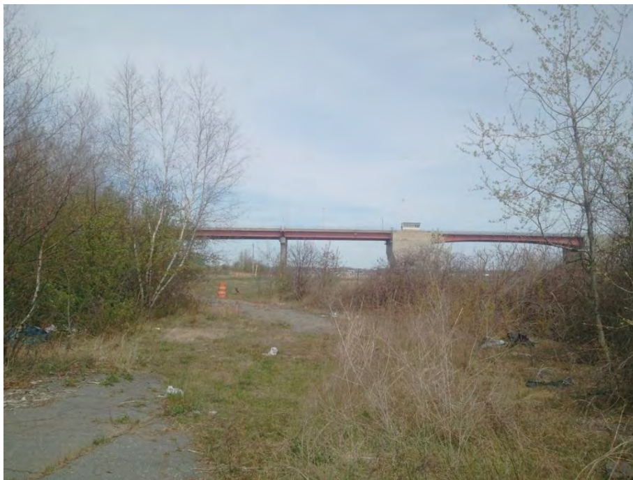
Vegetation overgrowth on abandoned paved road, small tree growth
