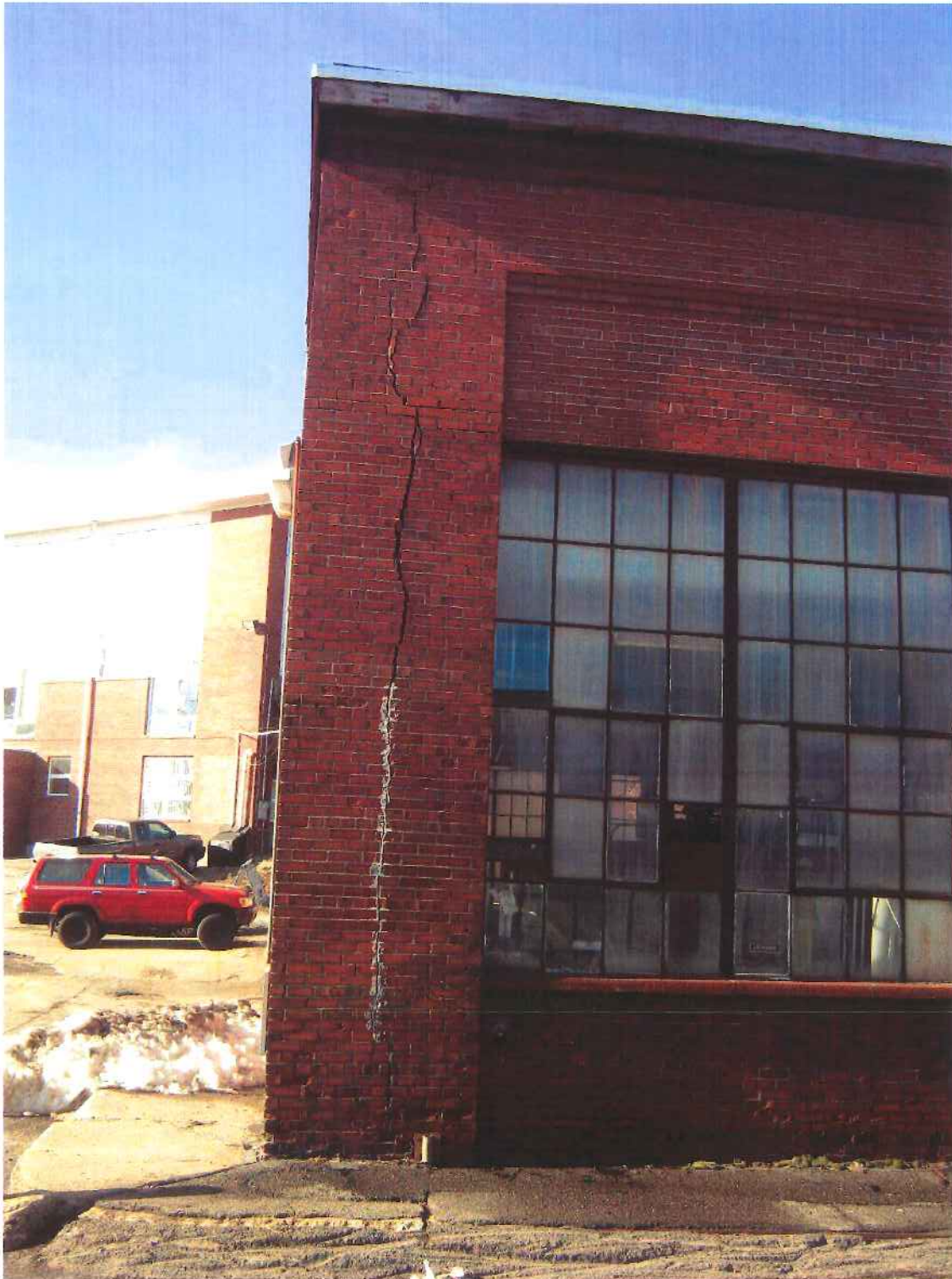
Photo 1-4: Vertical brick masonry crack at southwest pilaster.
