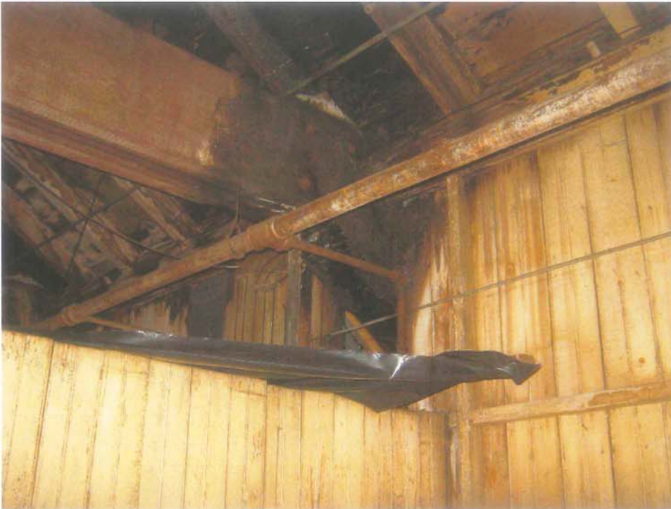
Photo 2-3: Charring of truss top chord.
