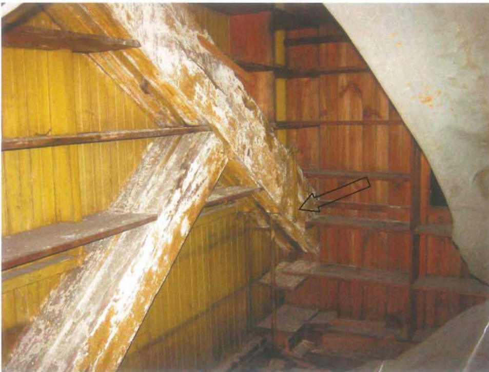
Photo 2-4: Broken truss hanger saddle hanger.
