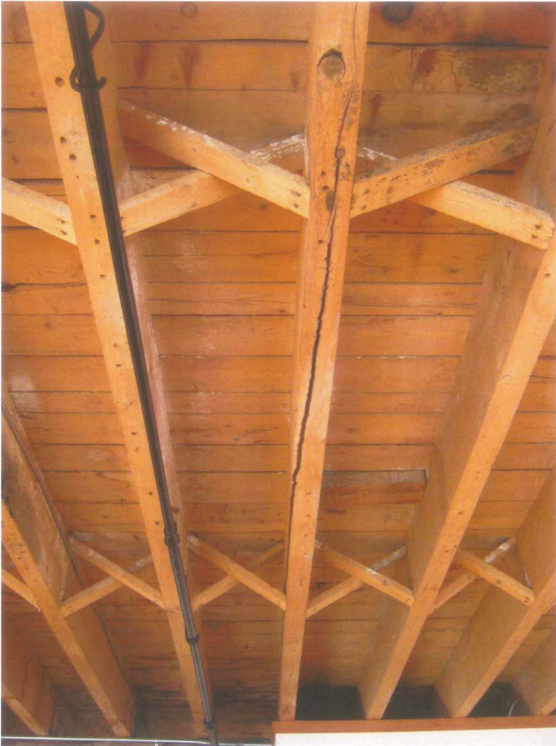
Photo 6A-4: Floor joist splitting.
