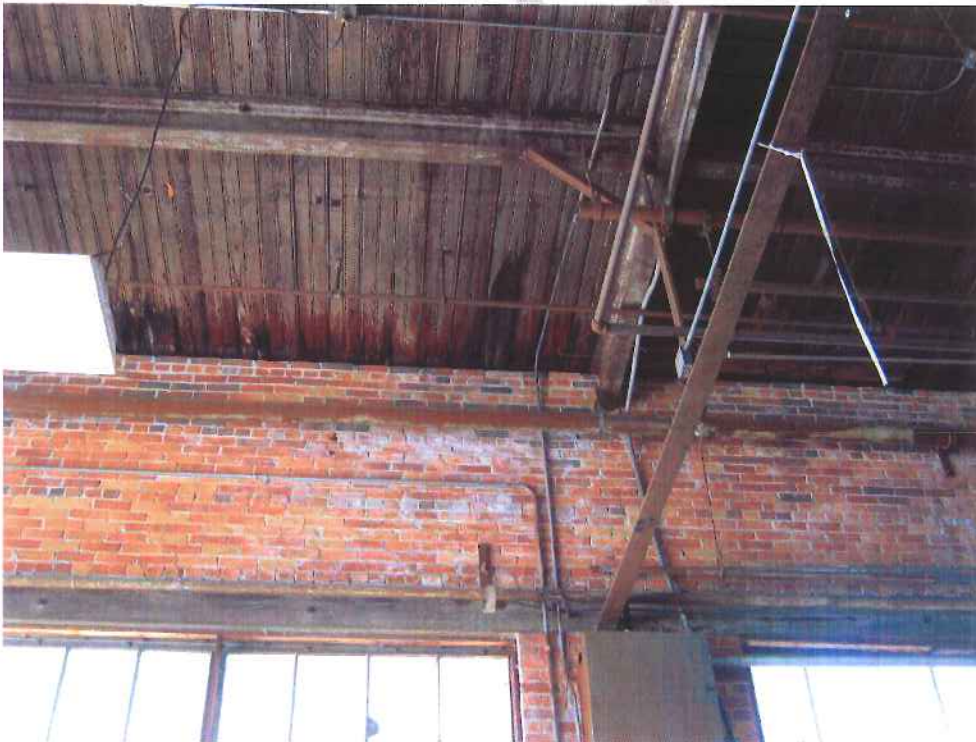
Photo 1-2: Wood deck condition at eave.
