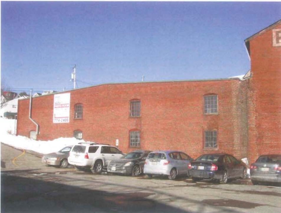
Photo 11-2: West elevation of Building 11. Note drainage condition where building 11 meets building 12.
