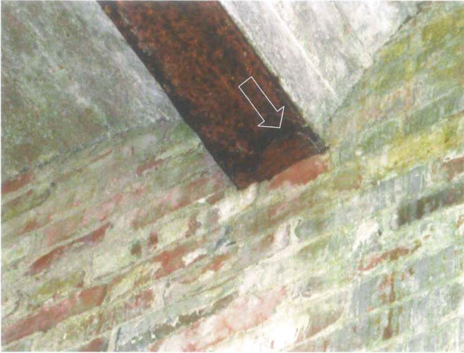
Photo 58-3: Beam end condition with flaking rust.
