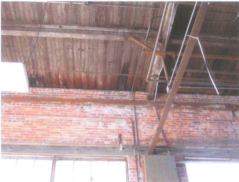
Photo 1-2: Wood deck condition at eave.
