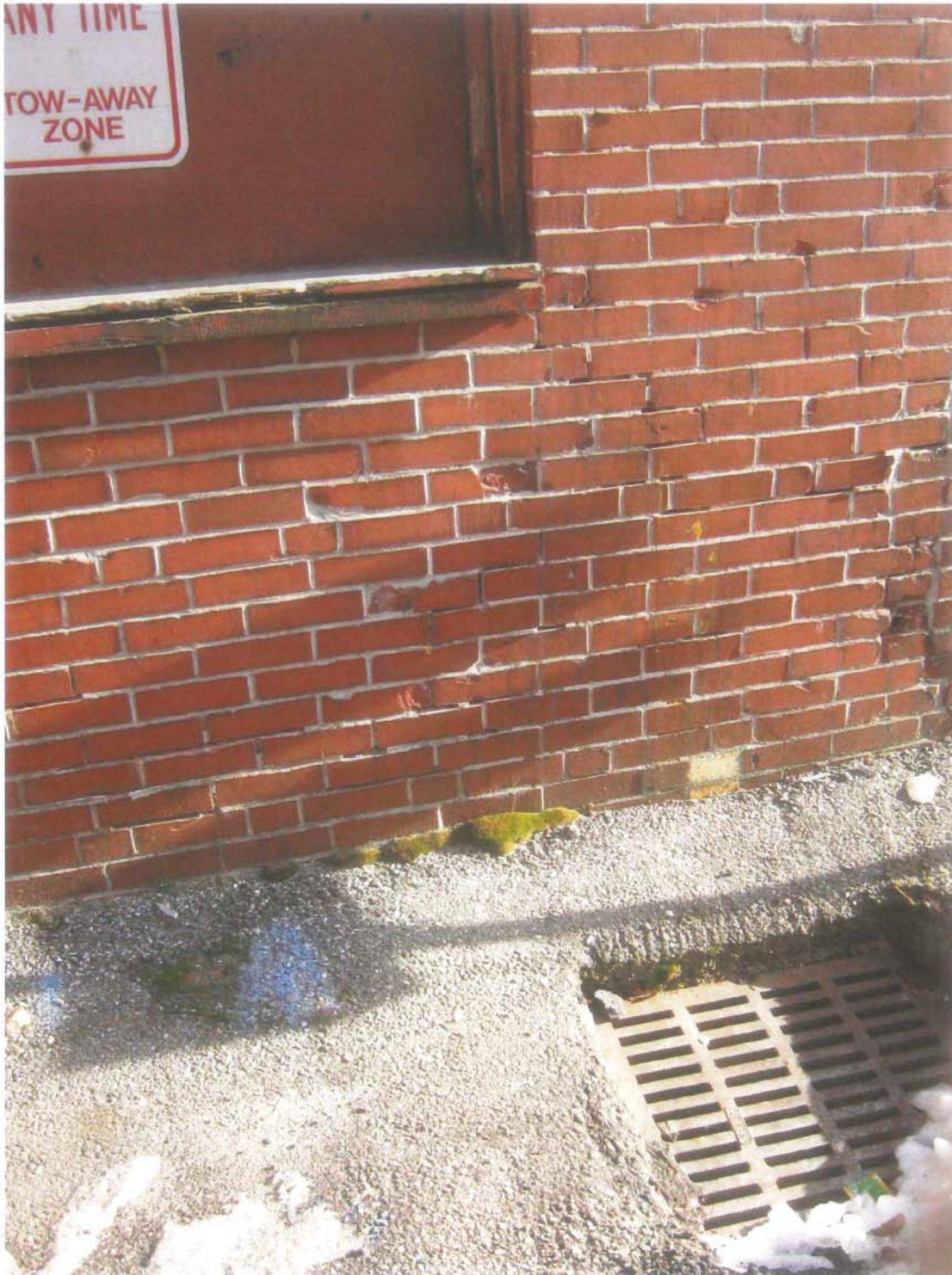
Photo 6A-6: Moss, spalled bricks, open masonry joints and rotting wood sill at Building 6A.
