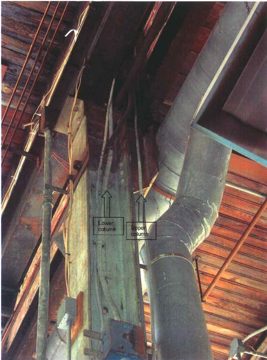
Photo 1-5: Column discontinuity at low-high roof condition.
