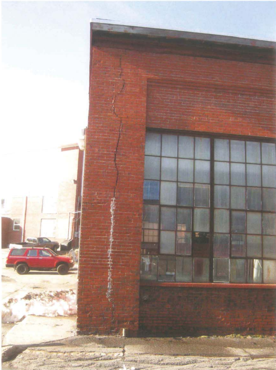
Photo 1-4: Vertical brick masonry crack at southwest pilaster.
