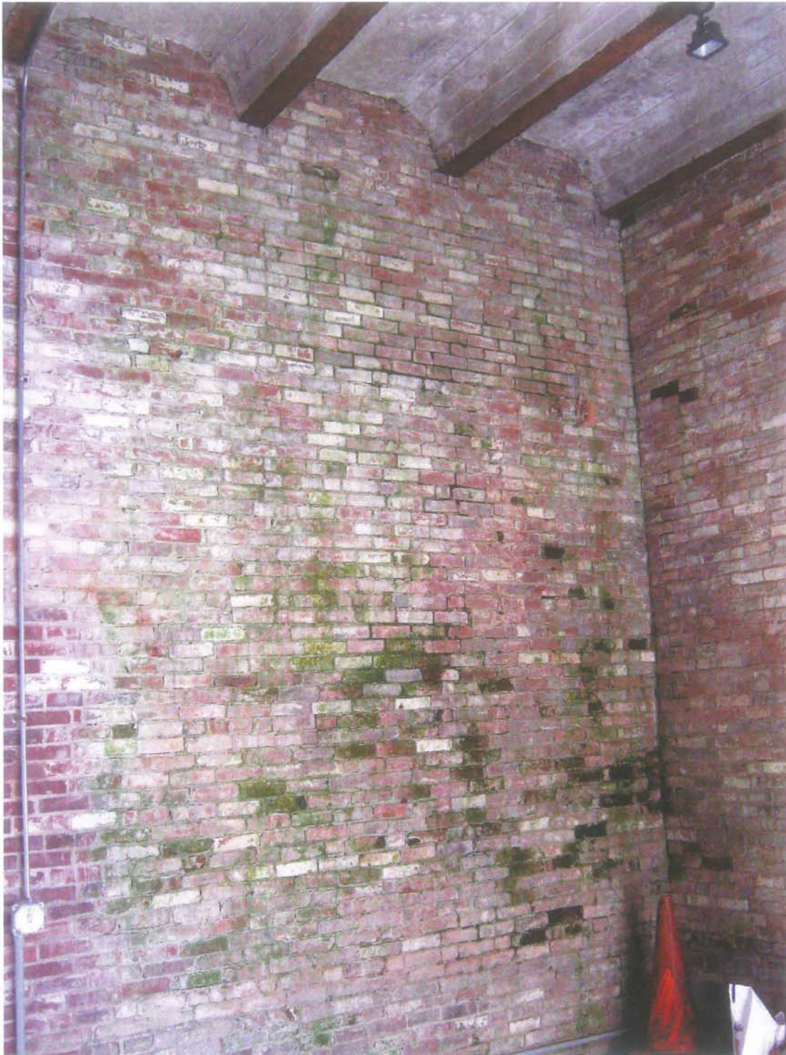
Photo 58-1: Moss growing on interior walls.
