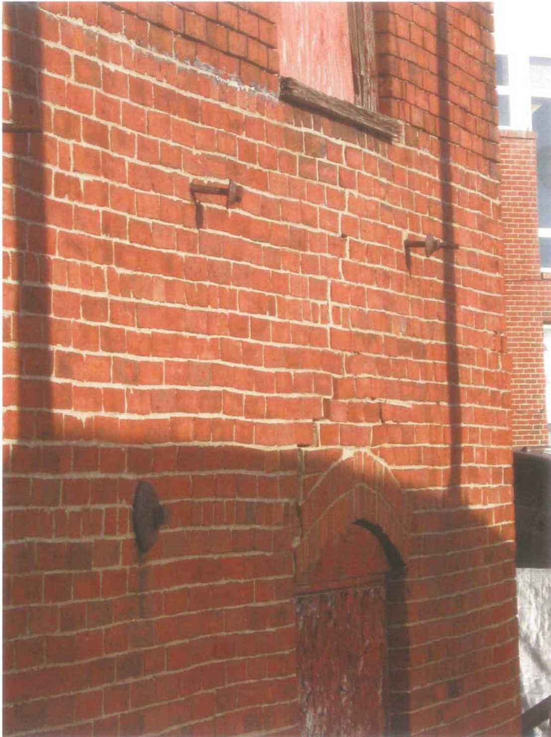
Photo 12-5: Diagonal masonry cracking over window opening, open joints, rotting window sill.
