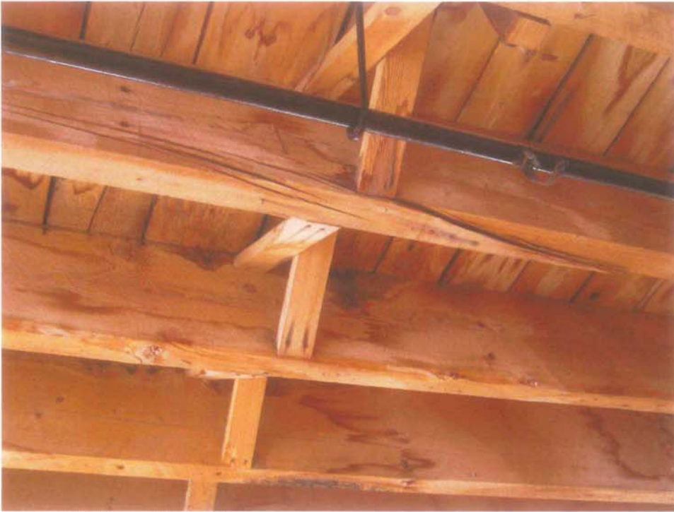
Photo 6A-3: Floor joist splitting.
