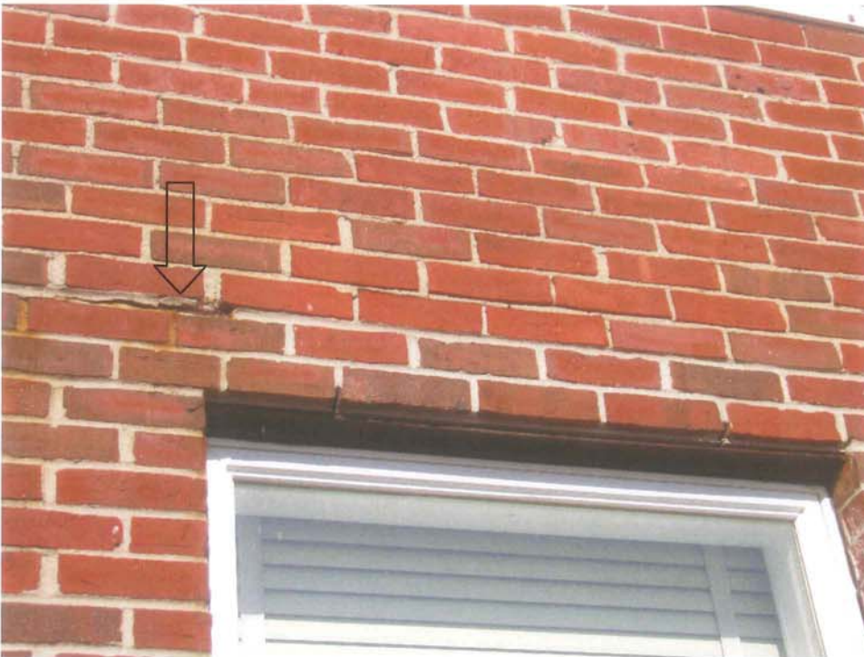
Photo 30-4: Mortar falling from joint with steel protruding; corroded steel lintel and broken mortar adhesion.
