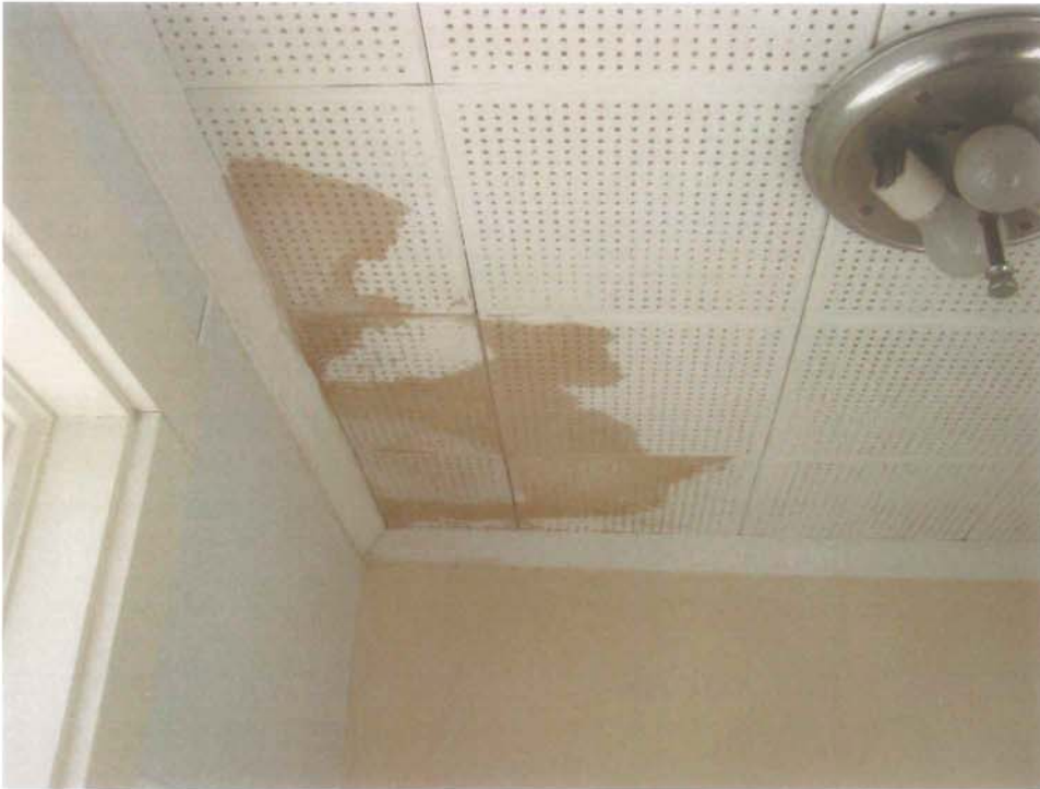
Photo 30-3: Leaking noted at ceiling adjacent to southwest wall.
