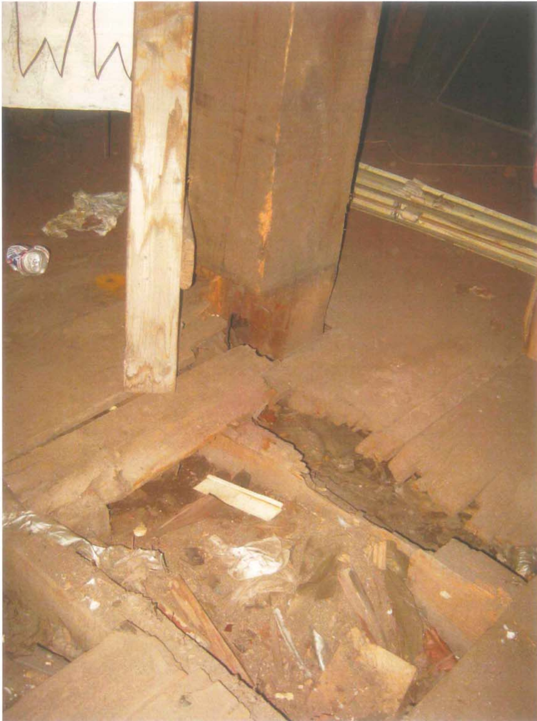
Photo 12-4: Rotting column bottom, floor joists and sills at ground floor.
