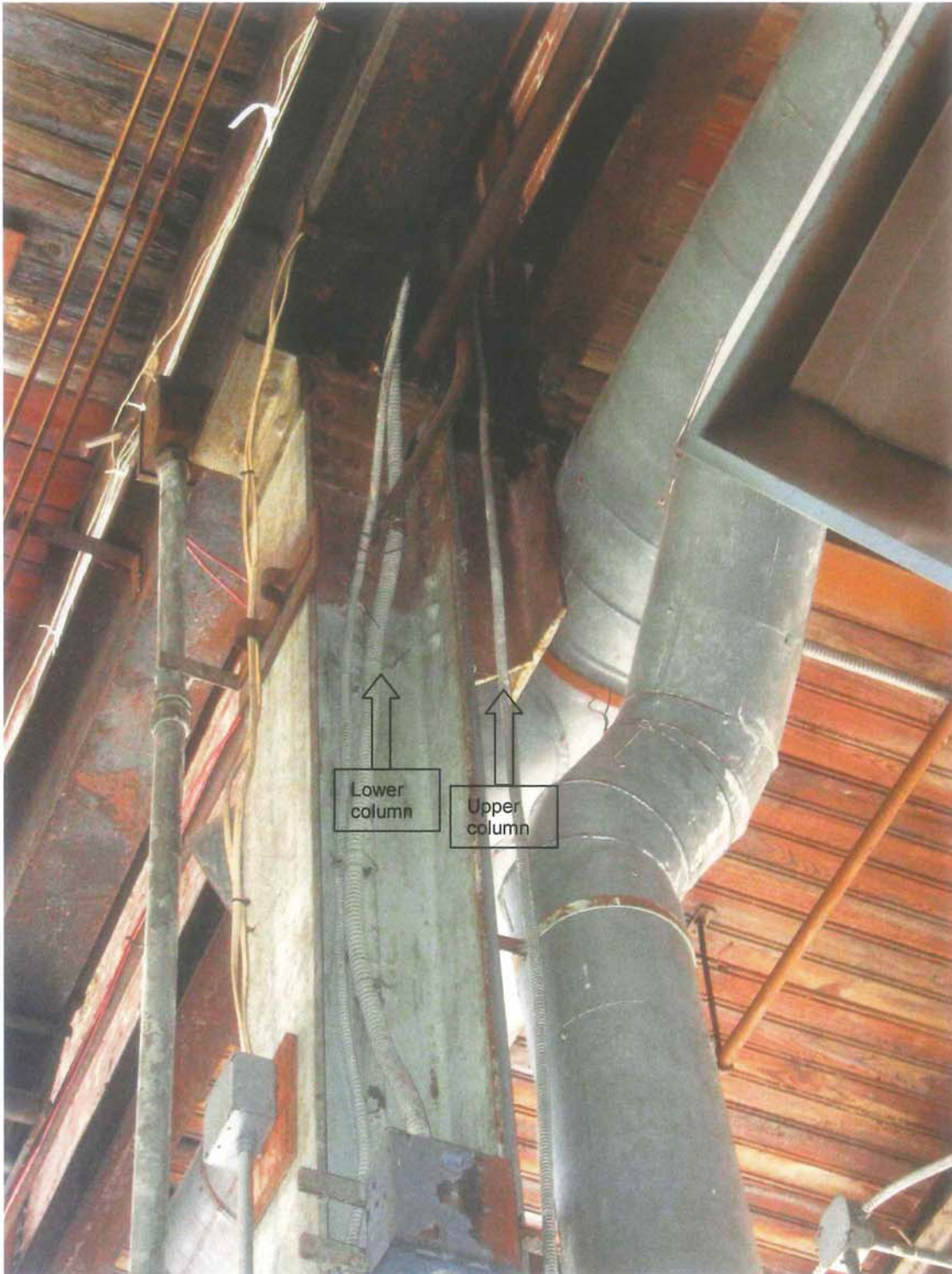
Photo 1-5: Column discontinuity at low-high roof condition.
