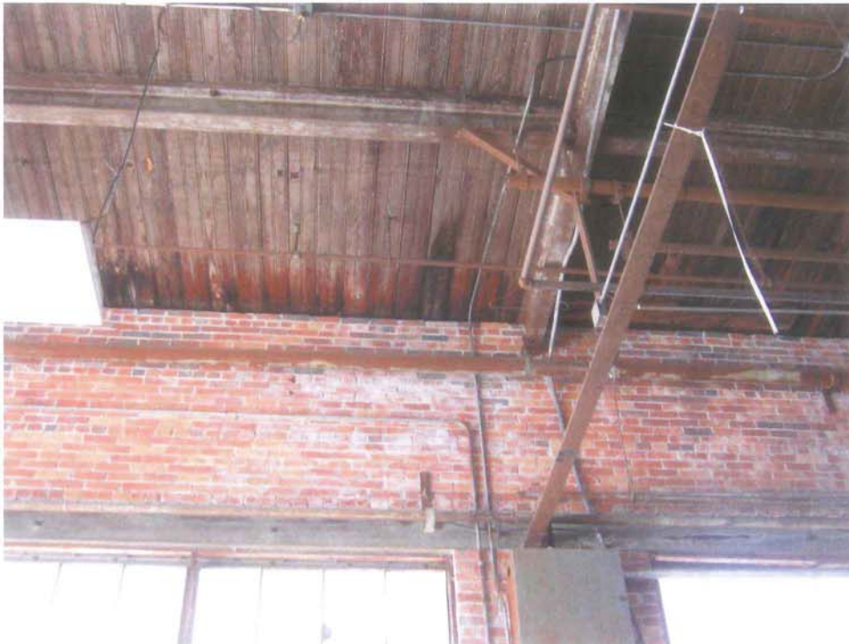
Photo 1-2: Wood deck condition at eave.
