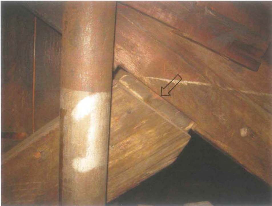
Photo 2-5: Timber truss joint separation.
