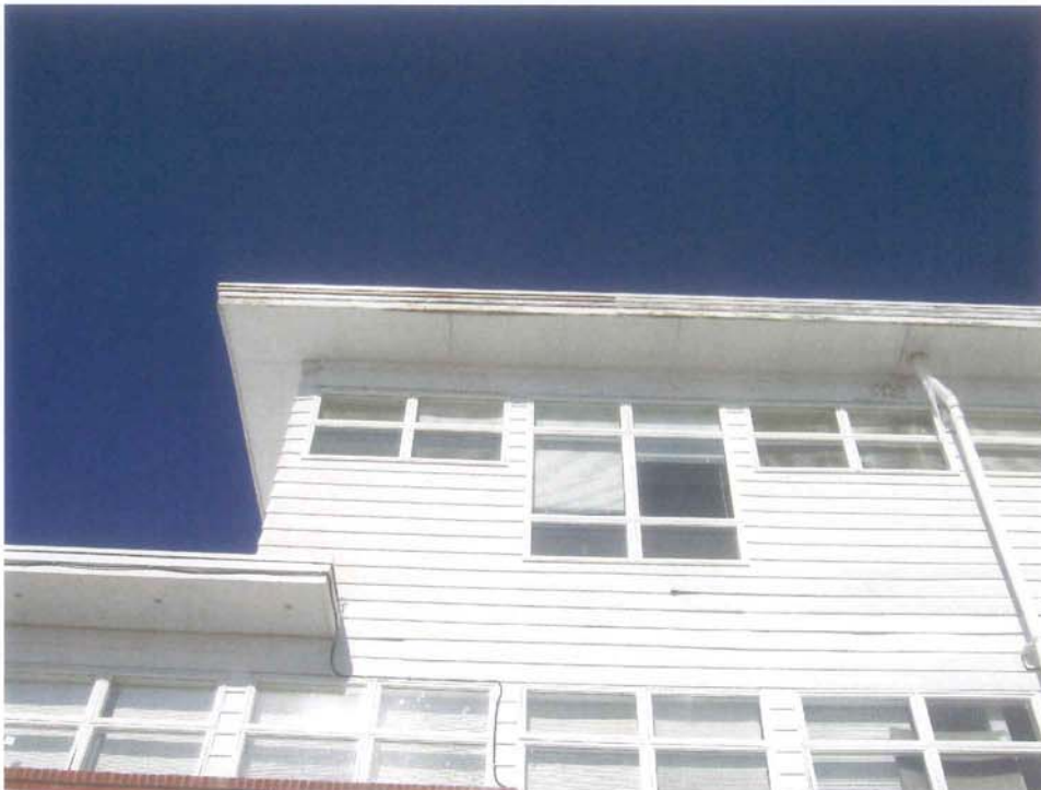
Photo 30-2: Peeling paint at roof eave, uneven siding.
