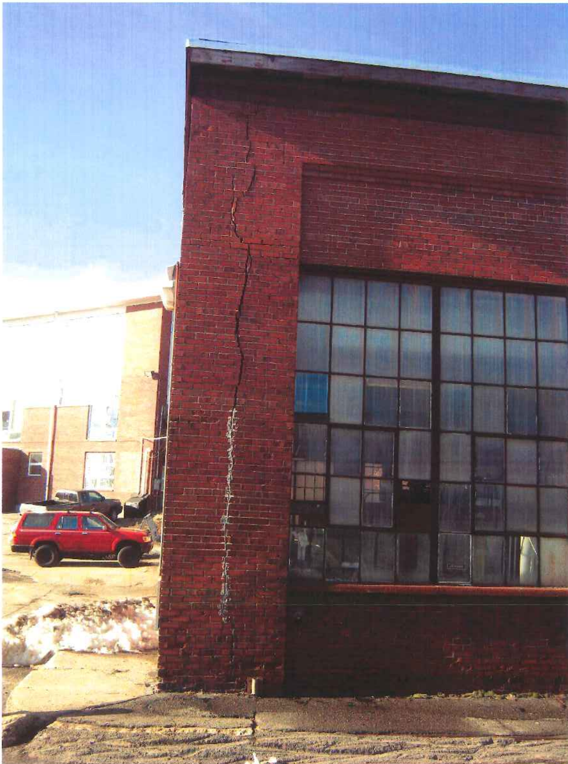
Photo 1-4: Vertical brick masonry crack at southwest pilaster.
