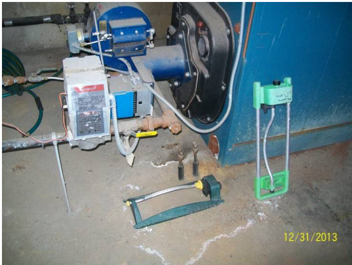
13. Image showing area surrounding new natural gas boiler in boiler room located in southeast corner of Site building.
