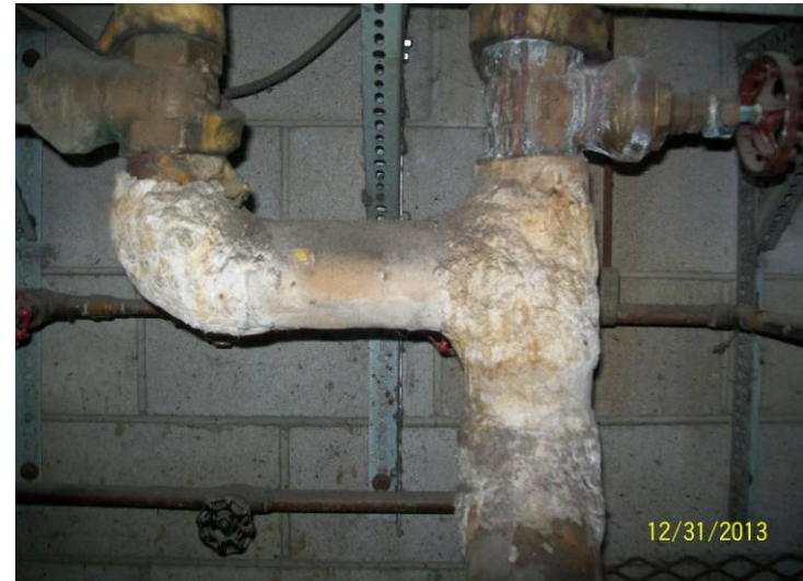
14. Image showing boiler piping in boiler room located in southeast corner of the Site building.
