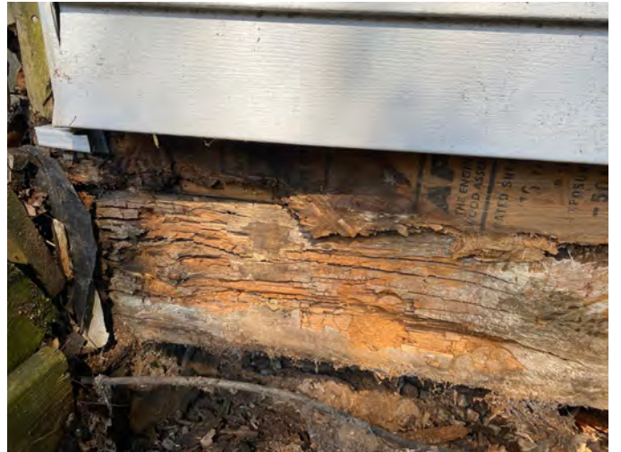
MORE SILL ROT
