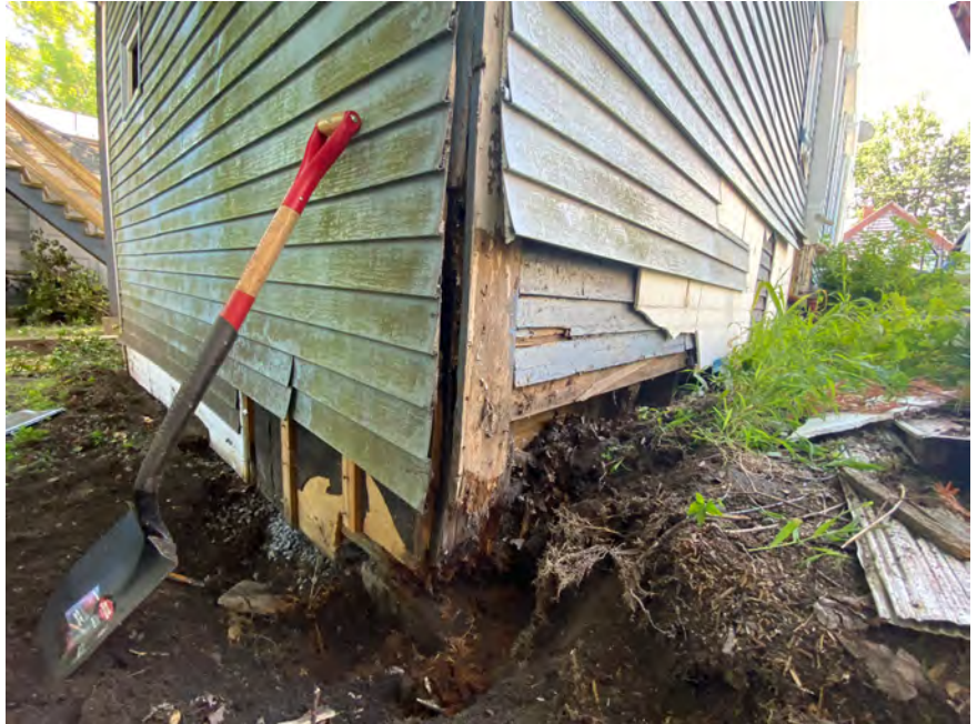
REAR ADDITION ROT
