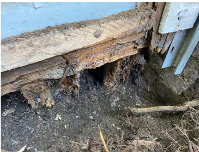
ADDITION SOUTH SIDE ROT
