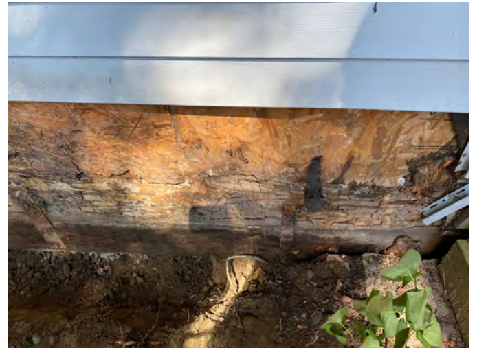
ADDITION EAST SIDE ROT
