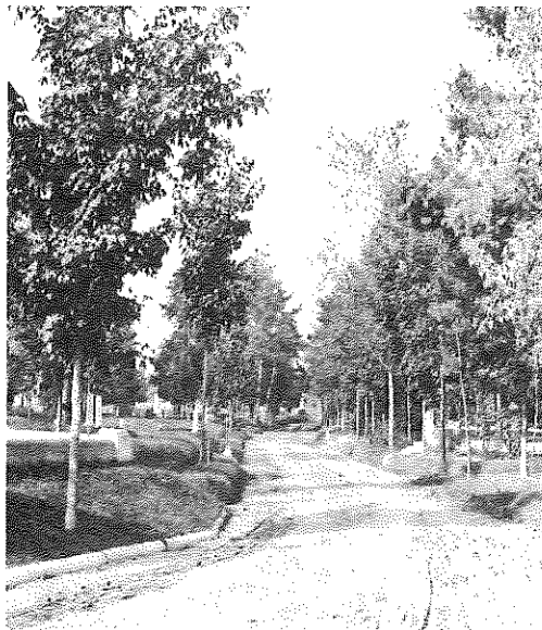
The original cemetery roads were earthen carriage paths. Today, the deteriorated road condition severely impacts the overall landscape character.
