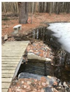
Deteriorating Dam for Haverly Way Pond.JPG 4337K
