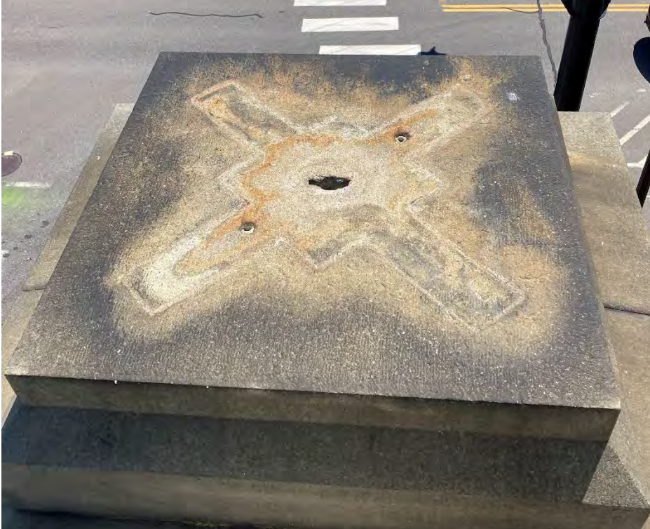
Figure 4: 2022 image of the top of the west pier showing the ghost of the original light fixture. (Parks, Recreation, & Facilities Staff)
