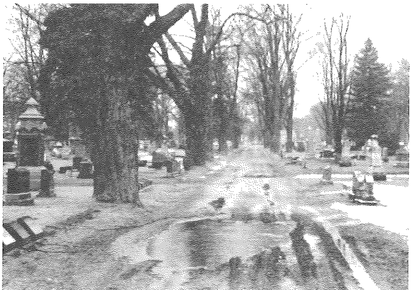
Deferred maintenance of the cemetery's roads has contributed to a condition in which the majority of the site's roads are in fair to poor condition. There is a lack of adequate road construction in the form of crowns and swales.
