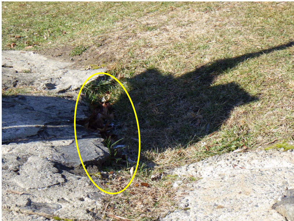
Photo 24: Sinkhole adjacent to left abutment training wall (in shaded portion of photograph)
