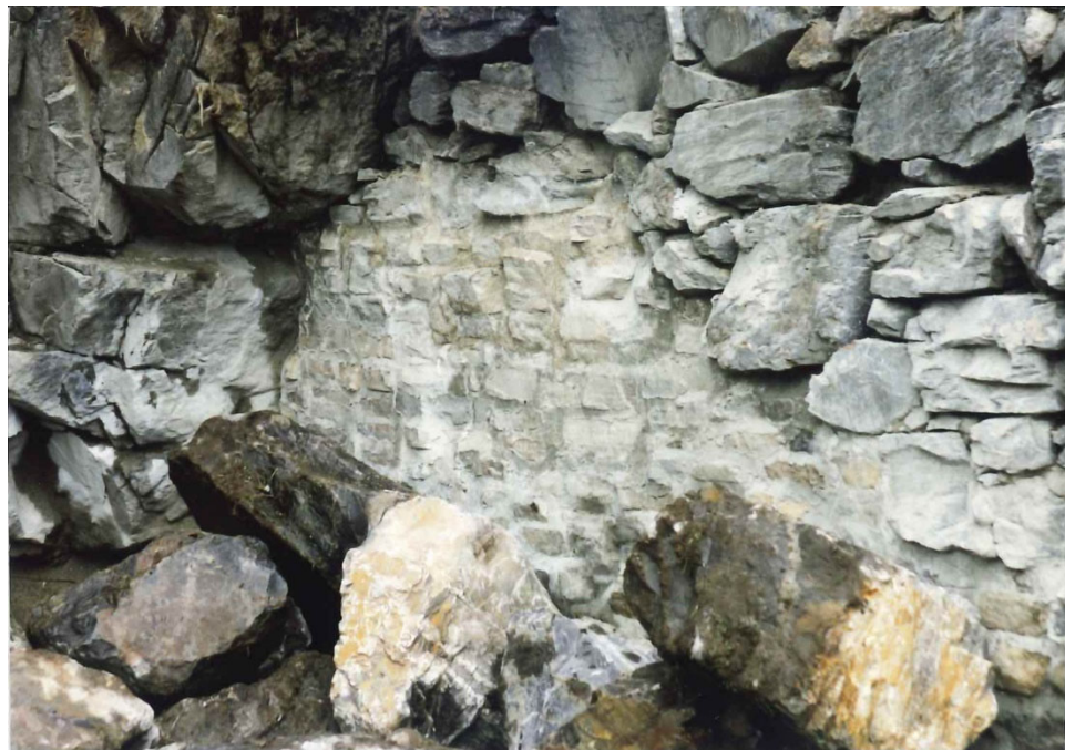
[Historic] Photo 46: 1998 repair of partial failure of downstream face at current site of void (detail of contact with right bedrock abutment)
