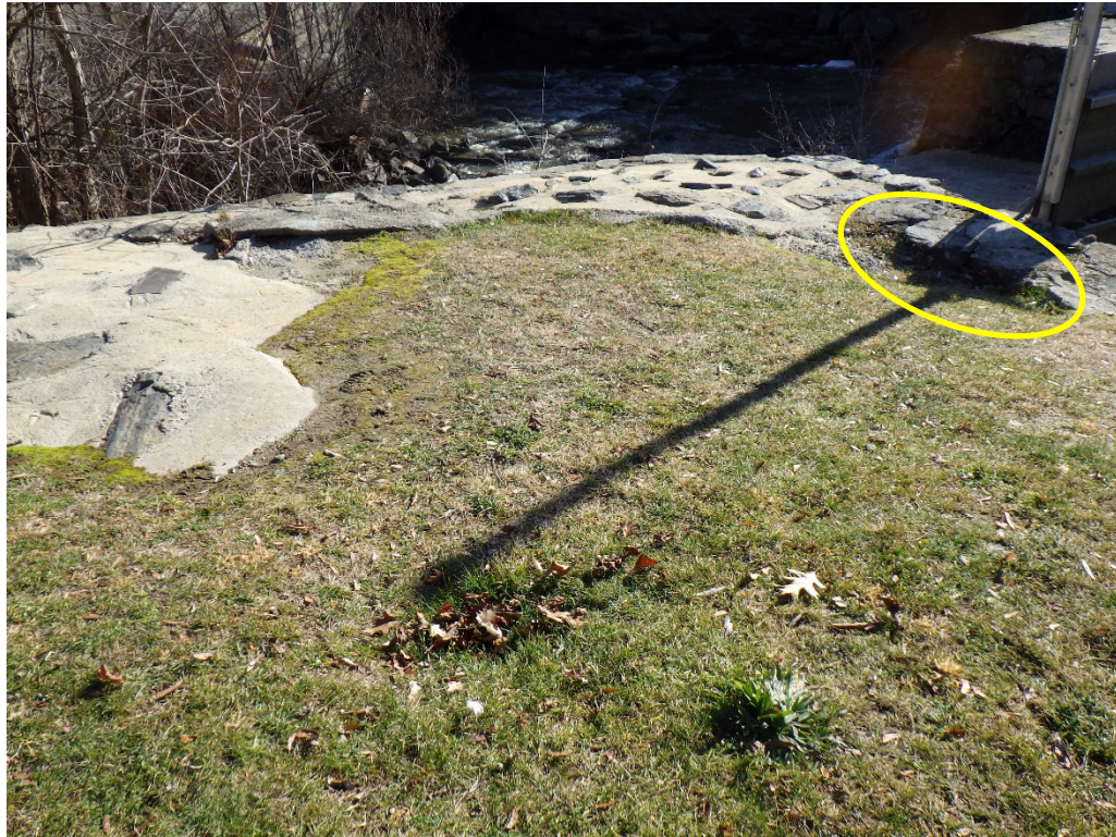
Photo 21: Localized sinkholes across Left Abutment
