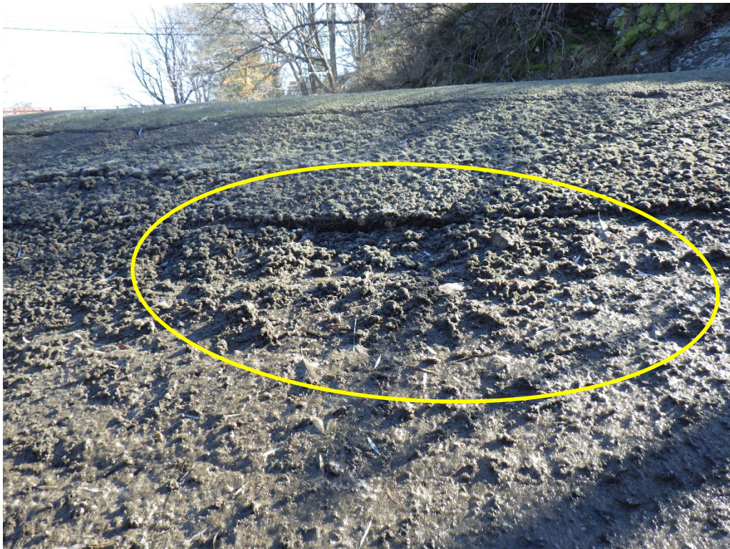
Photo 8: Depressed area of upstream face of Primary Spillway (similar condition as in 2012)
