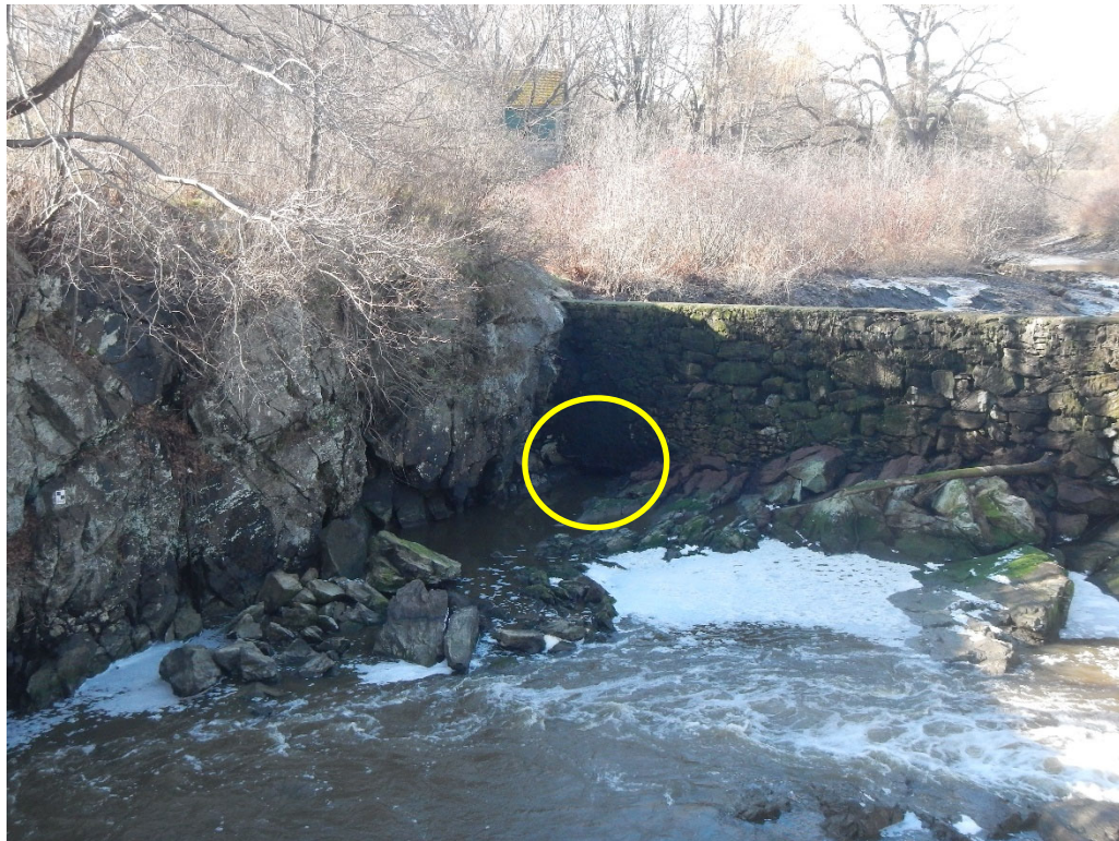
Photo 43: Interface between downstream face and right bedrock abutment (NOTE void at toe of downstream face at contact with abutment)
