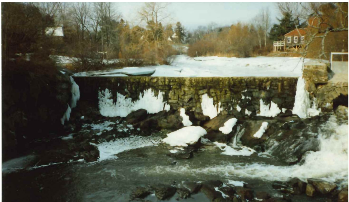
[Historic] Photo 4: Leakage areas through dam on February 17, 1999 (delineated by ice formations)
