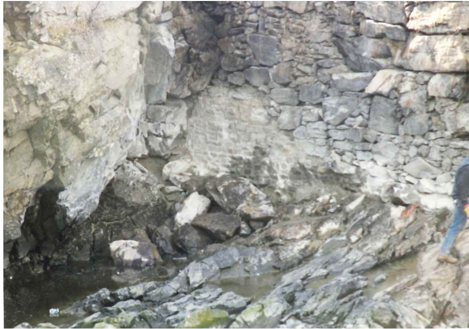
[Historic] Photo 45: 1998 repair of partial failure of downstream face at current site of void
