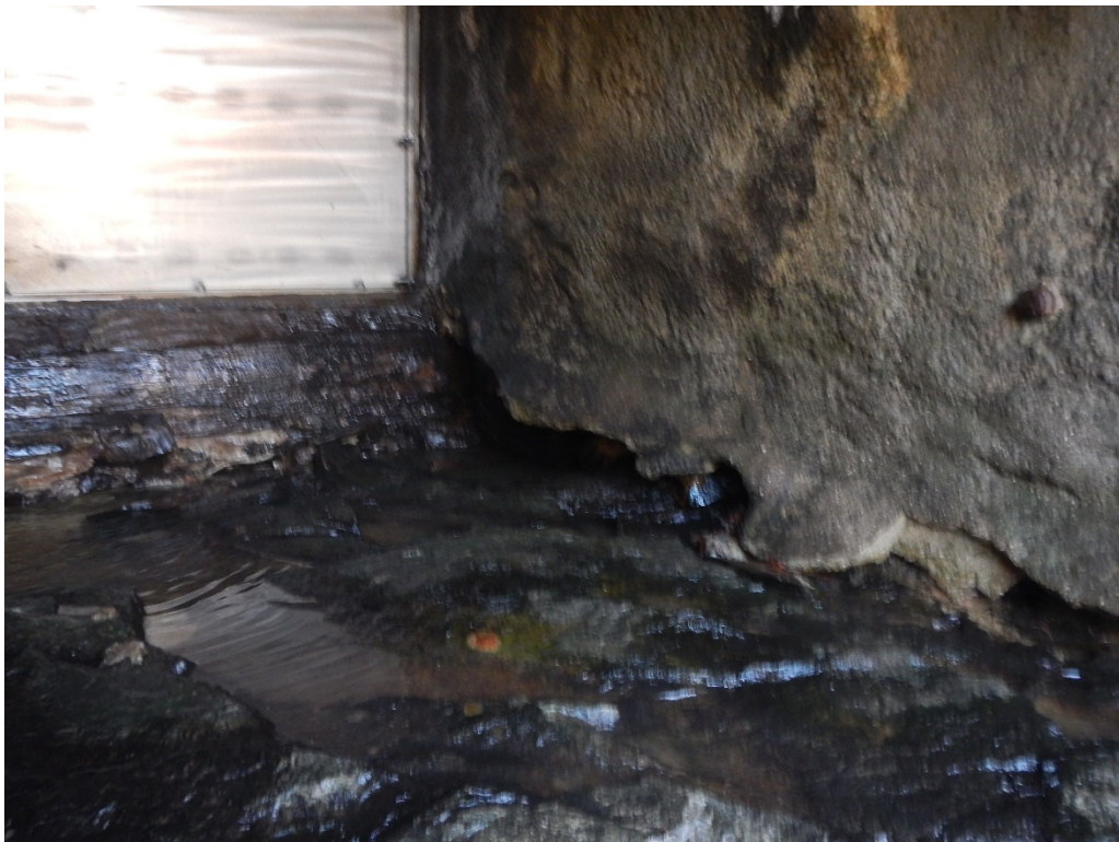
Photo 32: Interface between bedrock foundation and shotcrete overlay on left side of Sluiceway
