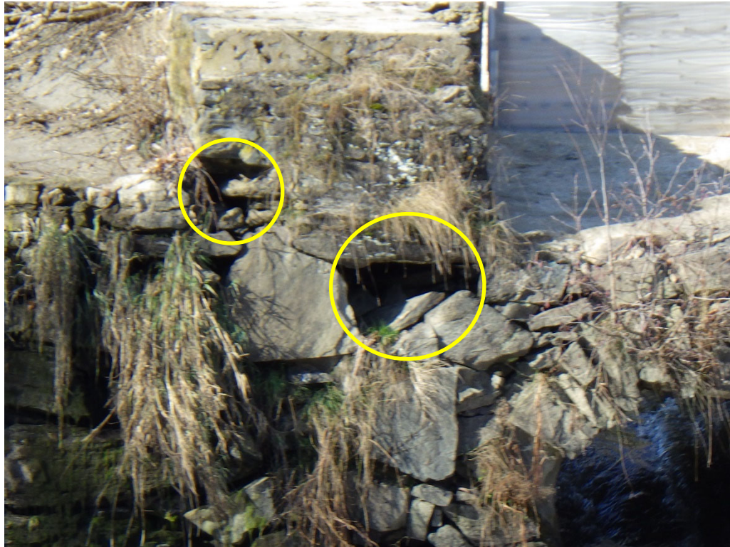
Photo 37: Stone loss and vegetation on downstream face of divider pier
