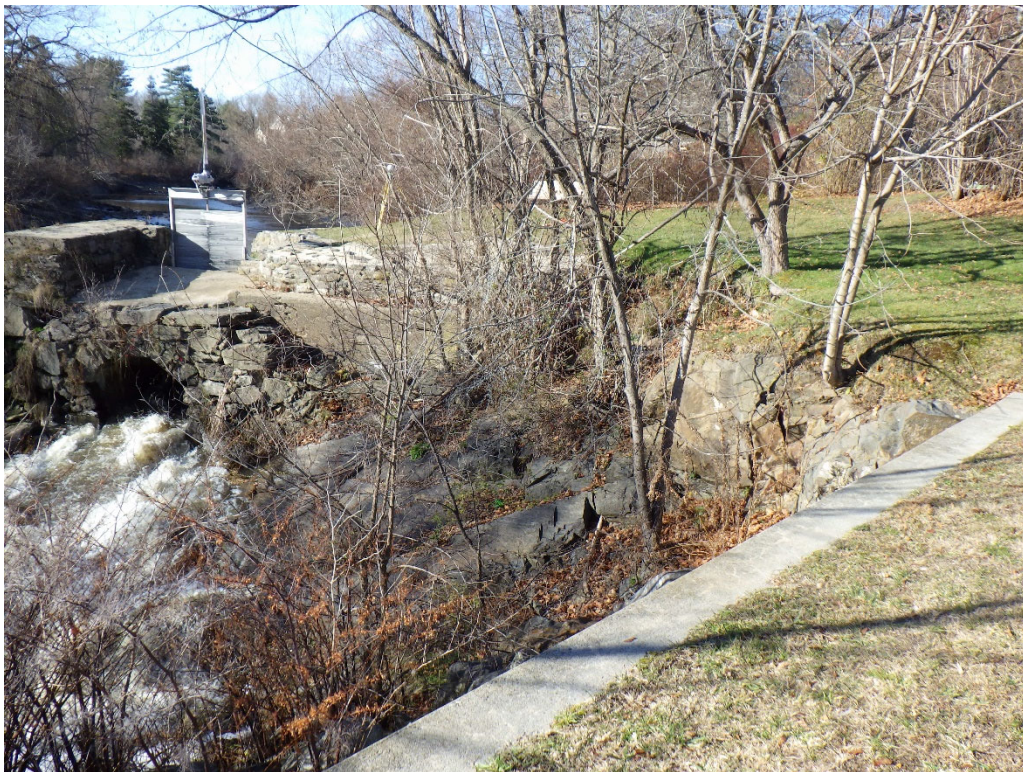
Photo 26: Tree growth on downstream side of Left Abutment
