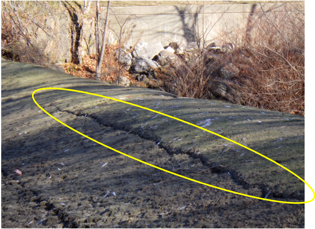
Photo 9: Upper concrete overlay crack and crest deformation on Primary Spillway
