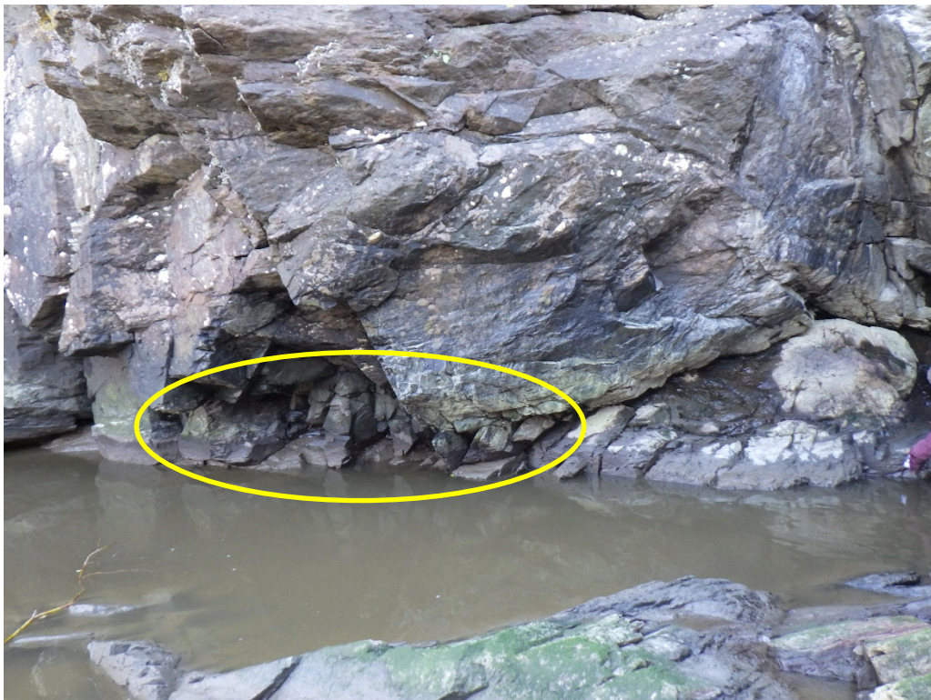
Photo 50: Spalling along toe of right bedrock abutment, downstream of dam
