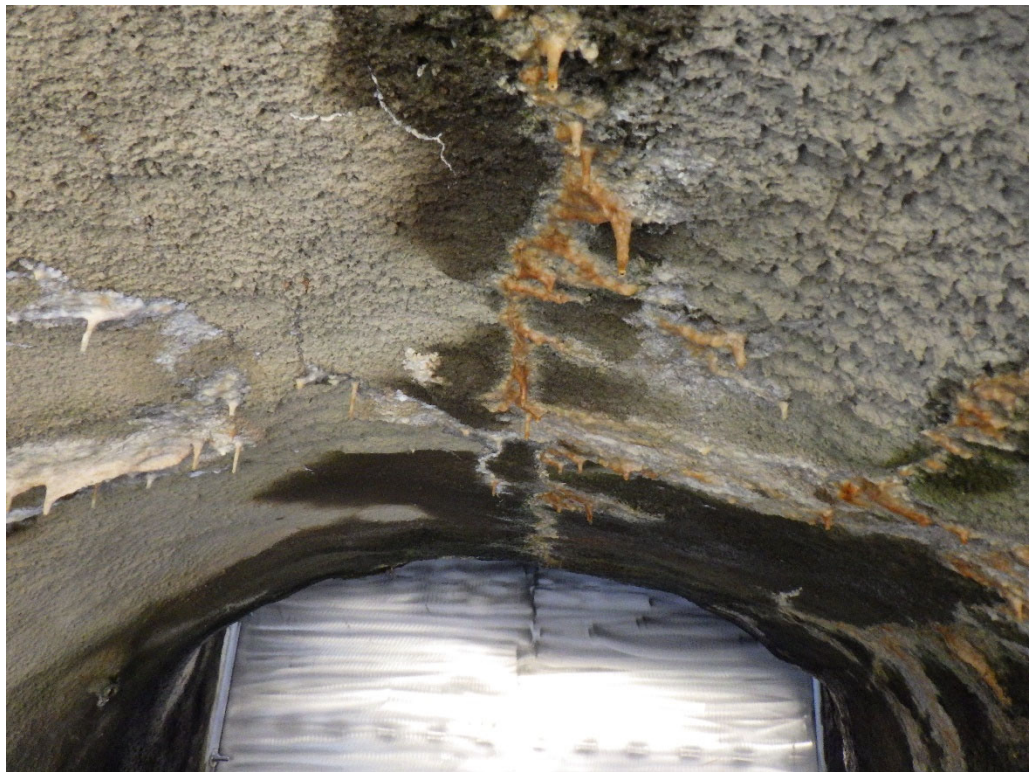
Photo 30: Condition of shotcrete overlay of Sluiceway ceiling
