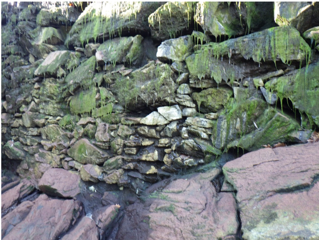
Photo 40: Sporadic stone movement and vegetation along downstream face of Primary Spillway
