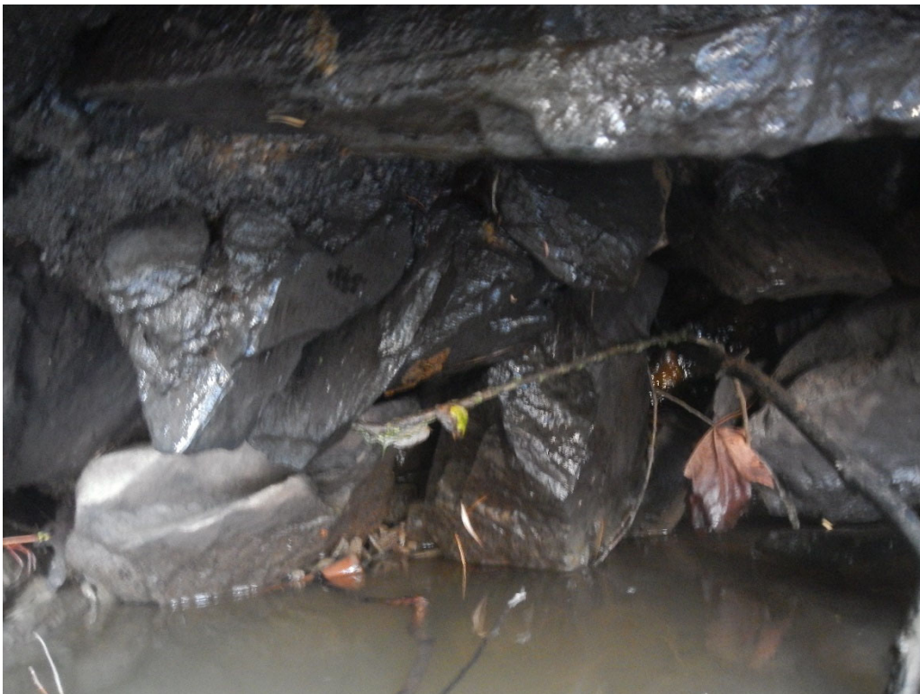
Photo 48: Detailed photo of right side of void
