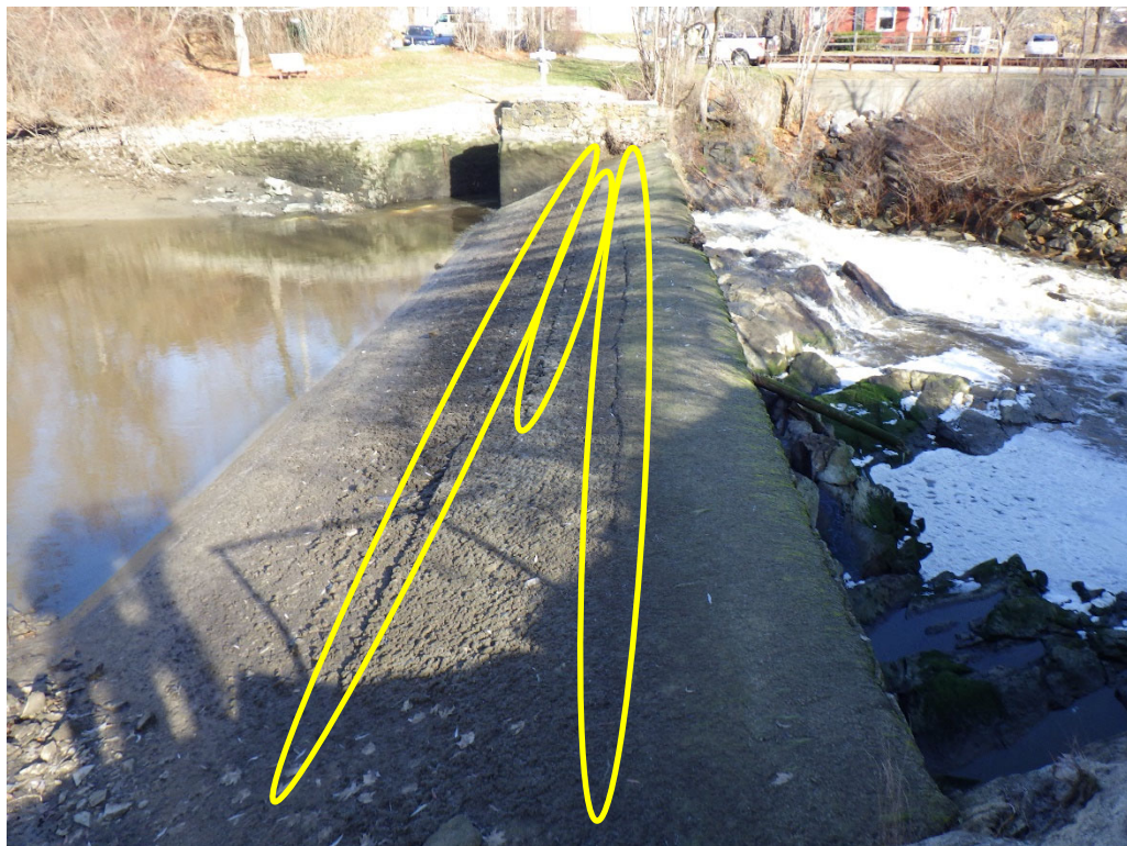
Photo 6: Primary Spillway concrete condition (NOTE longitudinal cracks)
