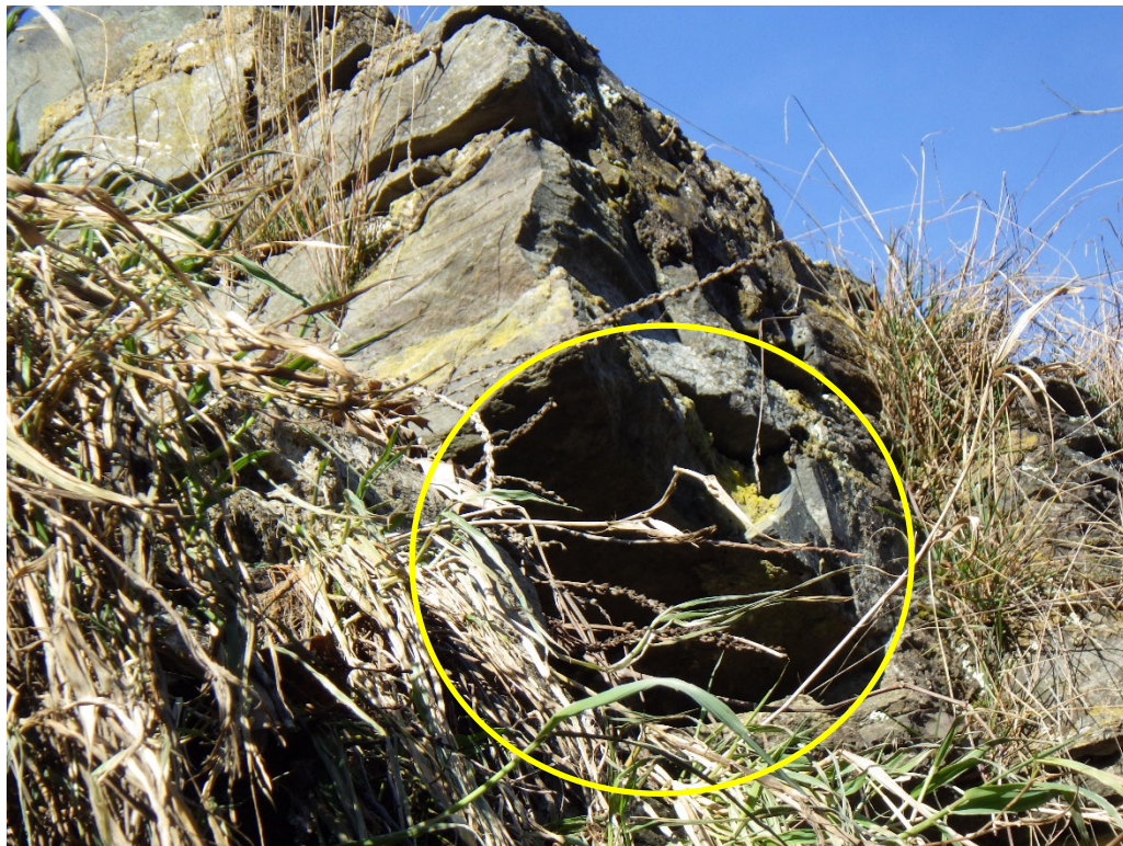
Photo 38: Stone loss along downstream face of divider pier
