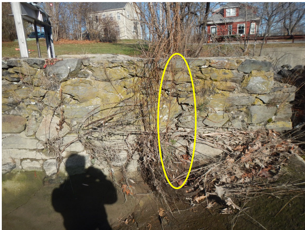
Photo 12: Divider pier cracking and vegetation growth (potential leakage source)
