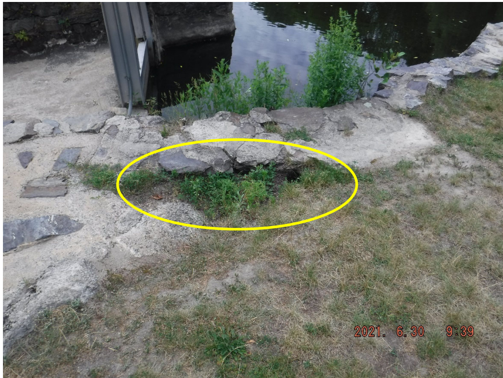
[Historic] Photo 23: Left Abutment sinkhole on 6/30/2021
