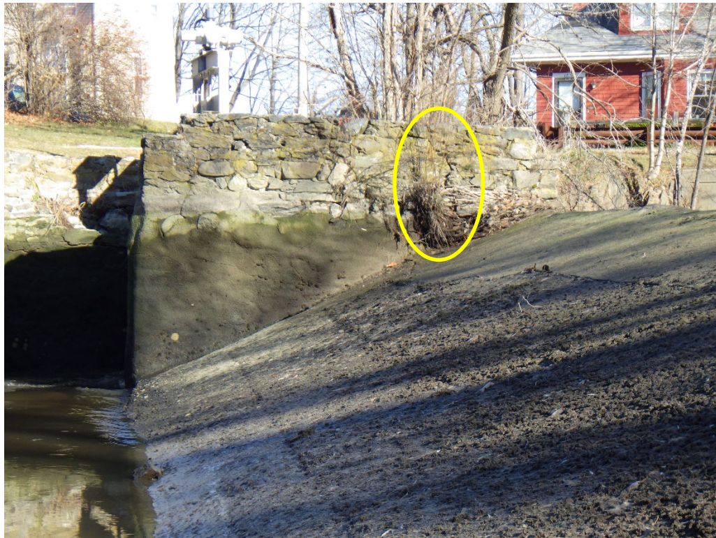
Photo 11: Divider pier with cracking and vegetation growth (potential leakage source)
