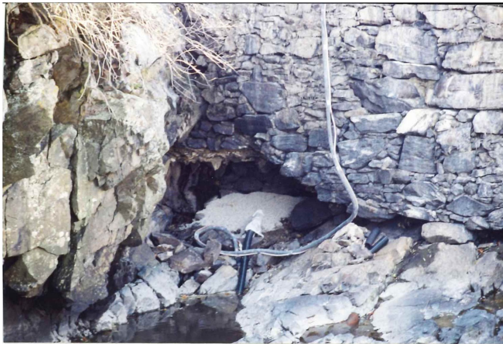
[Historic] Photo 44: 1998 partial failure of downstream face at current site of void
