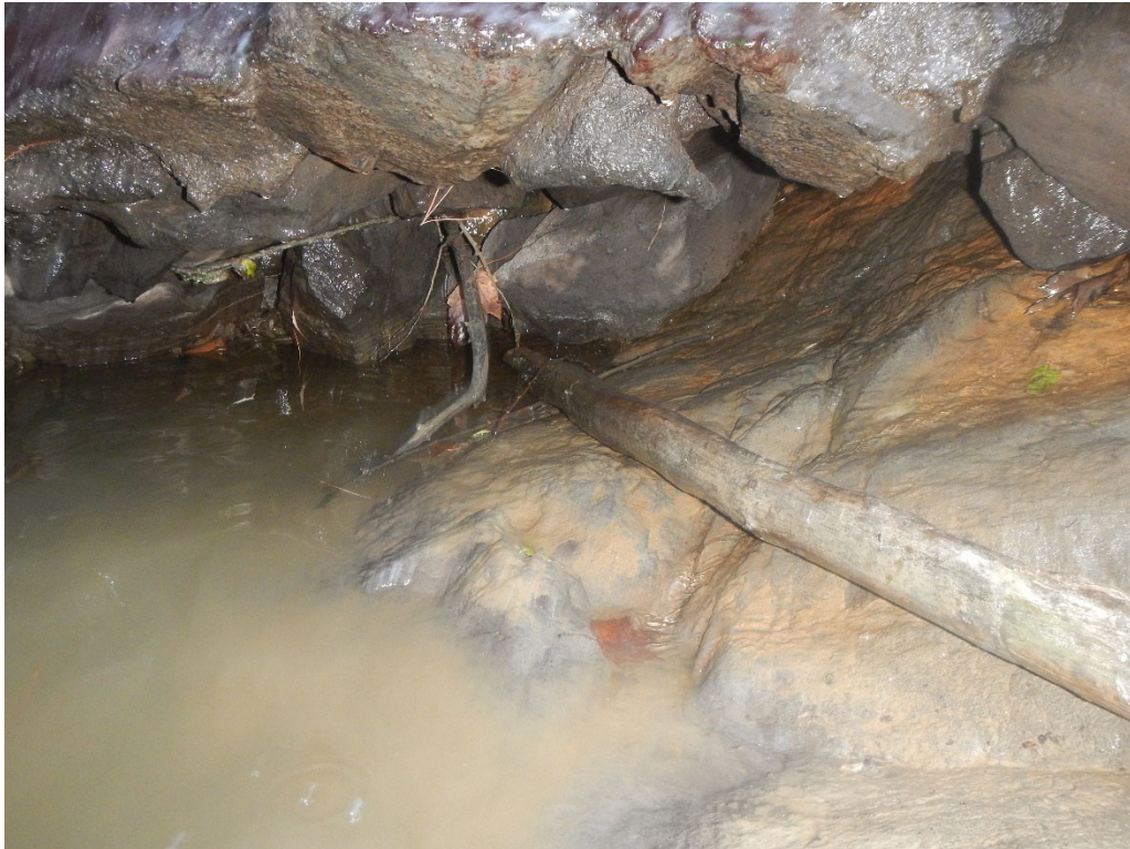
Photo 49: Detailed photo of left side of void
