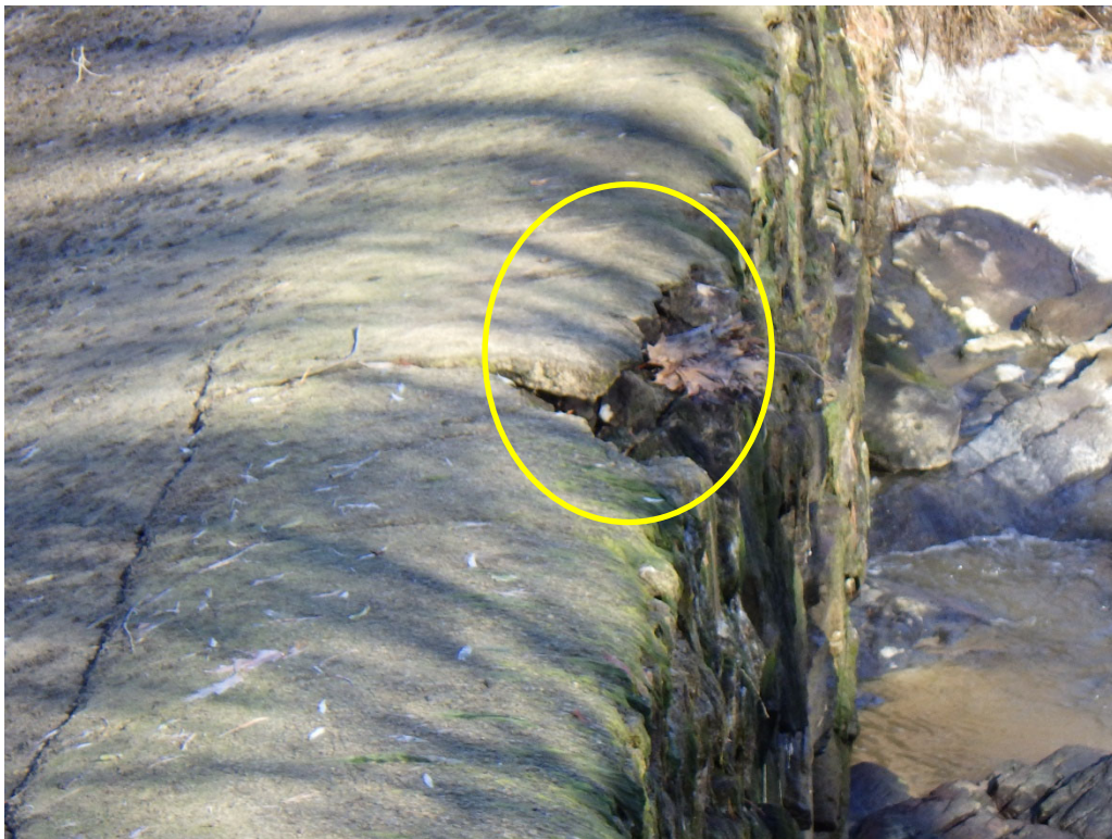
Photo 10: Damaged portion of spillway crest near center of Primary Spillway
