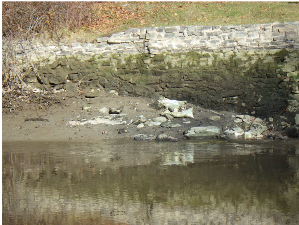
Photo 18: Upstream end of left abutment training wall with sediment accumulation
