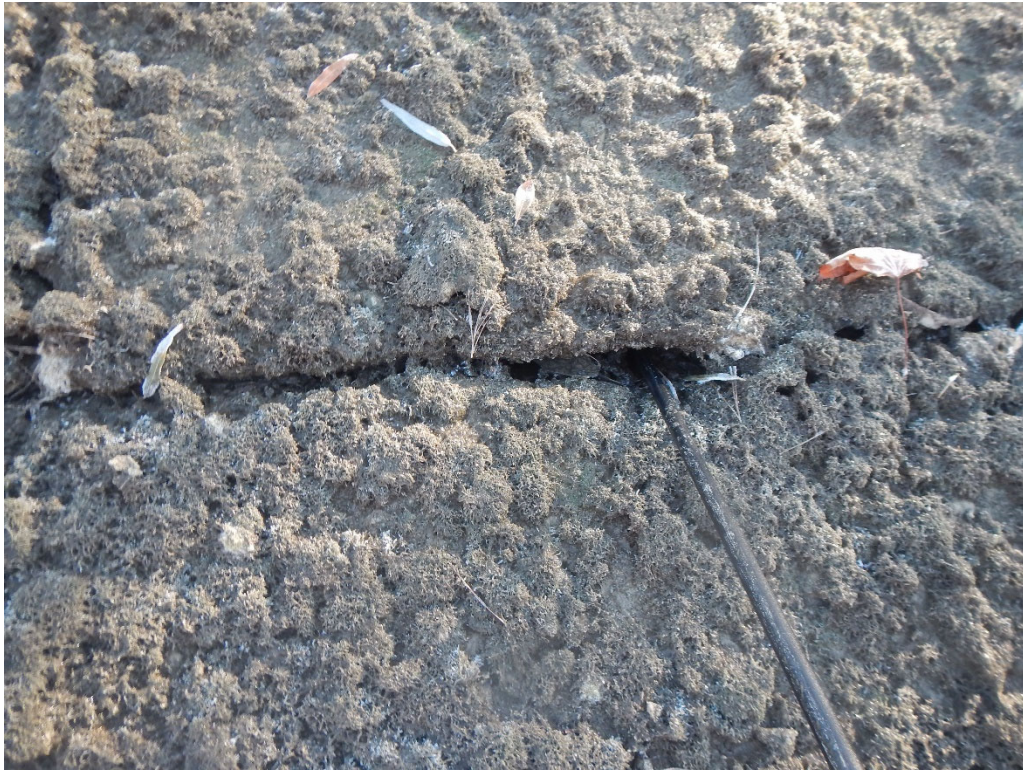
Photo 7: Deepest penetration (six inches) of longitudinal crack in Primary Spillway
