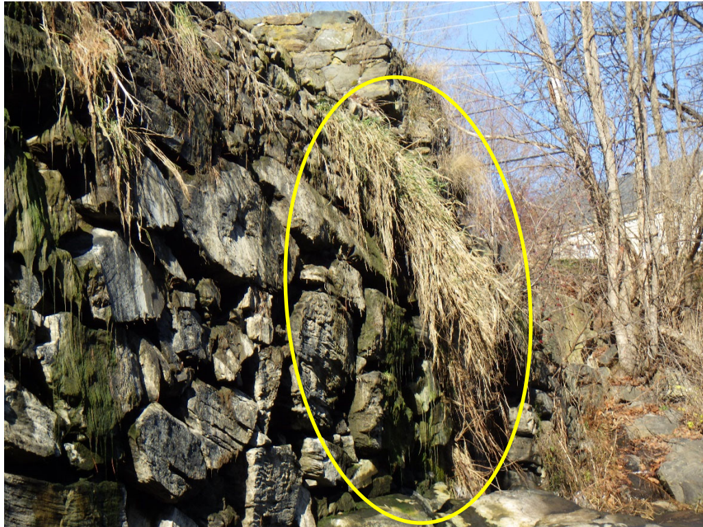
Photo 41: Bulged area of downstream face, near left contact of Primary Spillway and Divider Pier
