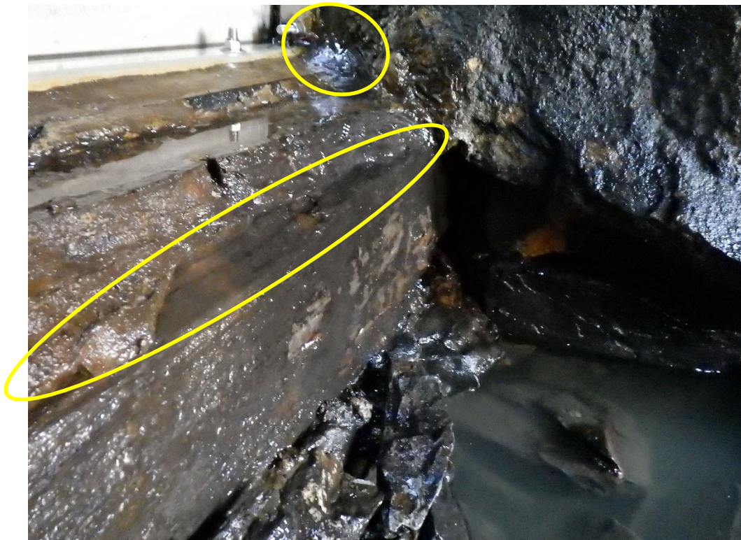
Photo 34: Interface between sill of Slide Gate, bedrock foundation, and shotcrete overlay of Sluiceway
