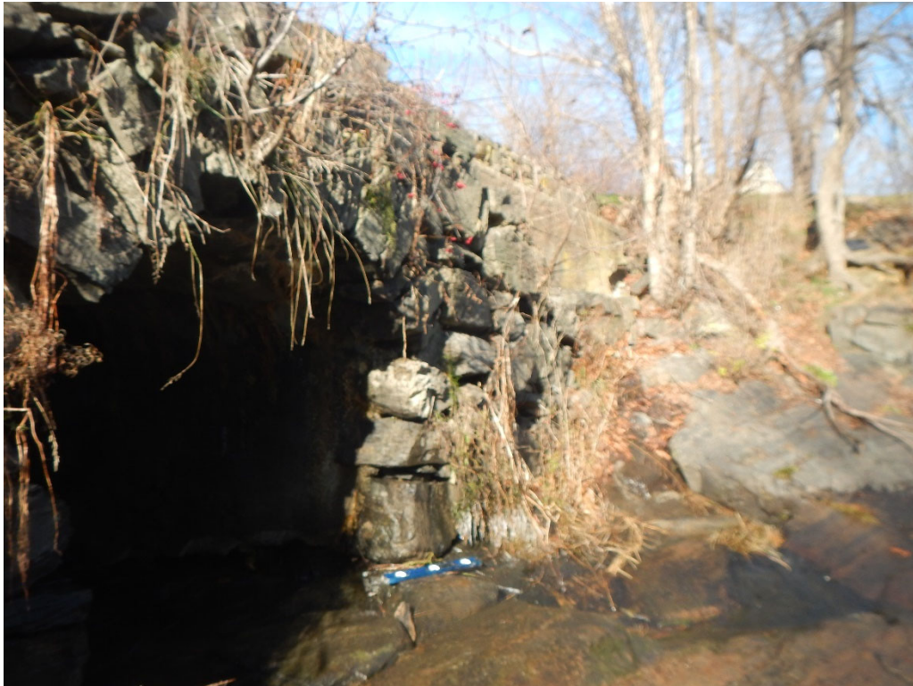
Photo 27: Tree growth and vegetation near Sluiceway outlet and downstream face of Left Abutment
