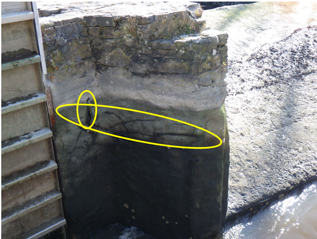
Photo 14: Condition of upstream face of divider pier; NOTE cracks in shotcrete overlay
