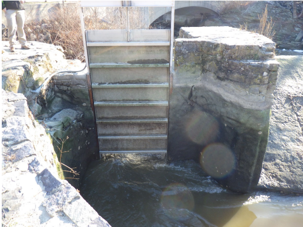
Photo 15: Aluminum Slide Gate (left side of dam) that controls discharge to Low-level Outlet
