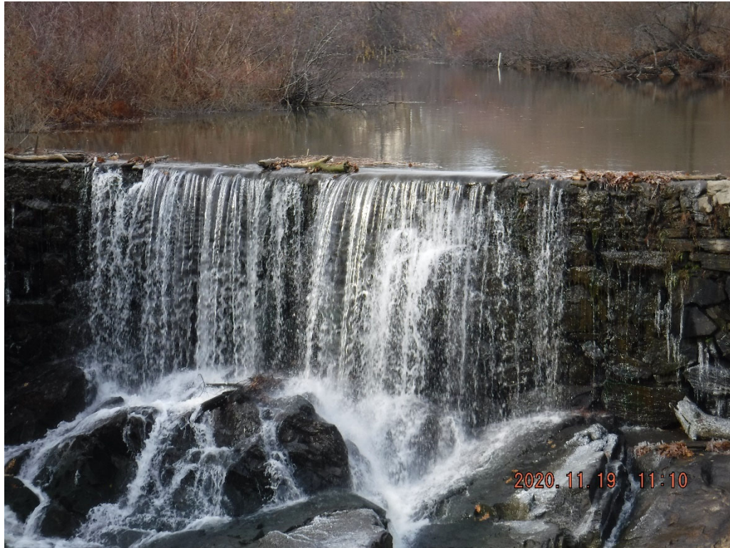
[Historic] Photo 5: Uneven spillway crest and spillage on November 19, 2020 (NOTE center discharge only)
