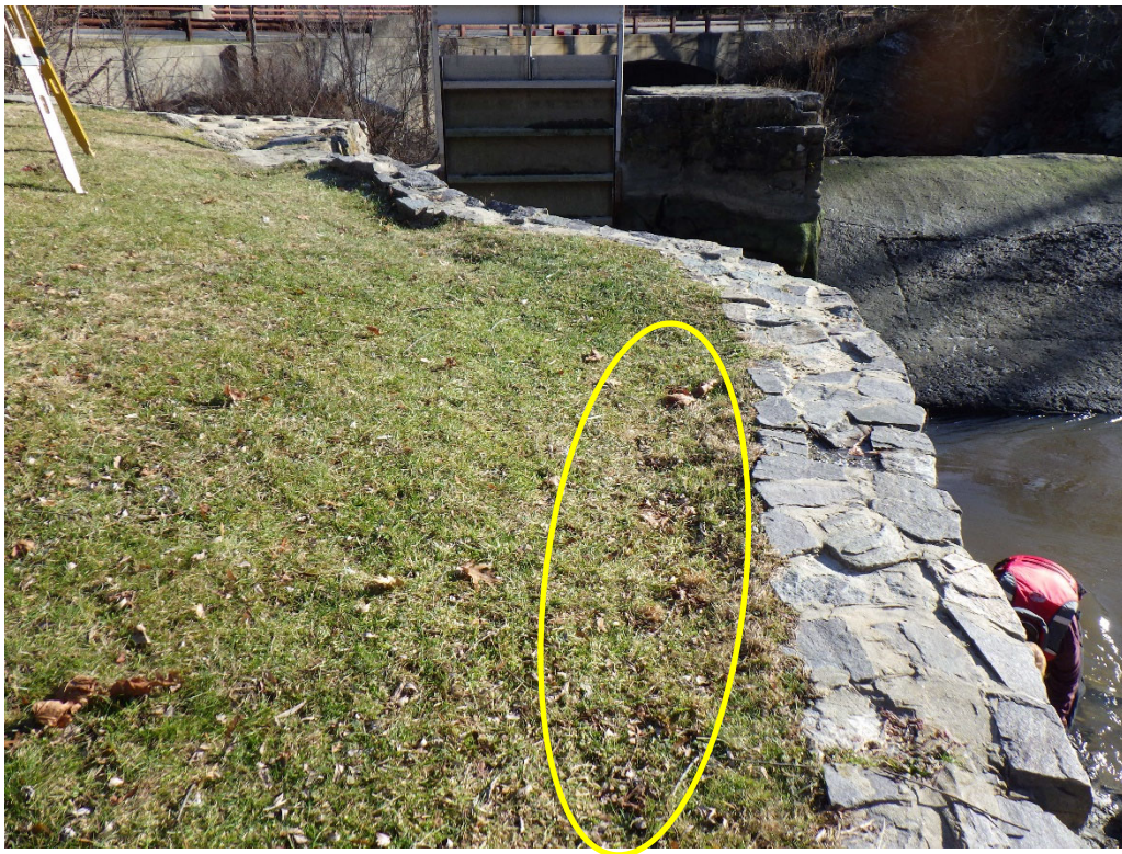
Photo 20: Depressed surface behind left abutment training wall
