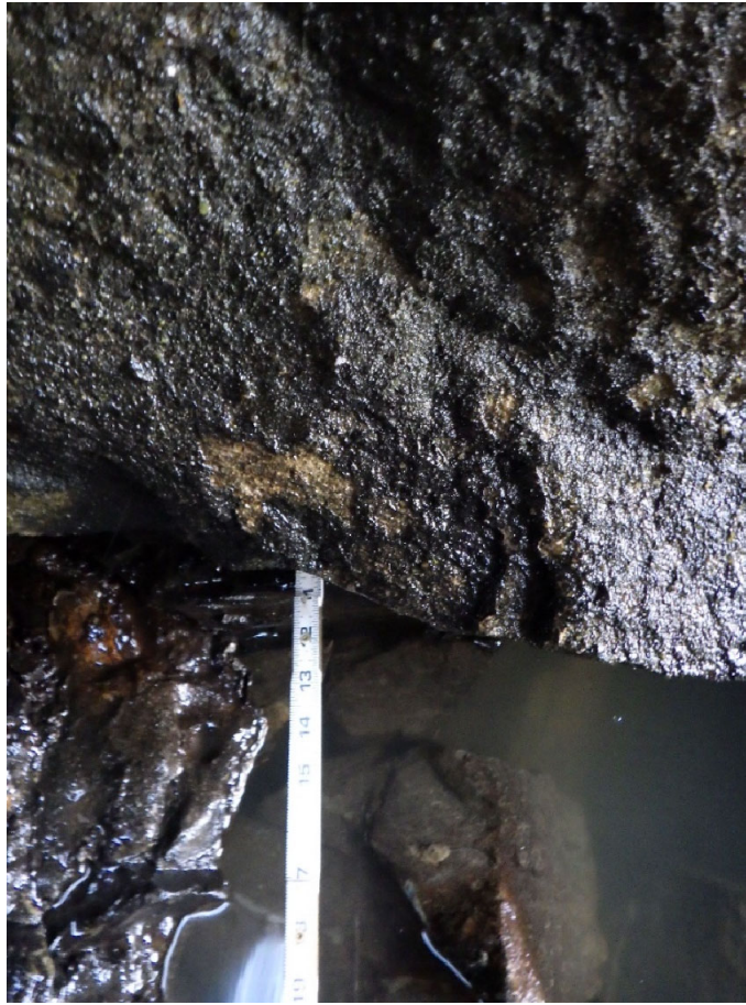
Photo 35: Depth of void along left side of Sluiceway
