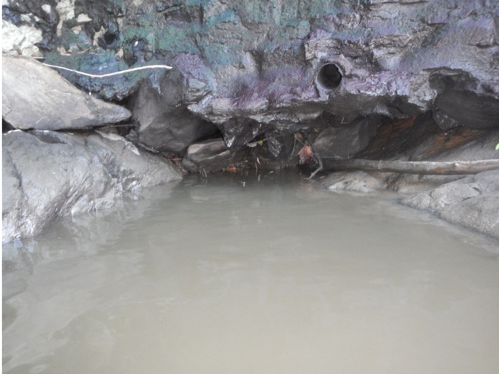
Photo 47: Void at interface of downstream face, right bedrock abutment, and bedrock foundation
