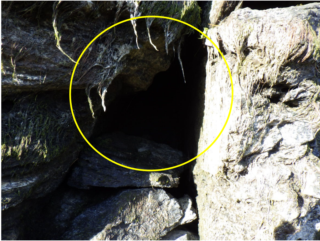
Photo 39: Stone loss near downstream face of divider pier
