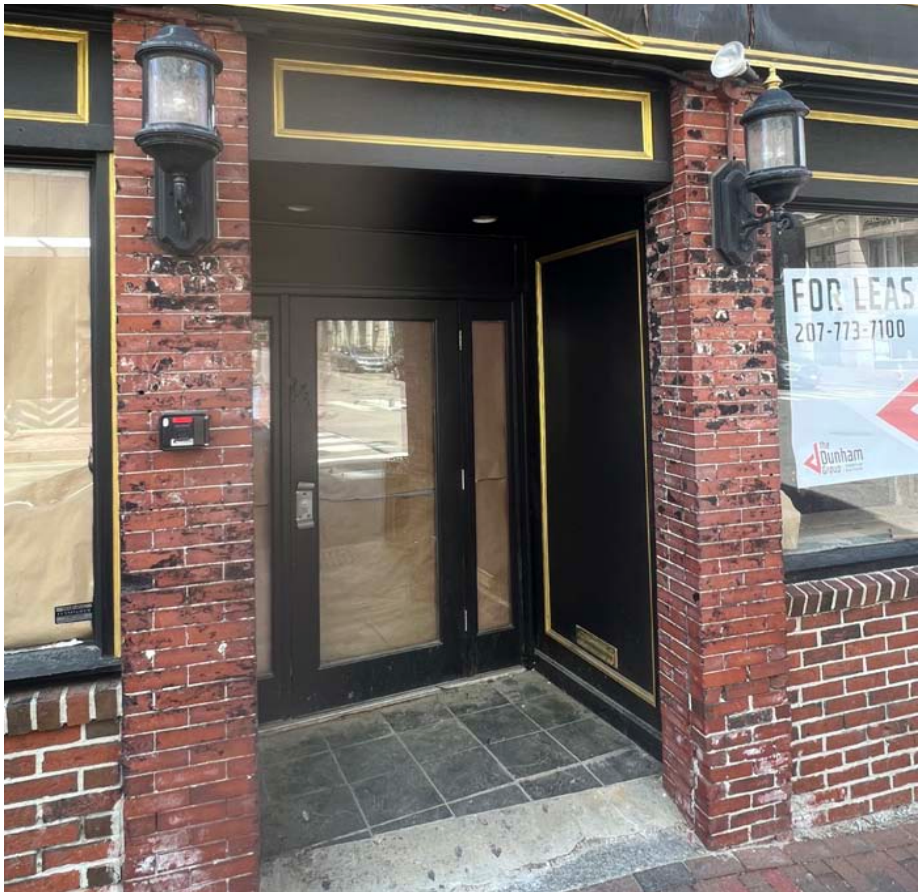
Photo 8 Primary Front Entry Recessed entry of 1st floor commercial space. Entry doors to be brought out to the street plane as from the historic pattern of the building. The existing tile floor pitches into the building, causing water and deterioration problems. Before Rehab. Fall 2022
