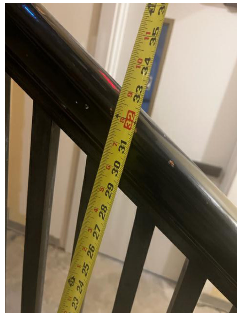
EXISTING GUARDRAIL ON STAIR 1C
