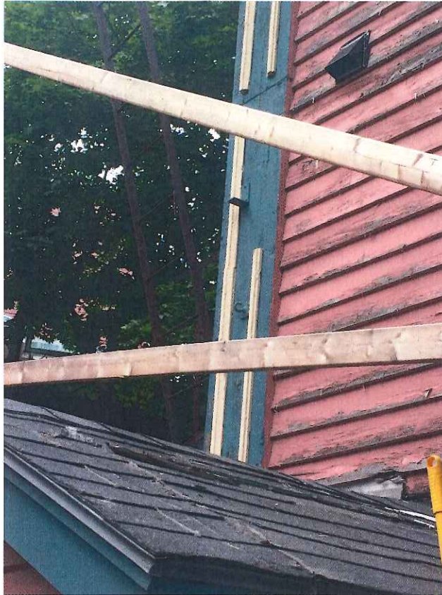
Detail (above) reveals missing cornerboard trim and paint ghost mark showing where back porch roof once existed.
