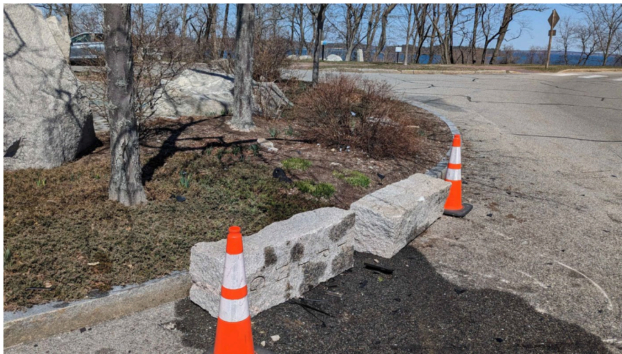
Figure 5: Granite sentinel post damage adjacent to Eastern Promenade roadway
