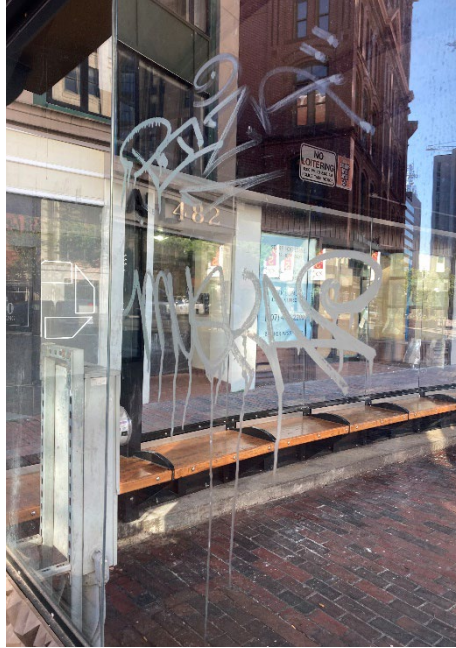
Figure 1: Glass Panels damaged by graffiti
