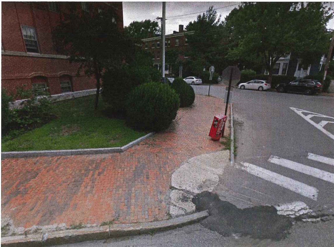
Photo 6: Concrete ramps to be removed and upgraded to brick curb ramps with cast iron detectable warning panels. Granite curbing to remain at back of sidewalk. Shrubs blocking view of monument to be removed. Additional plantings to be proposed in area behind monument.
