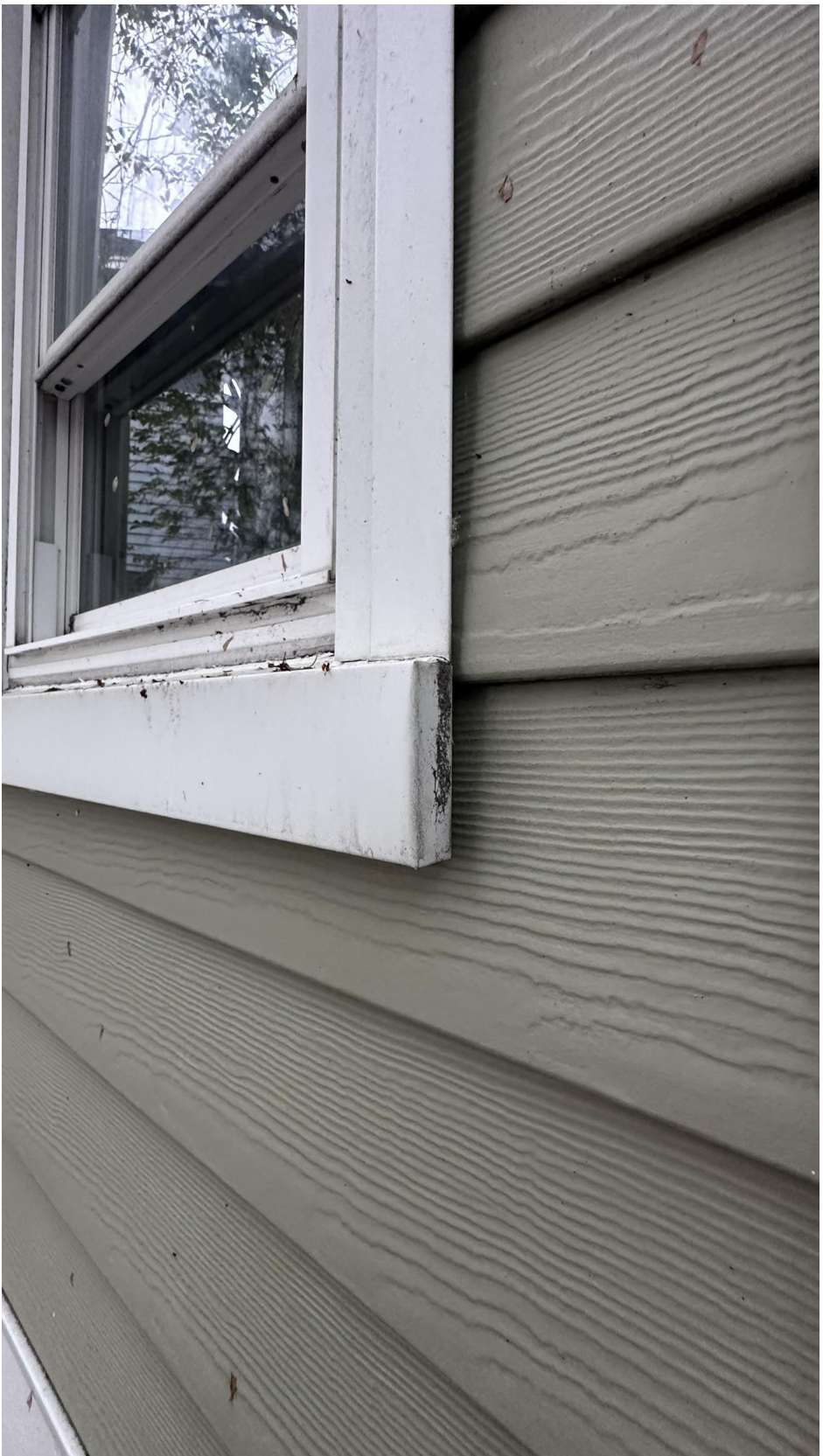
ALL ORIGINAL WINDOW TRIM HAS BEEN REMOVED. TYP. TRIM PHOTO.
