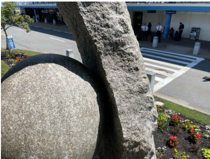
Photo of area above ball at approximately 96 inches. It is possible that the right hand column in the photo has hairline cracks in this area.
