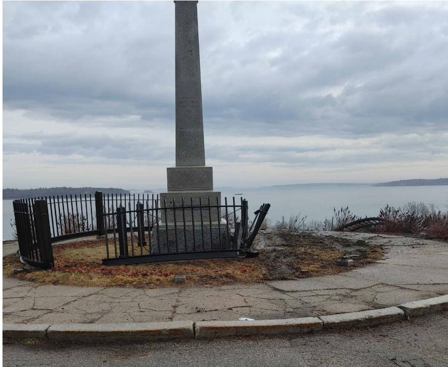
Figure 6: Metal fencing damaged by car
