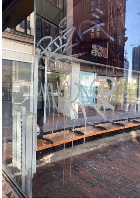
Figure 1: Glass Panels damaged by graffiti
