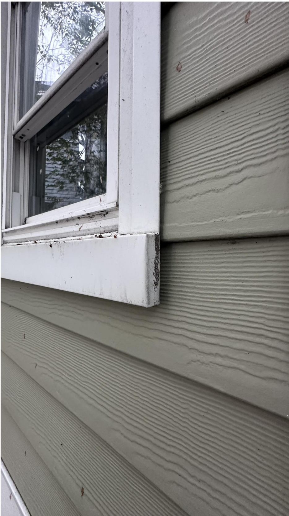
ALL ORIGINAL WINDOW TRIM HAS BEEN REMOVED. TYP. TRIM PHOTO.
