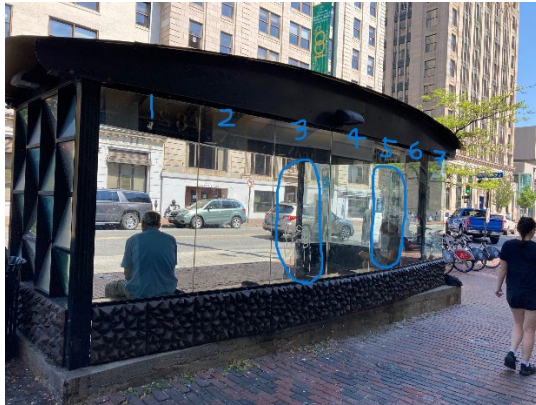
Figure 1: Glass Panels damaged by graffiti
