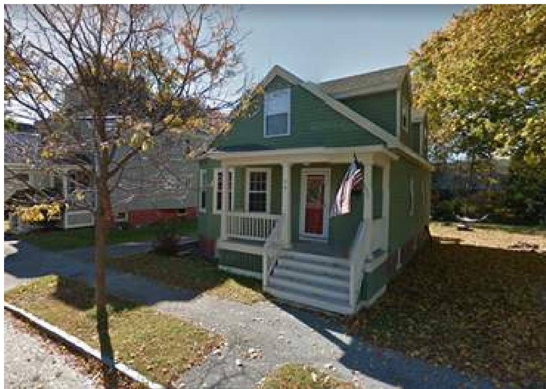
EXAMPLE OF TYPICAL PORCH CONDITIONS ILLSLEY STREET
