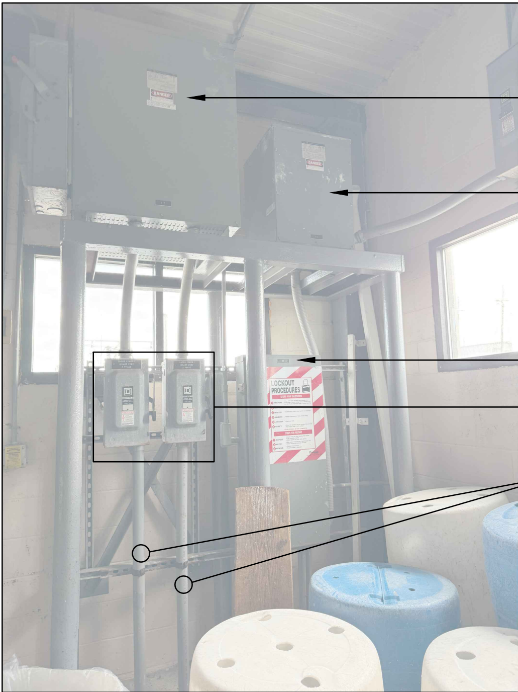
75 KVA STEP-DOWN TRANSFORMER T2 480V-208/120V, 3-PHASE 37.5 KVA STEP-DOWN TRANSFORMER T1 480V-240V, 1-PHASE
