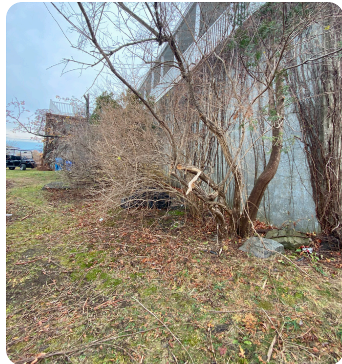
(Below) Mature Lonicera morrowii Shrub Honeysuckle, along the foundation of the home.
