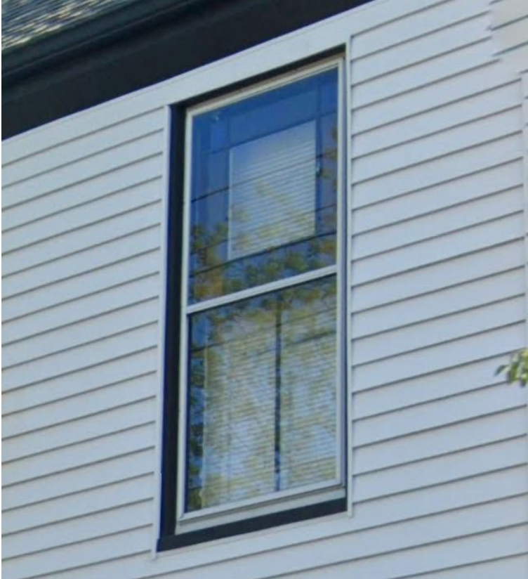
Figure 5: 2019 Google Street View close-up image of the second story window in 2019.
