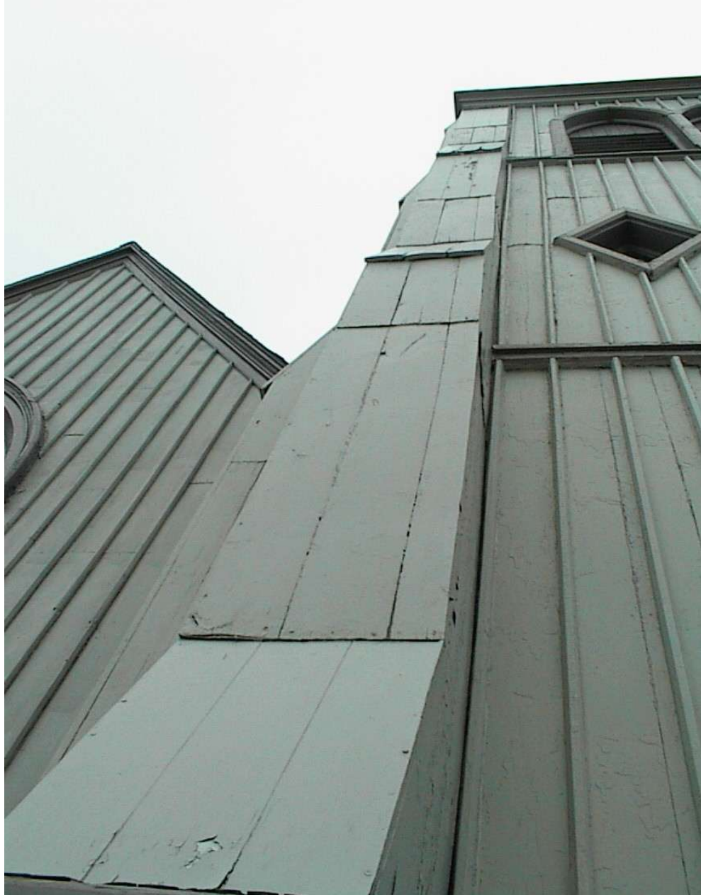
Image Showing Typical Buttress Condition
