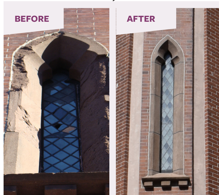
A number of the former church's leaded stained-glass windows were damaged with broken glass and failing leading. Given the distinctiveness of the windows and the amount of remaining glass, it made the most sense to repair rather than replace the windows.
