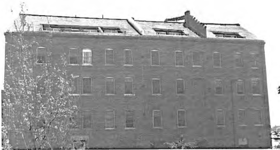
By constructing inverted dormers in this gambrel roof, the developers gained usable space in the former attic. The shape of the roof, a distinctive architectural feature, has been retained and conveys a sense of the building's original character.
