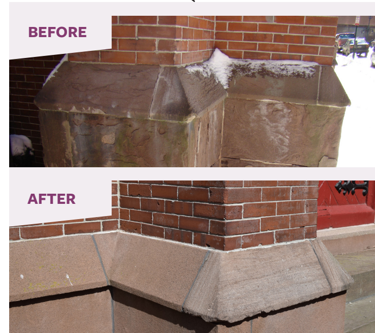
Brownstone is a very soft stone, susceptible to weathering, and the loss of details. Where deterioration was limited, an appropriately formulated patching compound or small dutchman repair was used to make the stones whole again.
