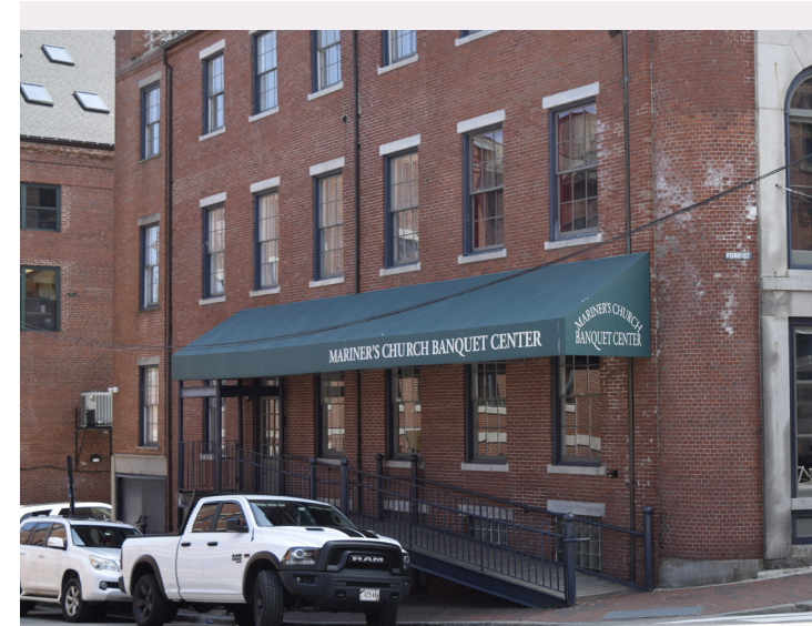
At the Mariner's Church (1828, 366 Fore Street) a new accessible means of entering the building was required. A new metal ramp was designed to be installed along the side elevation. The ramp was built with its own structure system, minimizing the points of connection to the historic structure. The ramp could easily be removed should a better accessibility solution be developed.
