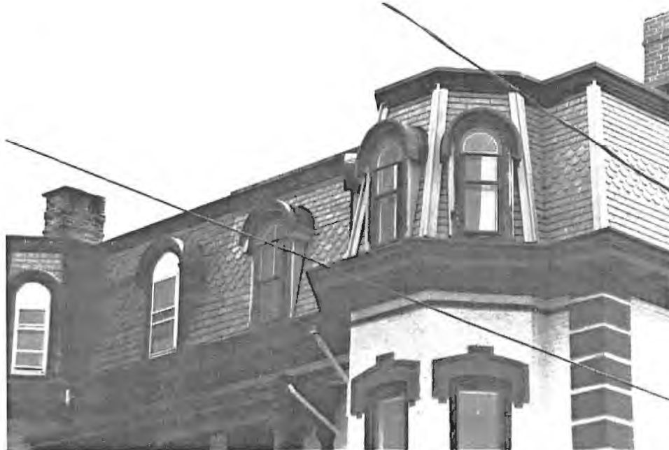
Sometimes a substitute material may be used to replace a deteriorated feature. The mansard roof on this double house retains its original slate on the left side while that on the right side has been replaced with "Supra-Slate", a mineral fiber-shingle product. This new material matches closely the design, color, and texture of the original slate.
