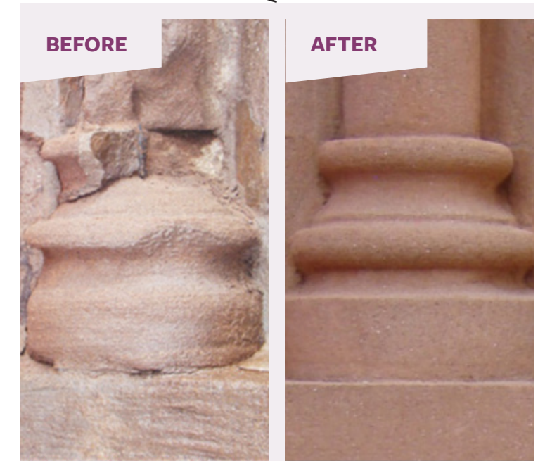
In other, particularly worn areas, the masonry was restored by creating new cast stone pieces, carefully matching the profiles, color, and texture of the original stone.
