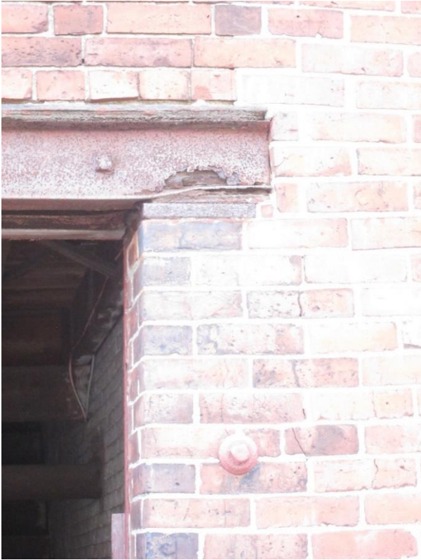
Corroded steel lintel at large door opening on east elevation. Channel is less than three courses deep. Approximately 12" deep in wall face. Note steel seat and return bricks on alternate courses.
