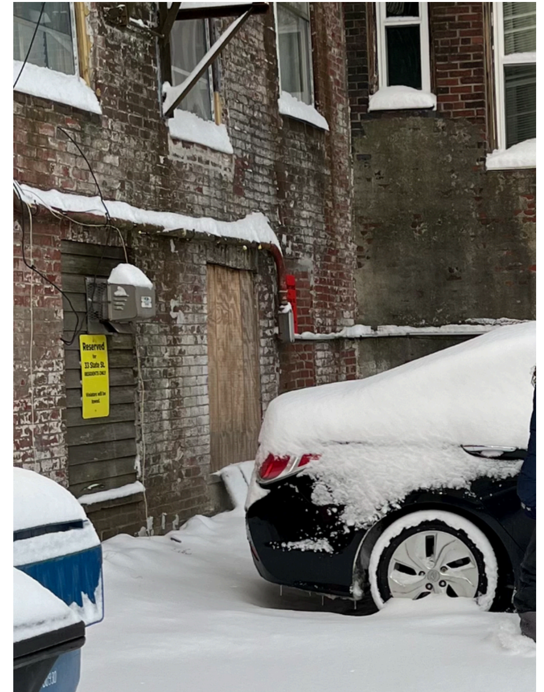
Boarded up windows to 33 State Street Basesment. 1/20/2025
