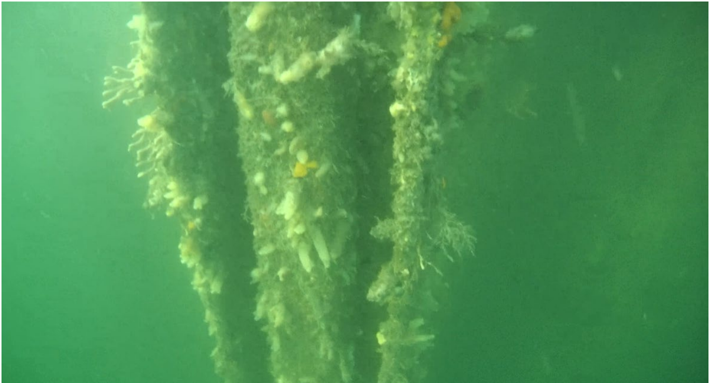
Picture #21 Underwater Drone Photo of Typical Anode of Cathodic Protection System
