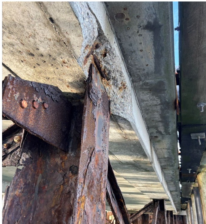
Picture #10 Sercive Pier #3 Bent 4, Pile 1 Cracked Concrete Cap Looking North
