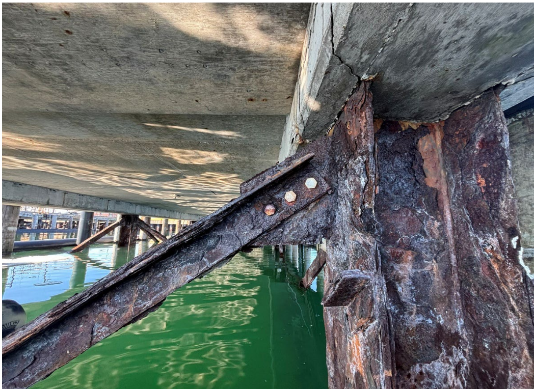
Picture #6 Typical Corrosion on H-Piles, Bracing, and Gussets on Service Pier #3
