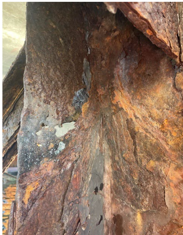
Picture #18 H-pile Corrosion in Service Pier 1.
