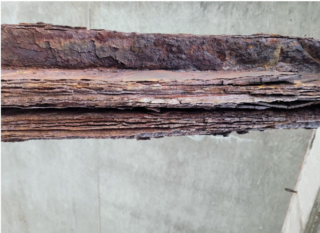
Picture #13 Typical Heavy Corrosion and Scale to Lateral Diagonal Bracing
