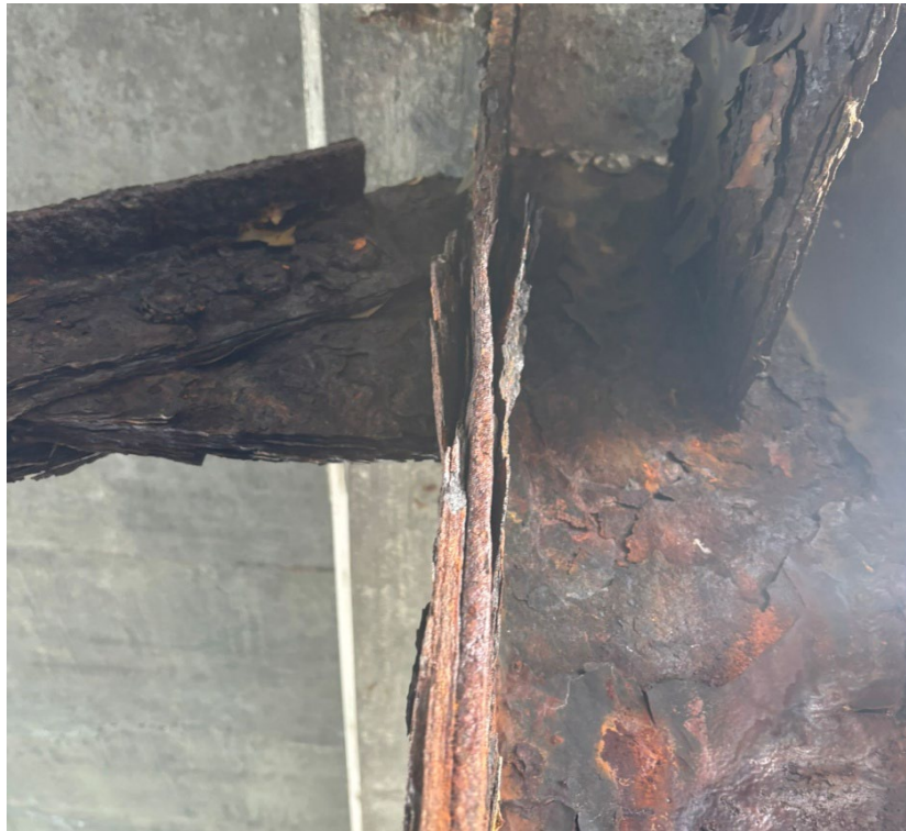
Picture #9 Sercive Pier #3 Bent 2, Pile 2 Local Flange Buckling Looking South
