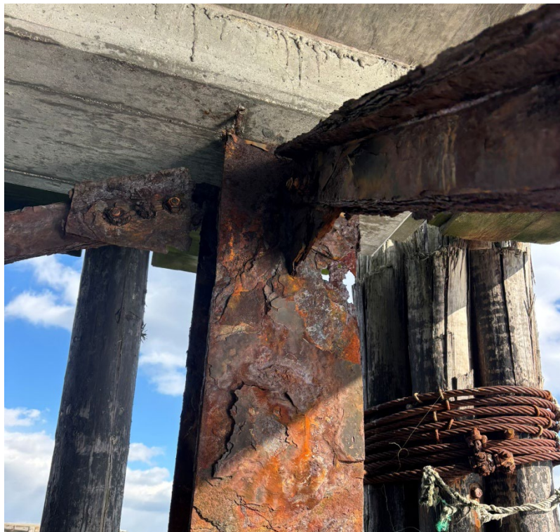
Picture #8 Sercive Pier #3 Bent 6, Pile 1 Corroded Flanges Looking Southeast
