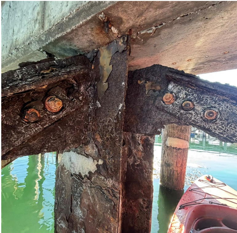
Picture #11 Serivce Pier #1 Bent 2, Pile 2 Flange Corrosion Looking Southwest
