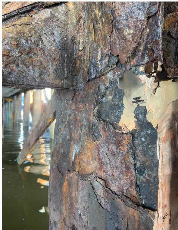
Picture #16 Heavy Corrosion in H-Pile Under Service Pier 3
