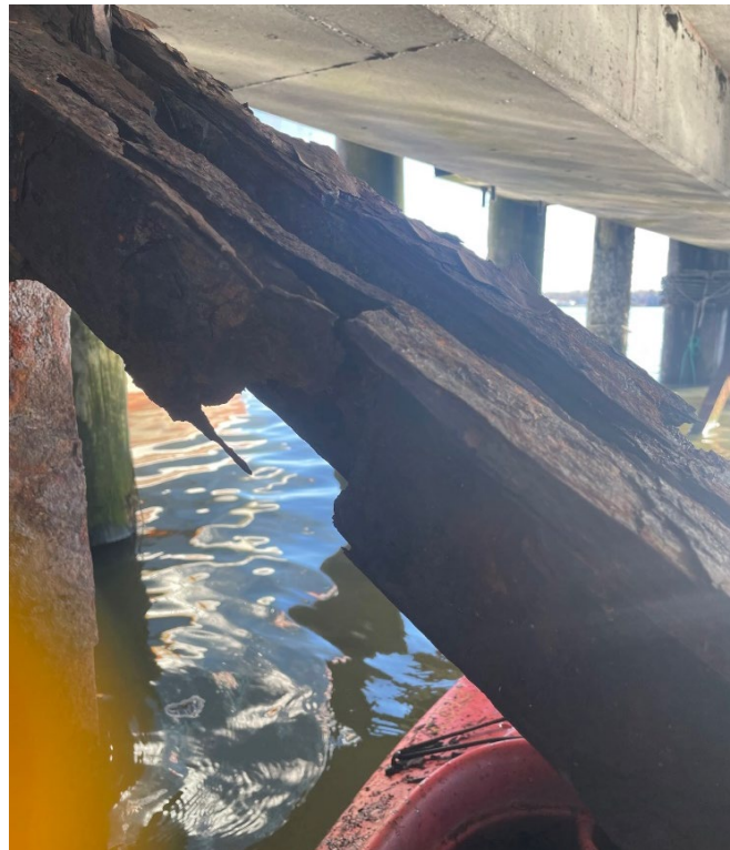
Picture #17 Typical Diagonal Bracing Corrosion (Poor)
