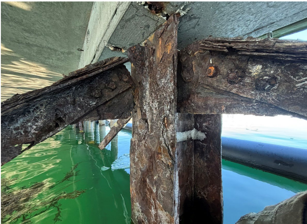
Picture #14 Lateral Diagonal Bracing Corroded and Disconnected at Gusset
