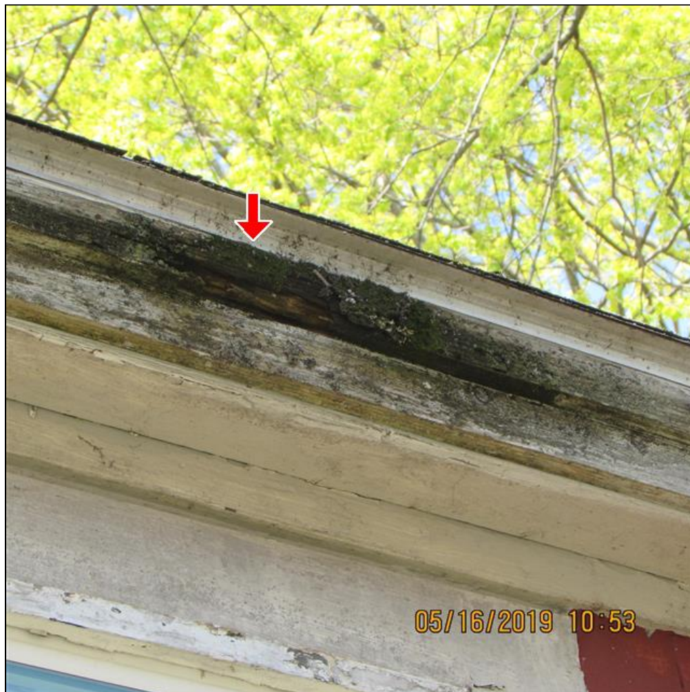
2.1 Item 2(Picture) Fascia rot on right side of home
