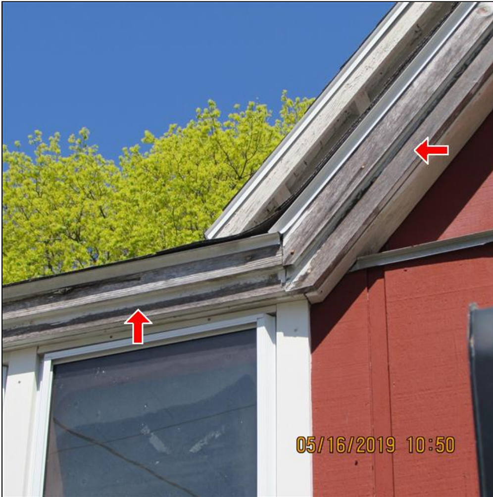
2.1 Item 1(Picture) All fascia boards and trim need paint
