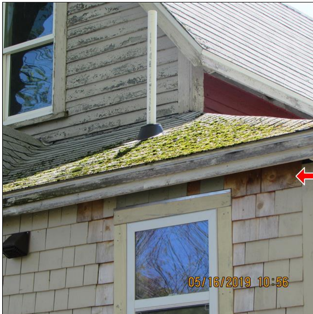
2.0 Item 6(Picture) Keep siding painted
