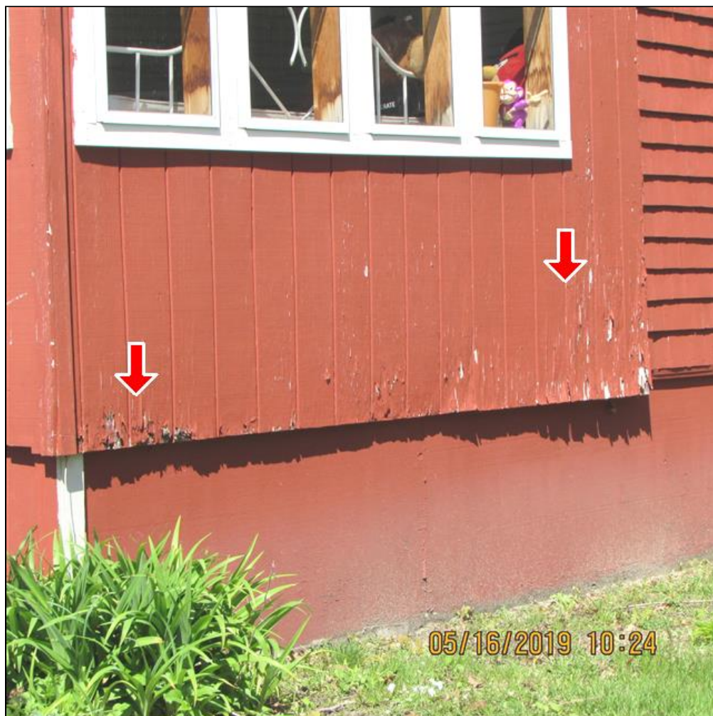
2.0 Item 2(Picture) Siding needs replacement on the right of the front porch
