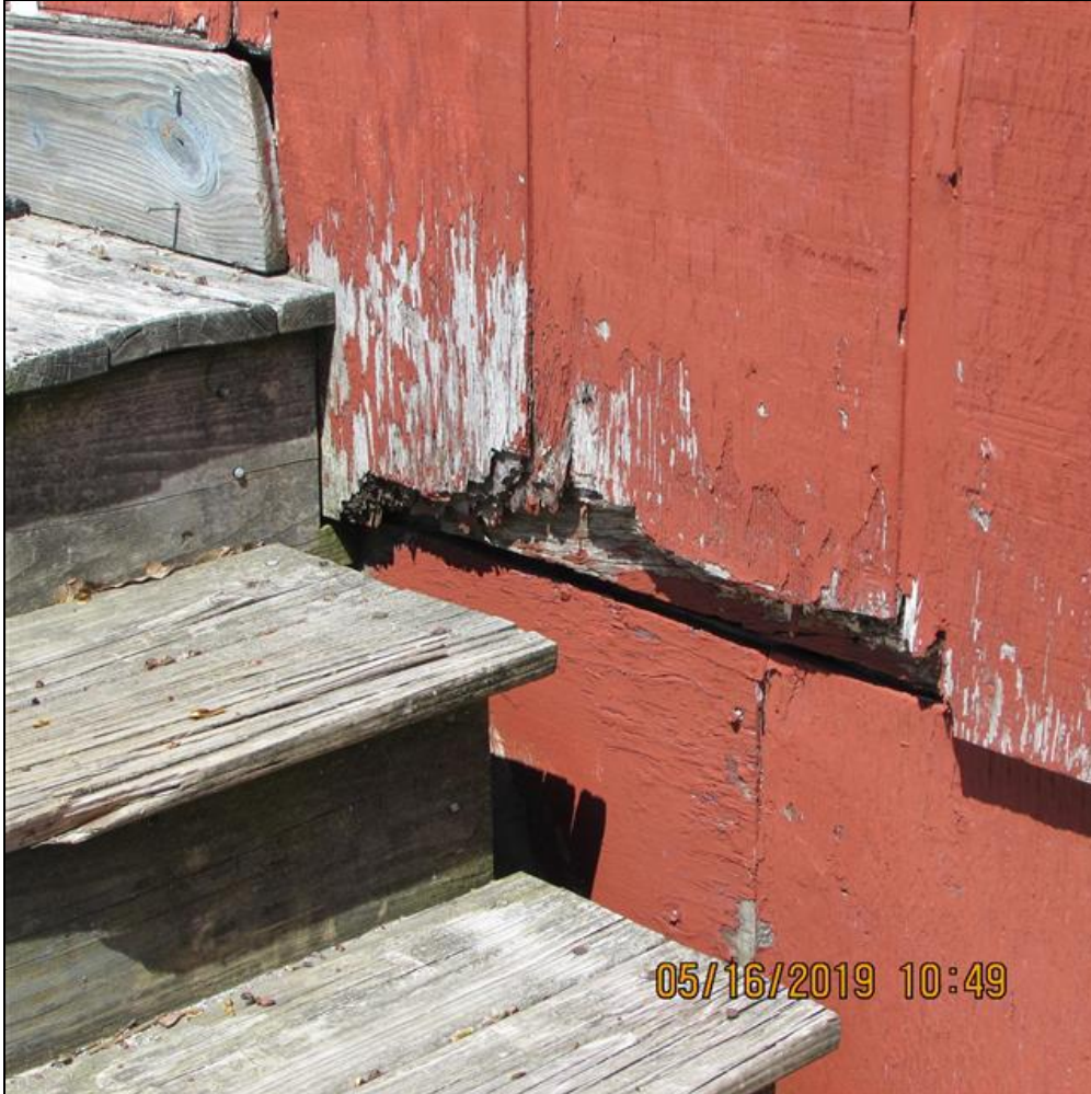
2.0 Item 1(Picture) Siding damage at front
