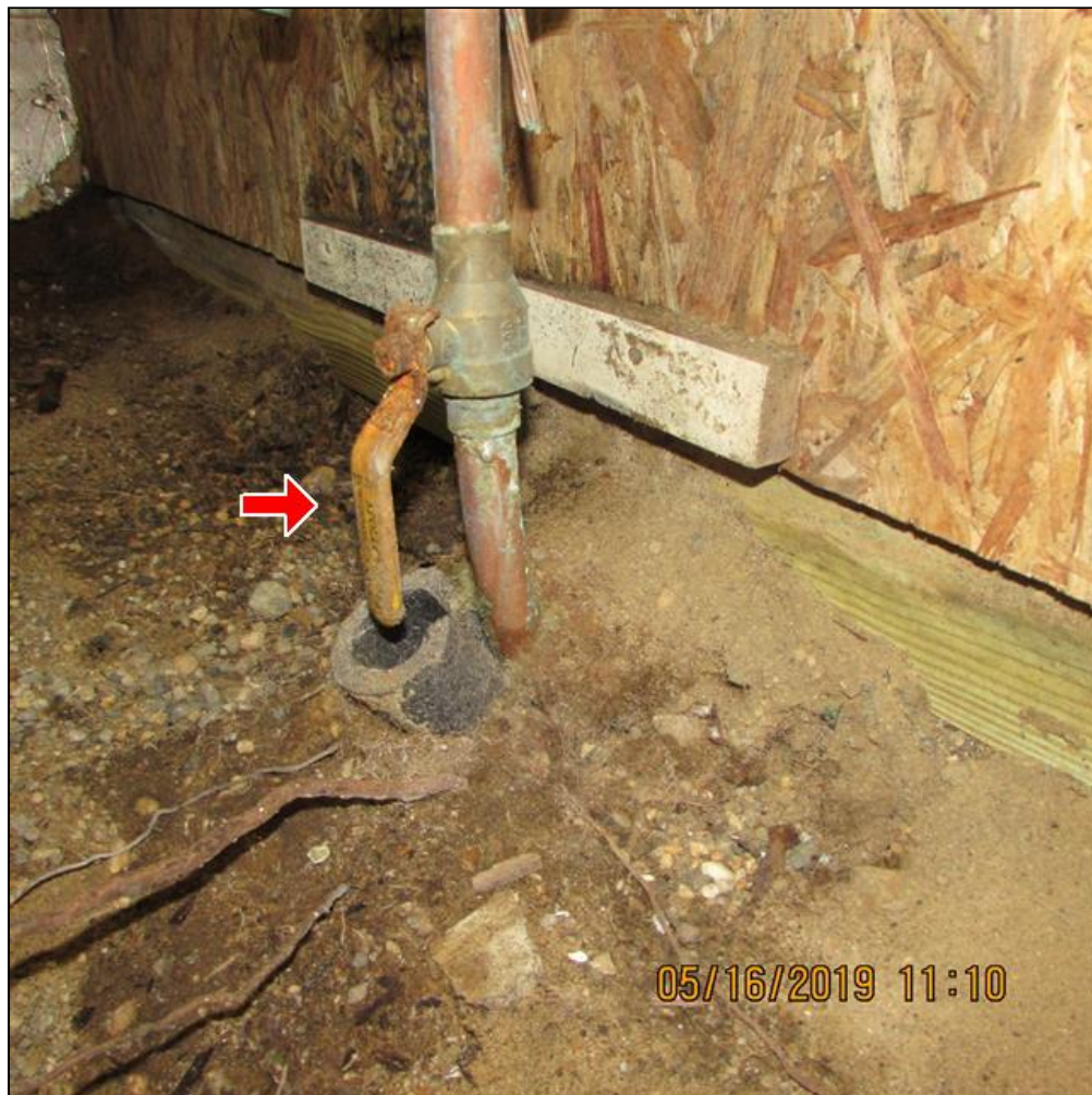
8.0 Item 3(Picture) Main water shut off
