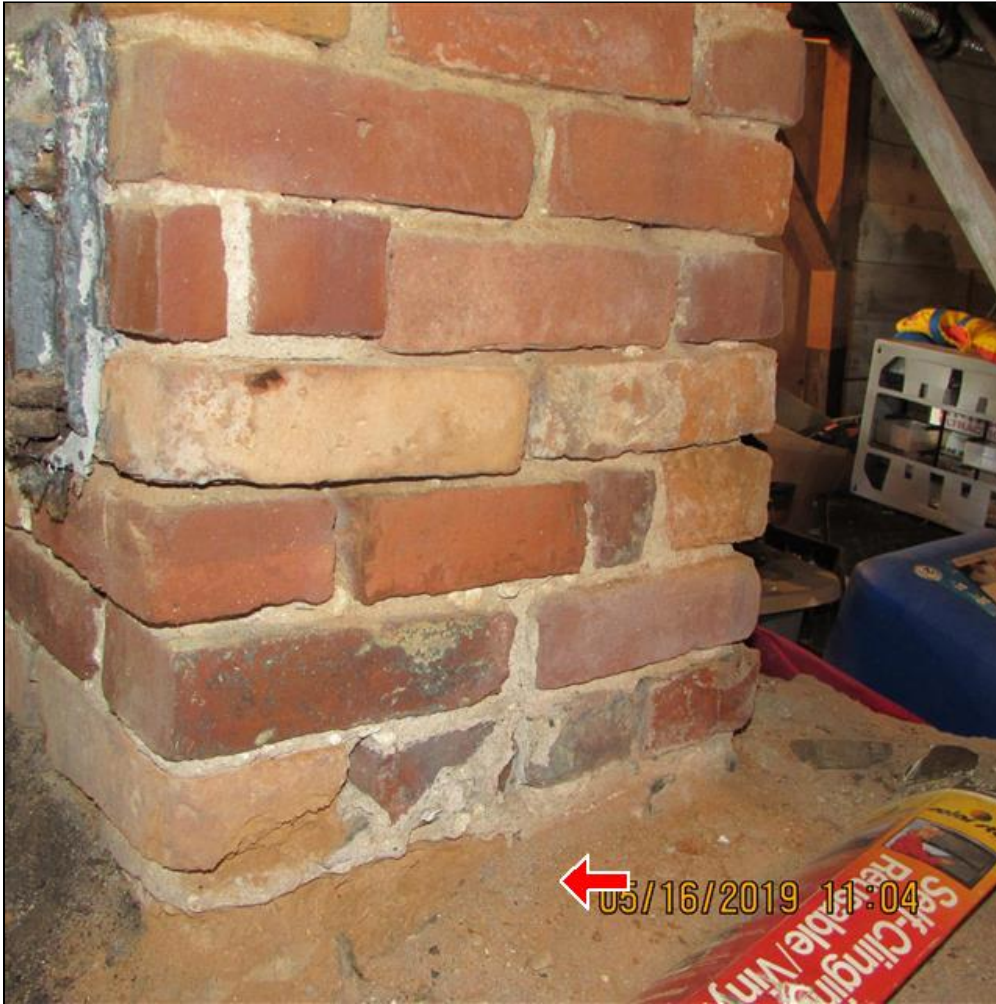
5.2 Item 1(Picture) Spalling chimney in crawlspace
