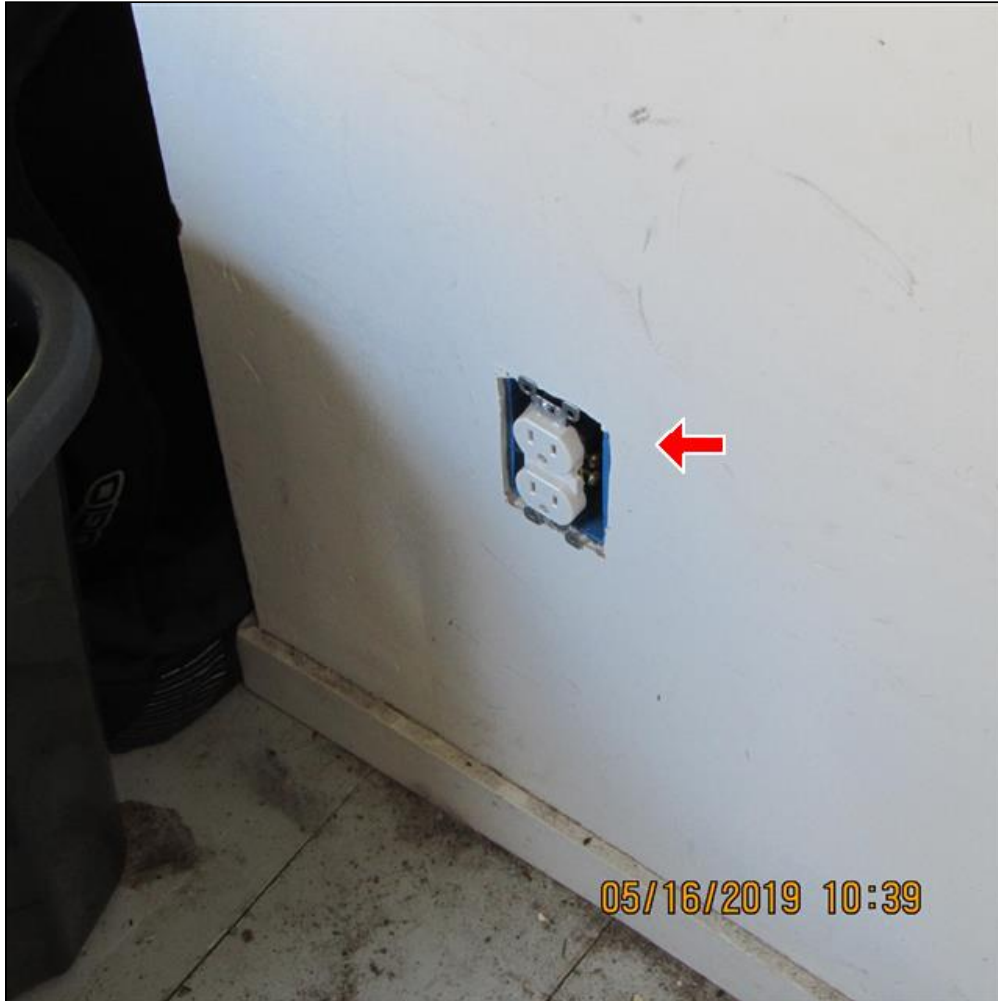
9.3 Item 1(Picture) Cover needed in laundry area
