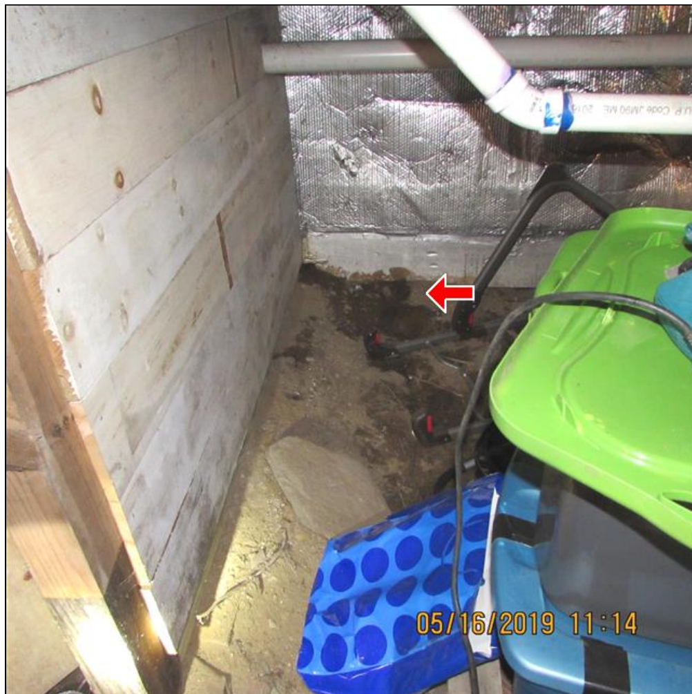
6.0 Item 15(Picture) Water seepage present
