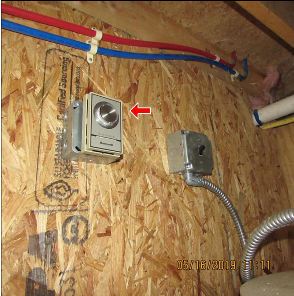
7.0 Item 2(Picture) Thermostat in crawlspace for heat
