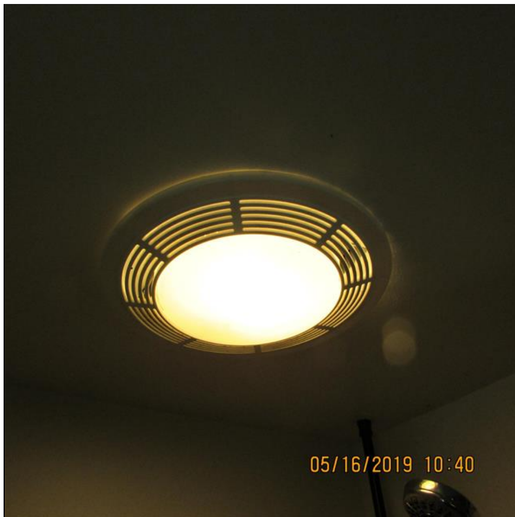
10.5 Item 4(Picture) Bathroom fan is noisy
