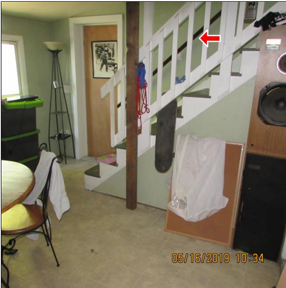
4.3 Item 1(Picture) Balusters should be 4" apart
