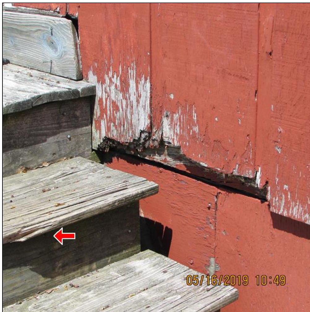
2.4 Item 2(Picture) Replace any damaged wood at front porch
