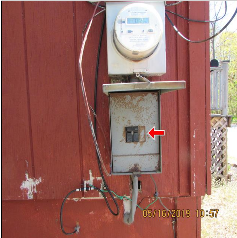
9.1 Item 1(Picture) Main power disconnect
