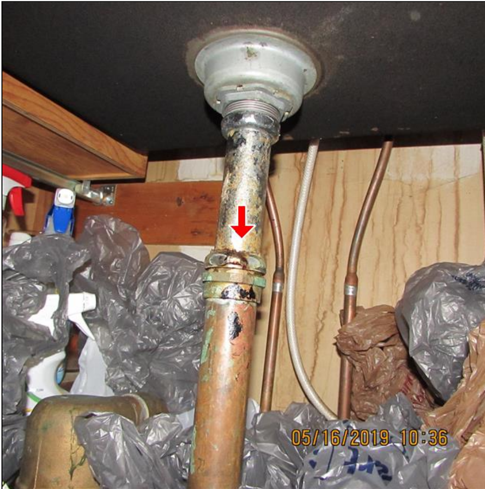
8.1 Item 3(Picture) Repair may be needed here
