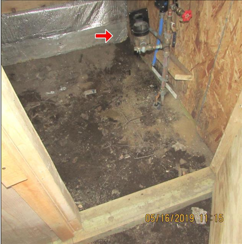
8.0 Item 1(Picture) Water meter
