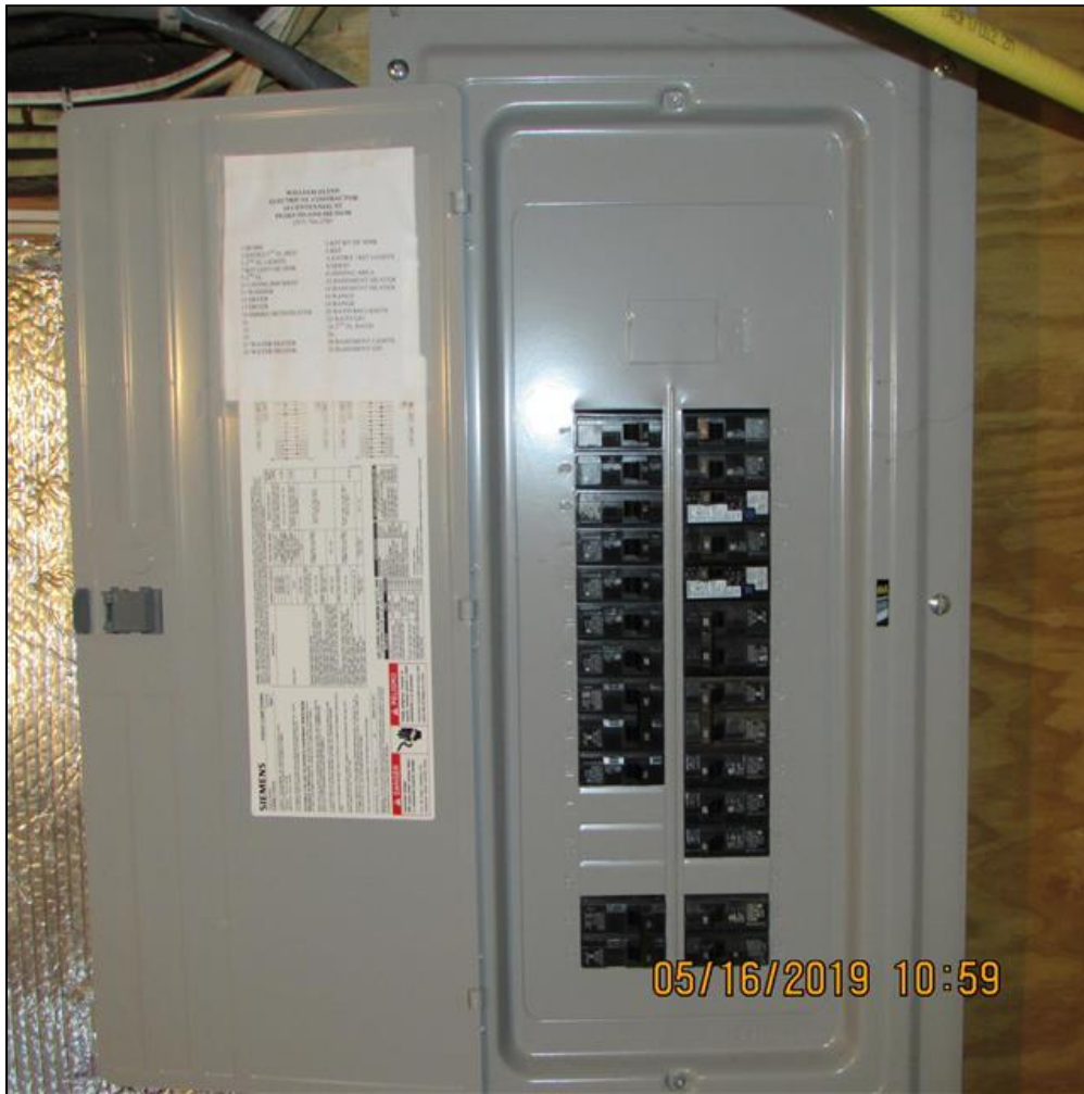
9.1 Item 2(Picture) Panel in crawlspace
