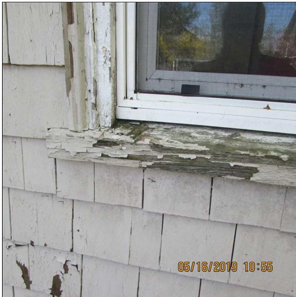
2.3 Item 4(Picture) Rear window
