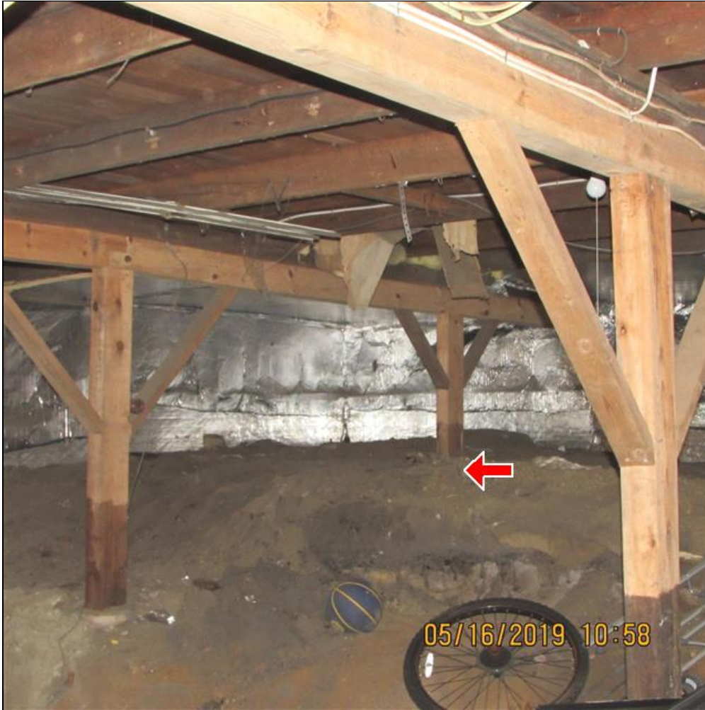
10.3 Item 1(Picture) install a vapor barrier in the crawlspace
