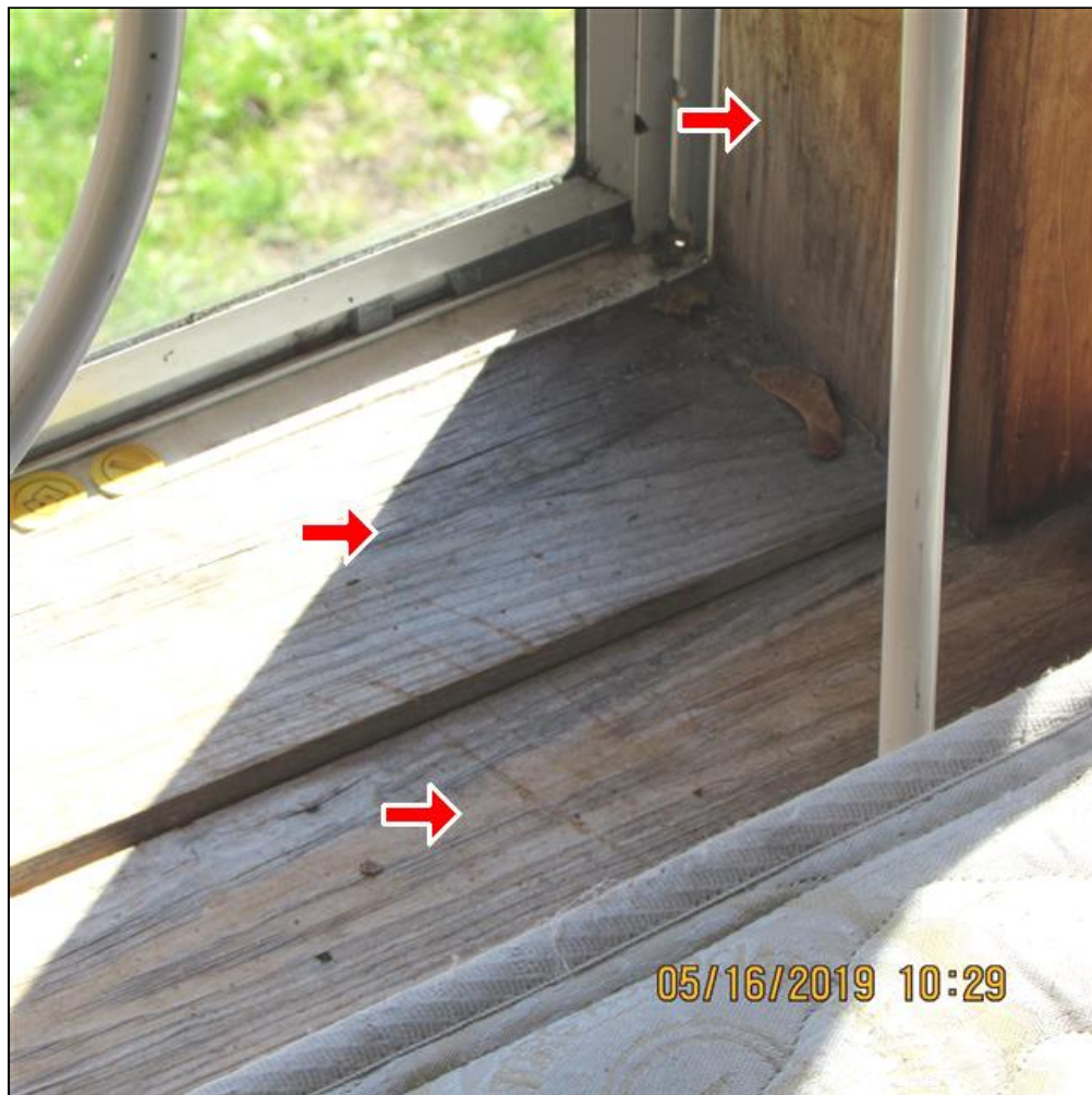
4.6 Item 2(Picture) Porch windows need sealing
