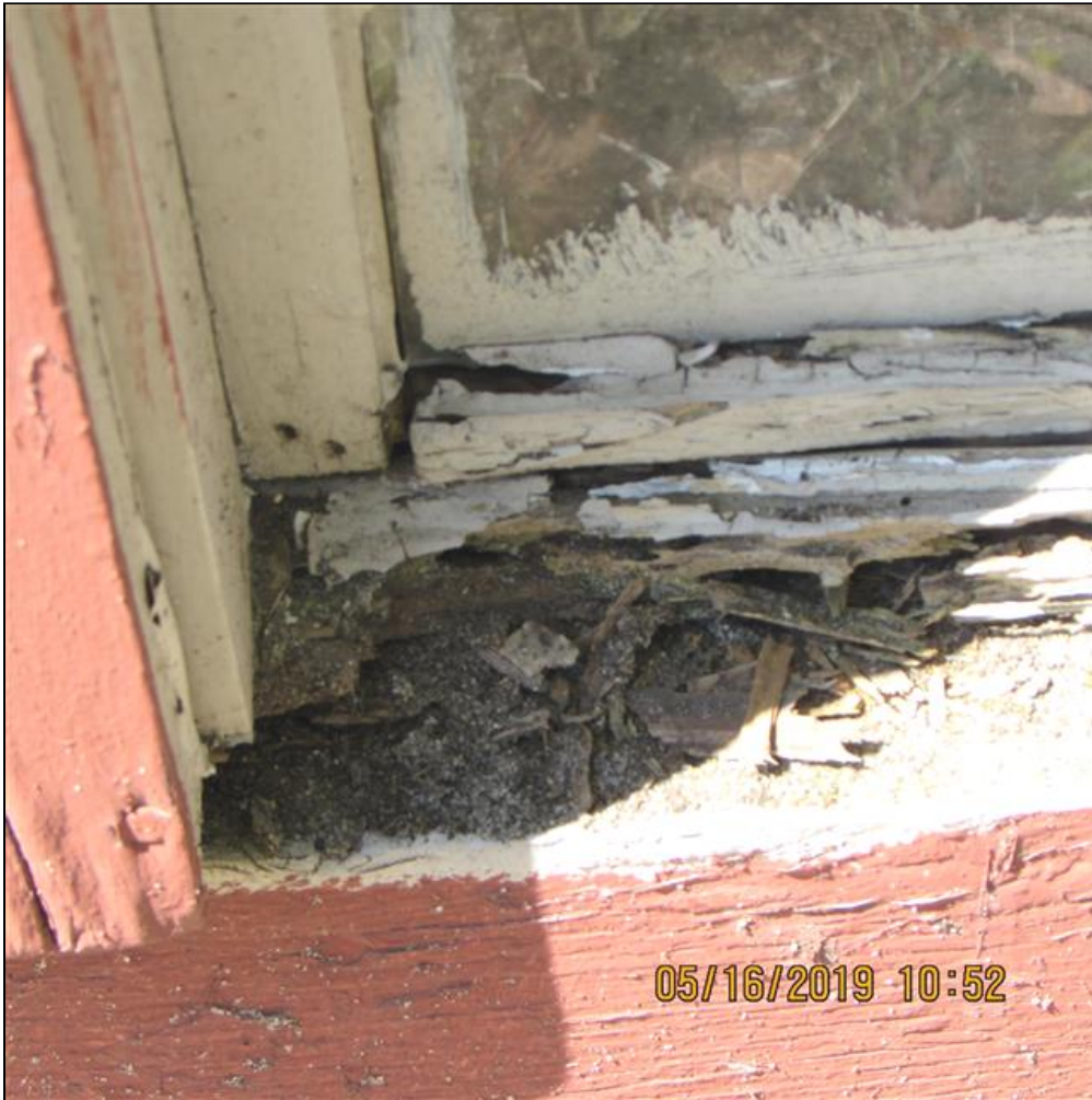
2.3 Item 3(Picture) Basement window rot
