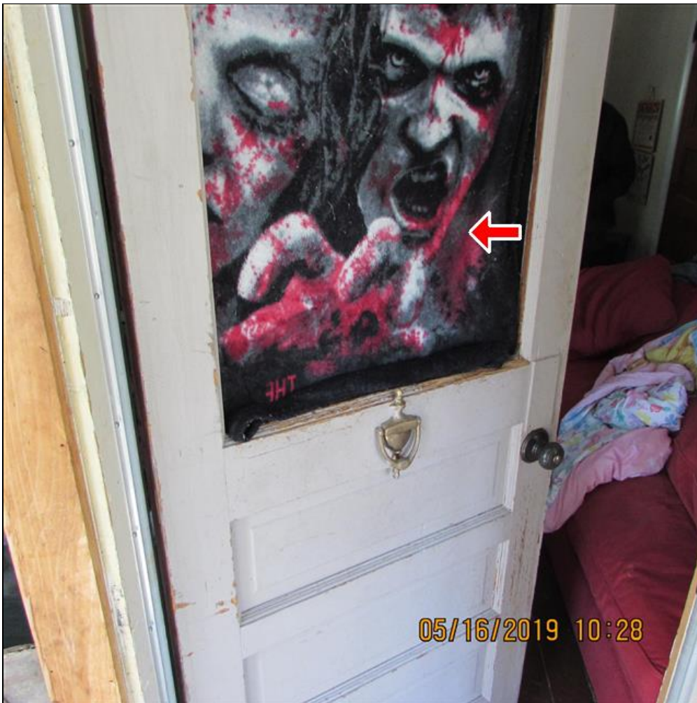
2.2 Item 1(Picture) Window missing in front door
