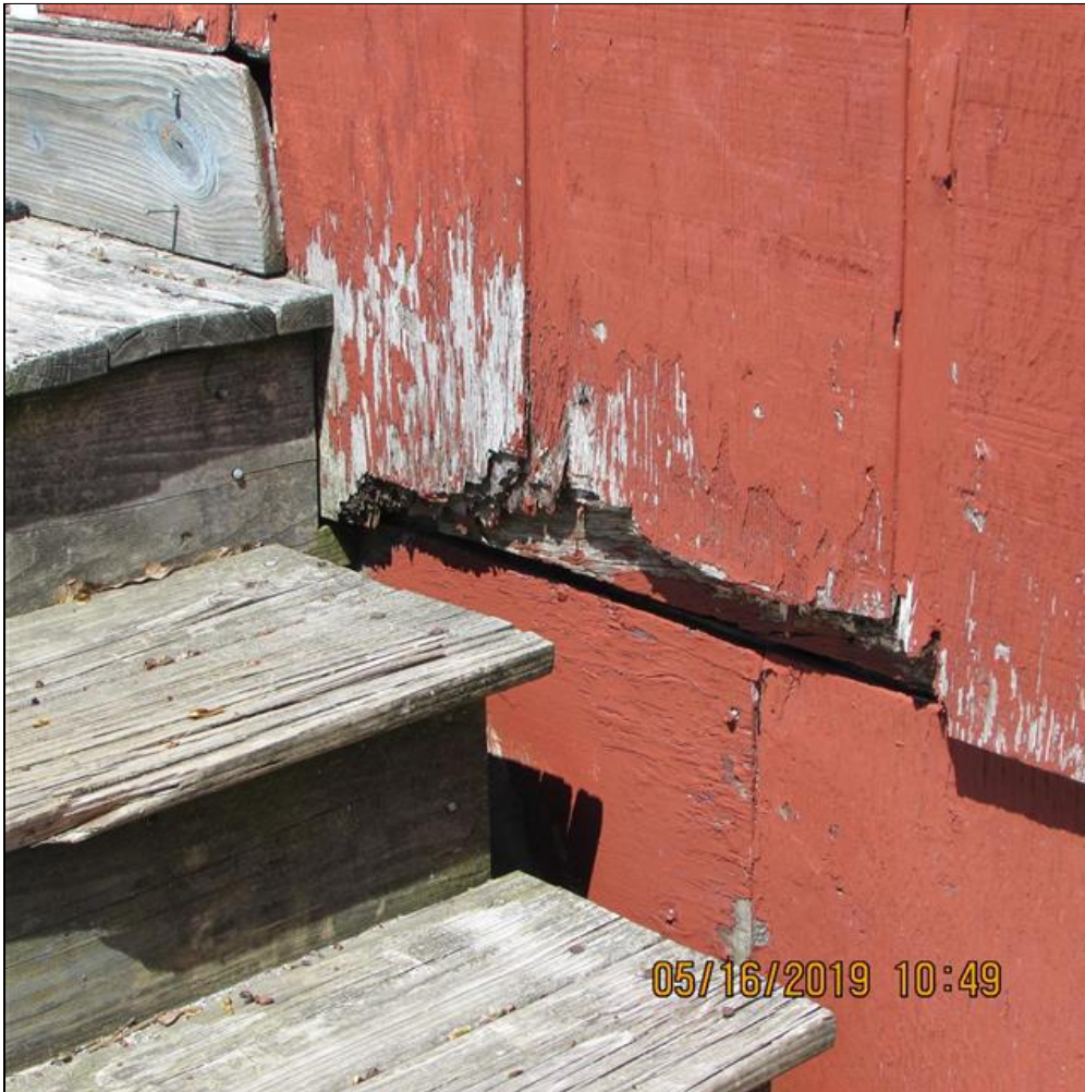
2.0 Item 1(Picture) Siding damage at front
