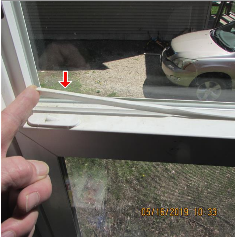
4.6 Item 4(Picture) Loose window trim
