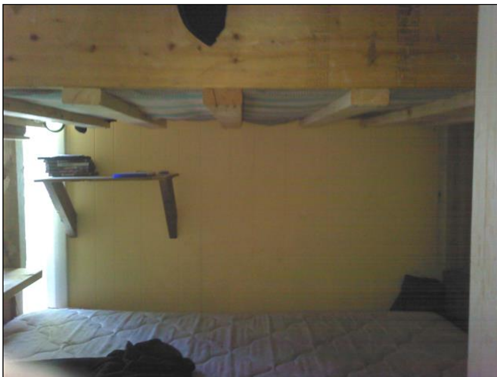
13.0 Item 1(Picture) Bedroom wall without thermal image
