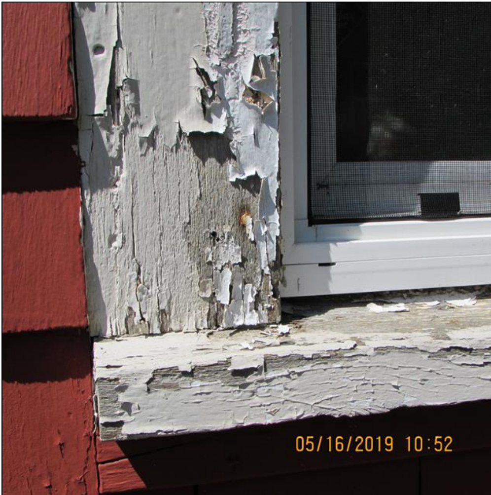
2.3 Item 1(Picture) Exterior windows need paint
