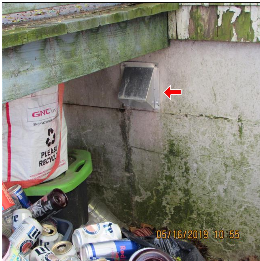
10.5 Item 2(Picture) Dryer duct at rear
