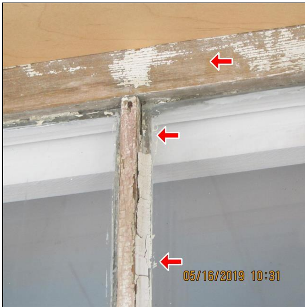
4.6 Item 3(Picture) Paint and glazing compound needed on front porch window
