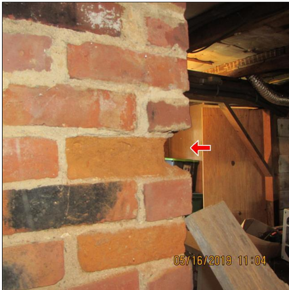
5.2 Item 3(Picture) Chimney deterioration
