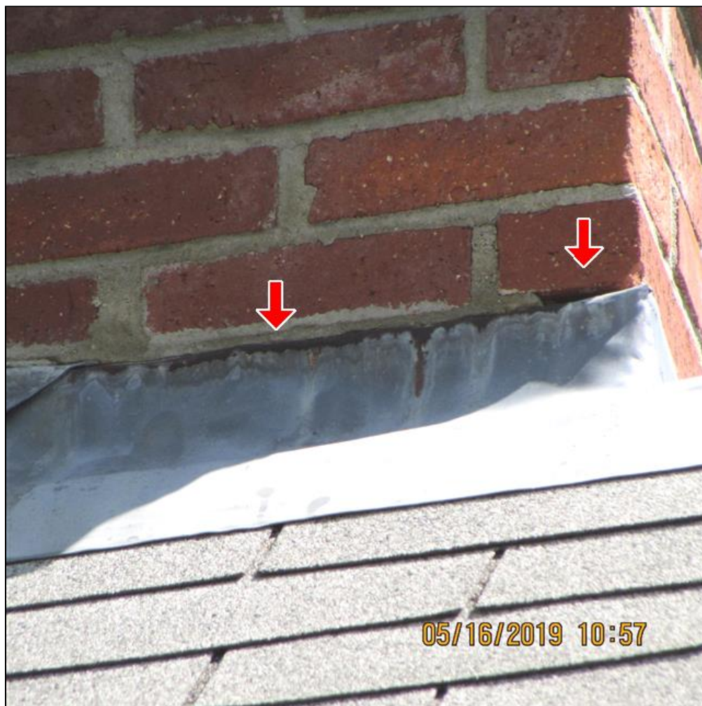
1.2 Item 3(Picture) Rusty chimney flashing and missing mortar
