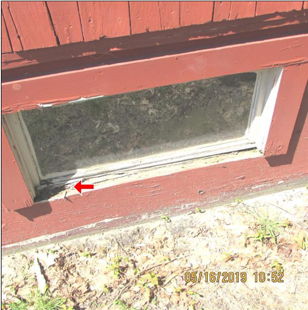
2.3 Item 2(Picture) Basement window rot
