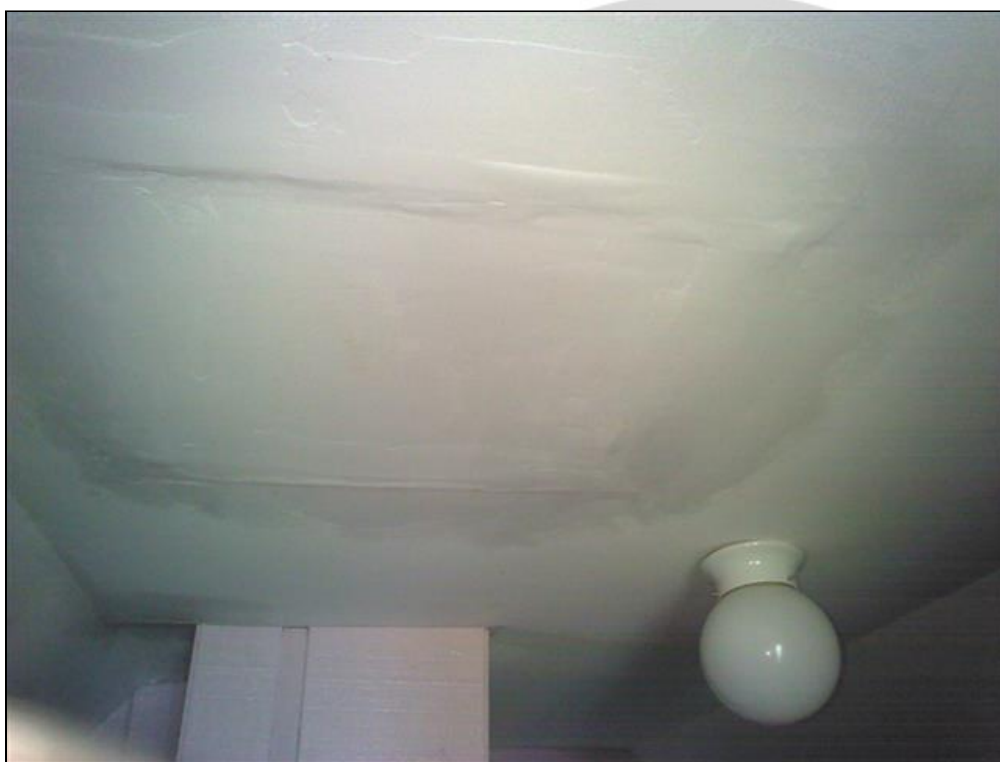
13.0 Item 9(Picture) 2nd floor ceiling patch
