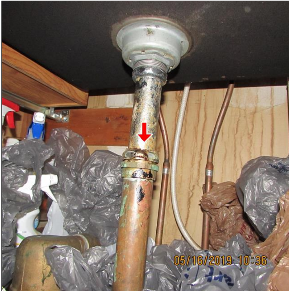
8.1 Item 3(Picture) Repair may be needed here
