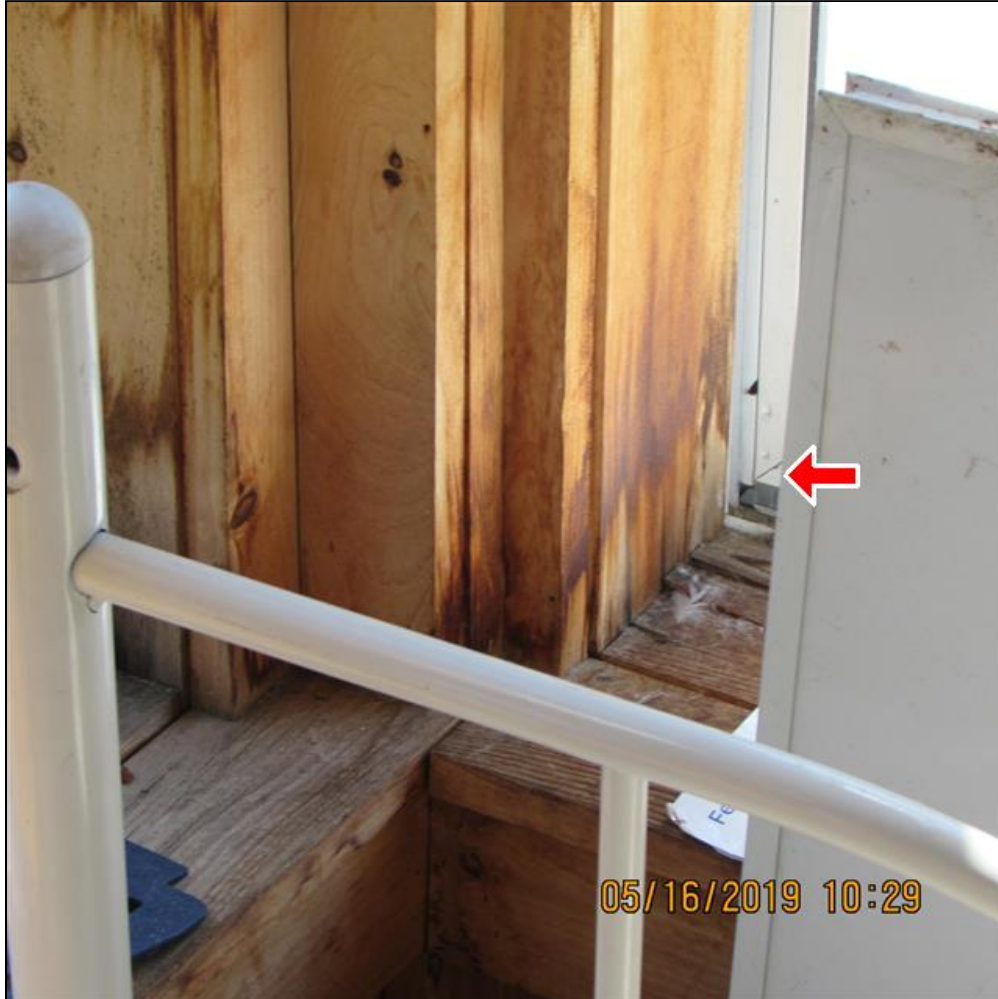
4.6 Item 1(Picture) Water stains on porch window sills
