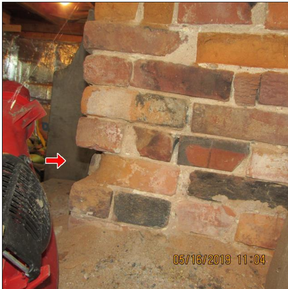
5.2 Item 2(Picture) Chimney is in need of repair
