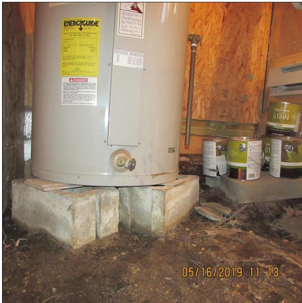
8.3 Item 2(Picture) Hot water heater
