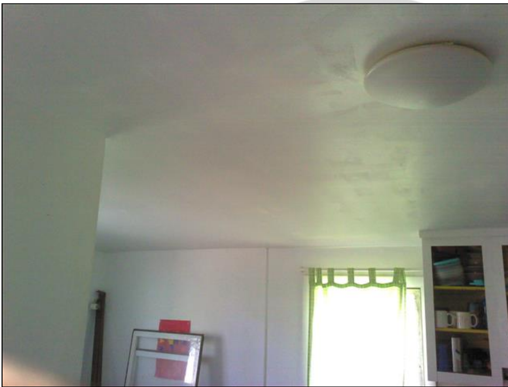
13.0 Item 3(Picture) Addition ceiling without thermal image
