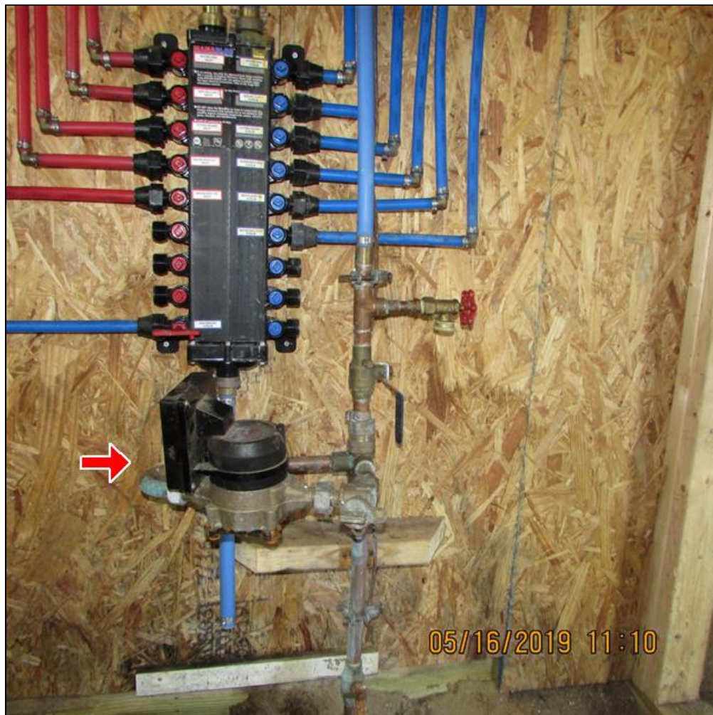
8.0 Item 2(Picture) Water meter
