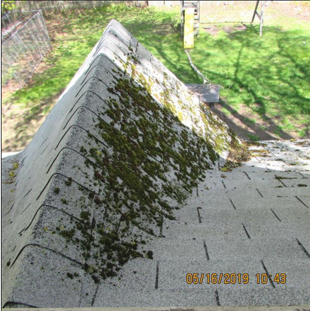
1.0 Item 1(Picture) Moss on roofing
