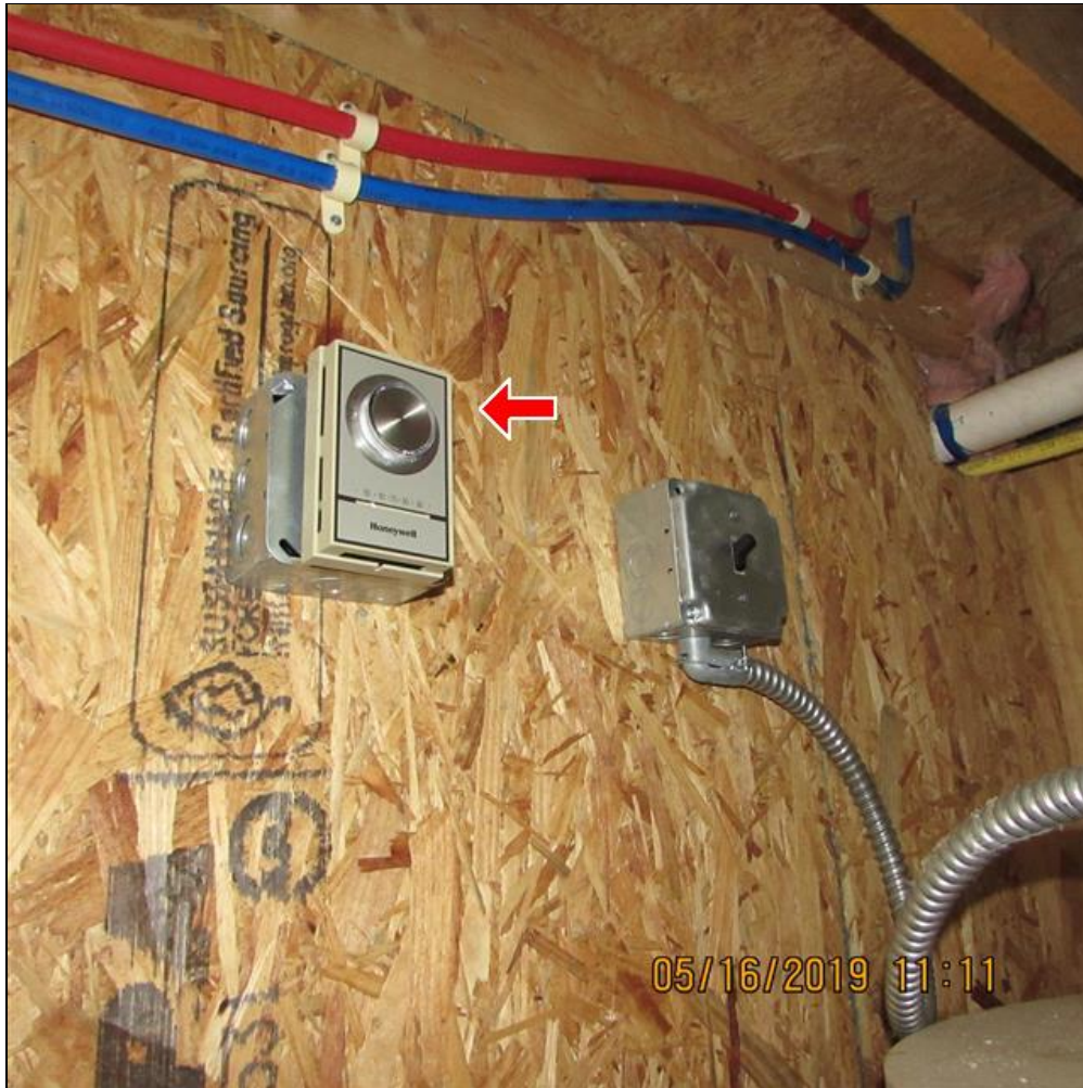
7.0 Item 2(Picture) Thermostat in crawlspace for heat
