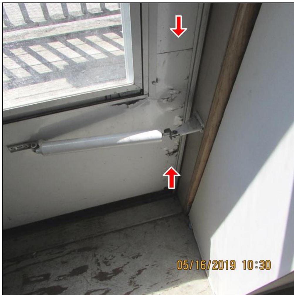
2.2 Item 2(Picture) Storm door damage and wear
