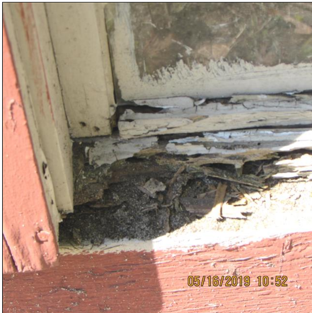
2.3 Item 3(Picture) Basement window rot
