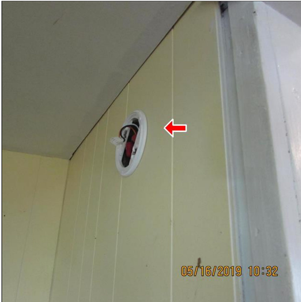
9.7 Item 1(Picture) Replace missing smoke detectors
