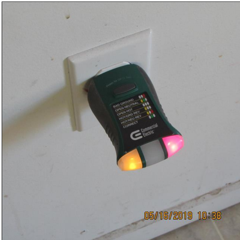
9.3 Item 3(Picture) Reversed polarity outlets need repair
