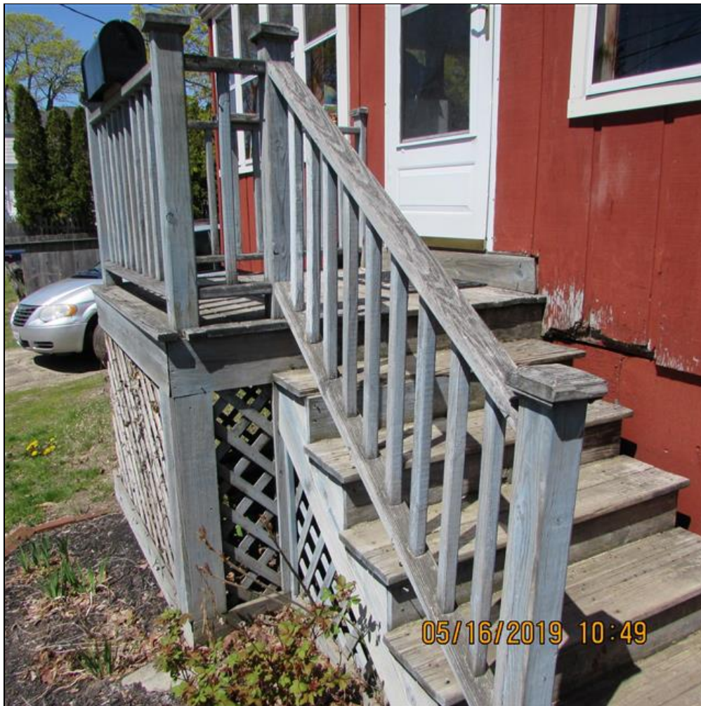
2.4 Item 1(Picture) Stain or paint needed
