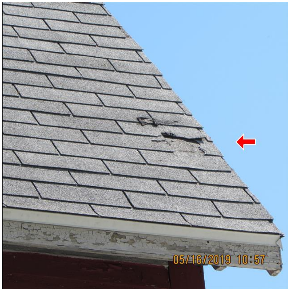
1.0 Item 5(Picture) Shingle damage on left side of home
