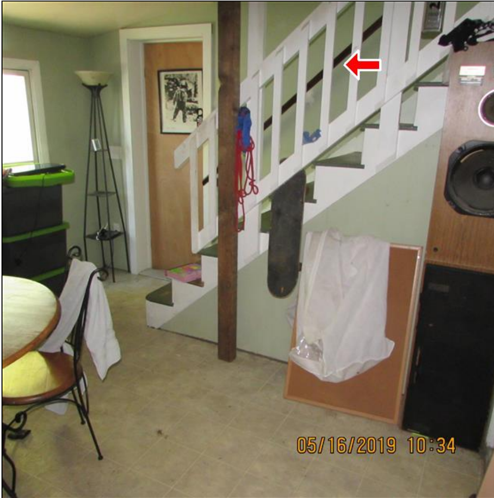
4.3 Item 1(Picture) Balusters should be 4" apart
