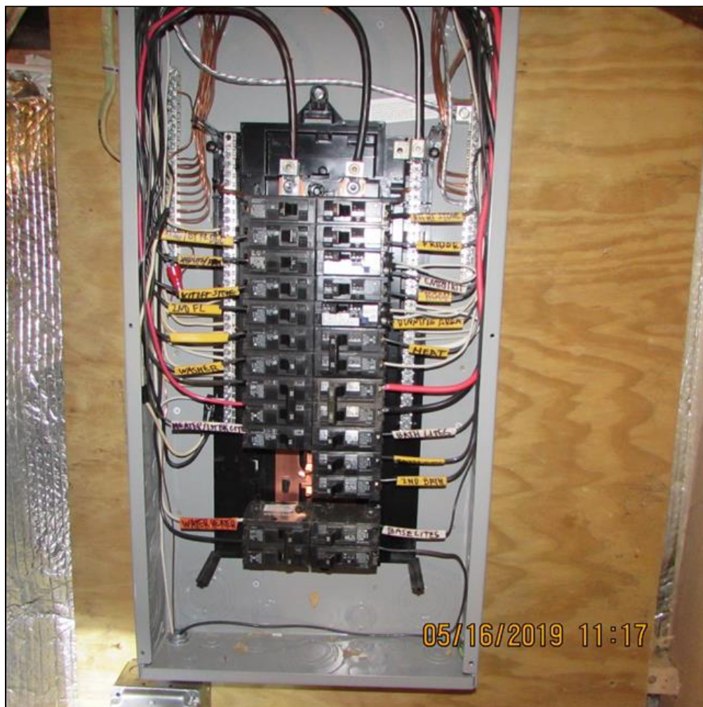
9.1 Item 4(Picture) Distribution panel in crawlspace
