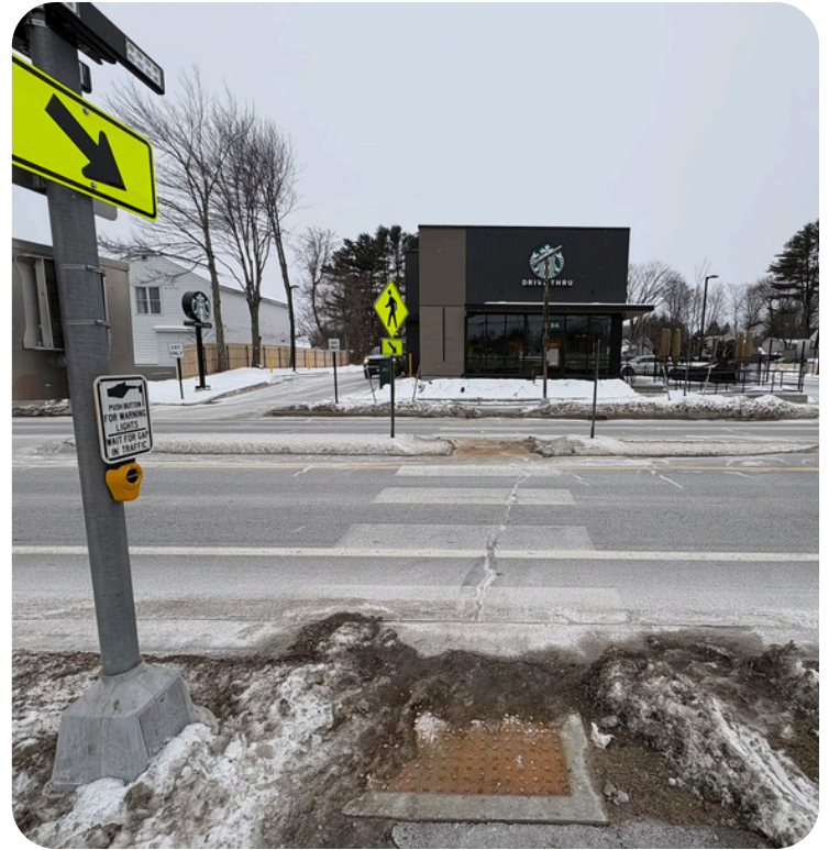
STARBUCKS 84 AUBURN STREET New signalized crossing with median refuge island, sidewalks, and landscaping
