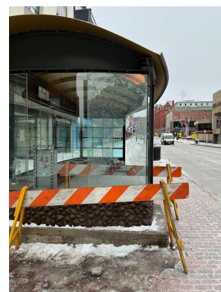
Image of damage at Jewel Box on January 25, 2025.
