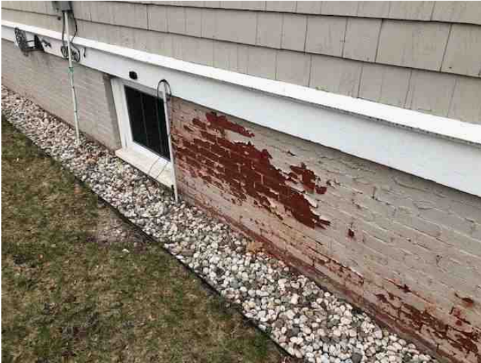
Brick foundation has chipping paint
