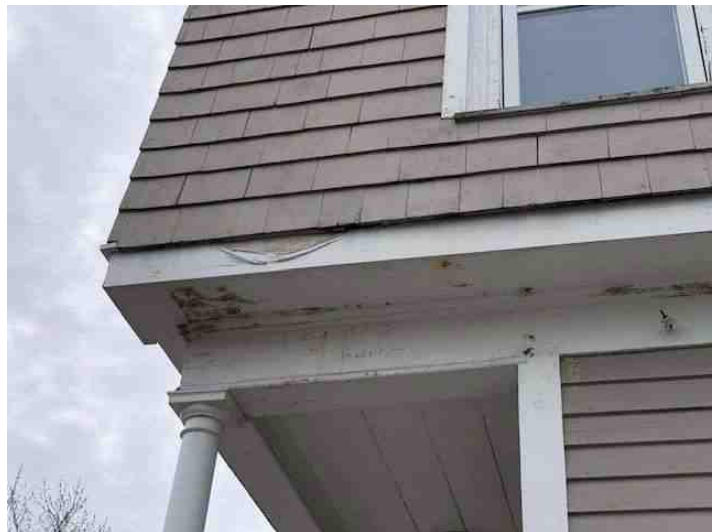
Exposed wood and chipping paint on trim
