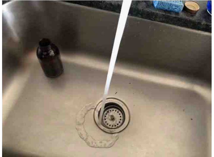
Utilities/mechanicals were on and appear to be working at the time of inspection
