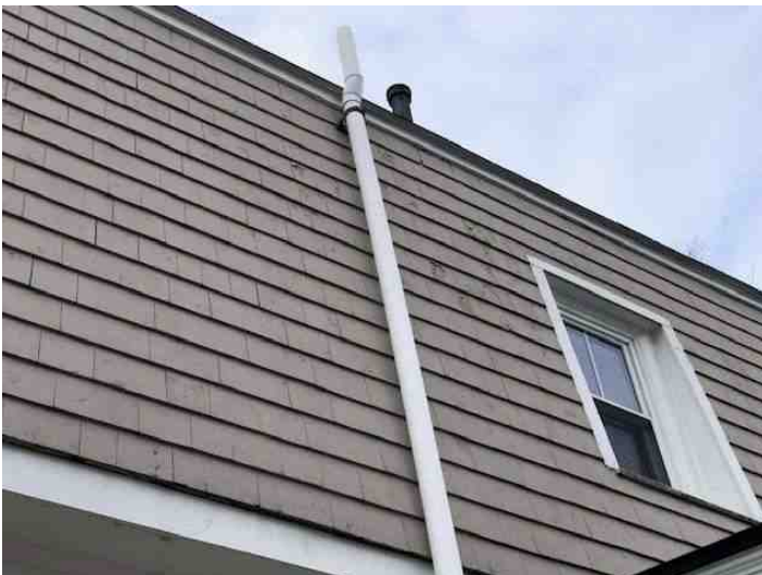
Exposed wood and chipping paint on siding
