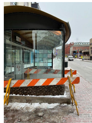
Image of damage at Jewel Box on January 25, 2026.
