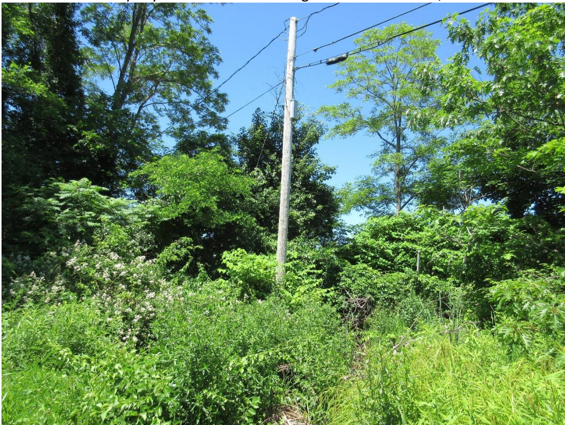
Photo 2: Existing utility pole on the west side of the property overgrown with vegetation.
