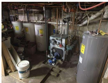
Water and Heating Utility
