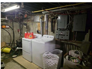
Unit 2 Laundry and Panels
