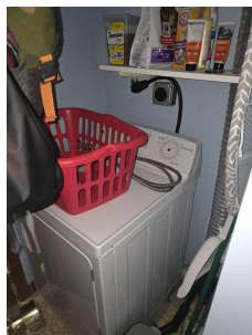
Unit 1 Laundry Utility
