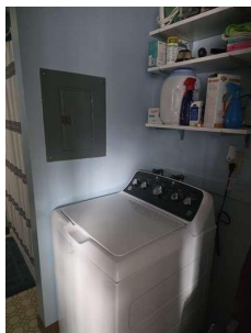
Unit 1 Laundry Utility
