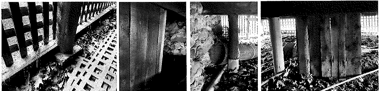
Photograph 3 : Structural deficiencies. There is no foundation, tree posts on blocks and support walls in direct contact with the ground make up most of the building support.
