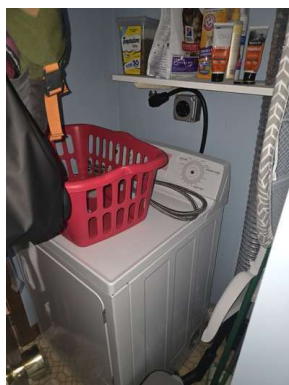
Unit 1 Laundry Utility
