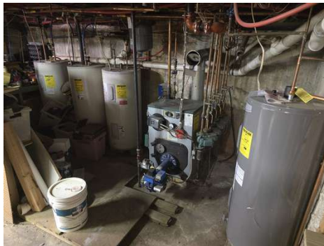
Water and Heating Utility
