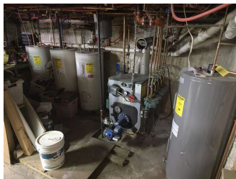
Water and Heating Utility
