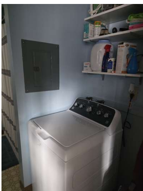
Unit 1 Laundry Utility
