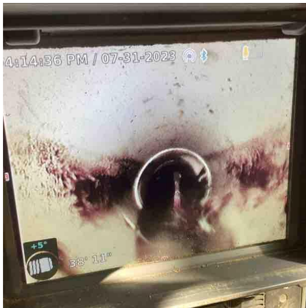
Pipe burst observed at 5 ft depth
