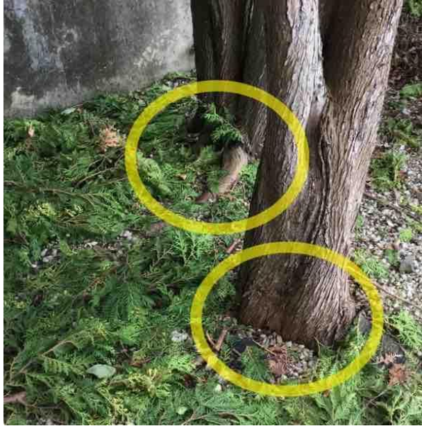
Root system growing into and around trees adjacent to the foundation
