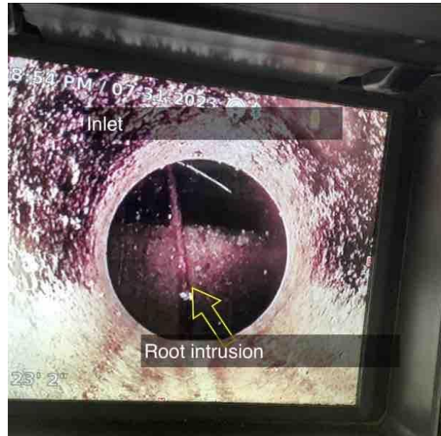
Root intrusion visible in inlet pipe
