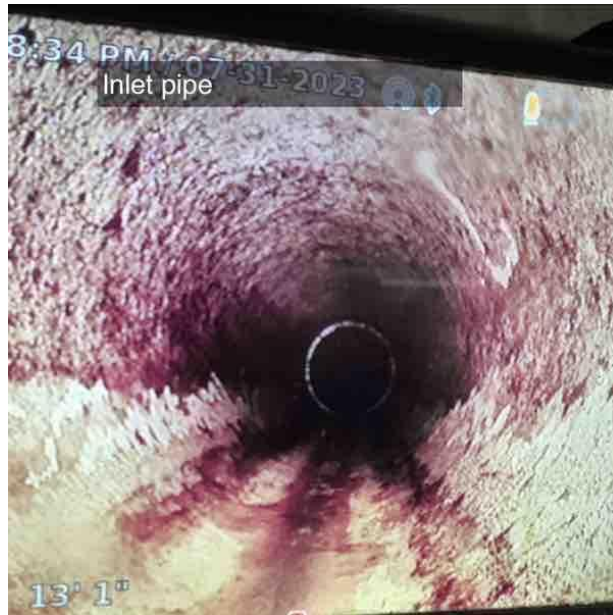
Inlet pipe break at 13 ft
