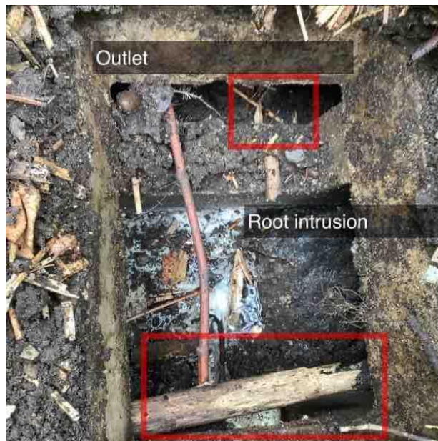
Outlet pipe — root intrusion confirmed
