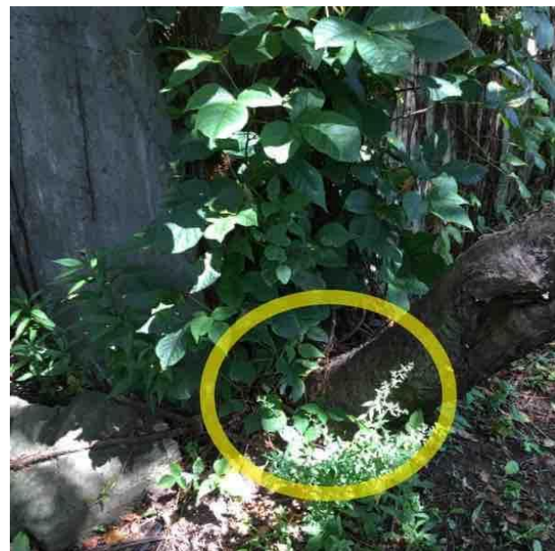
Roots growing into foundation wall
