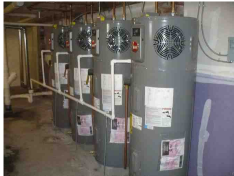
Hot Water Heaters
