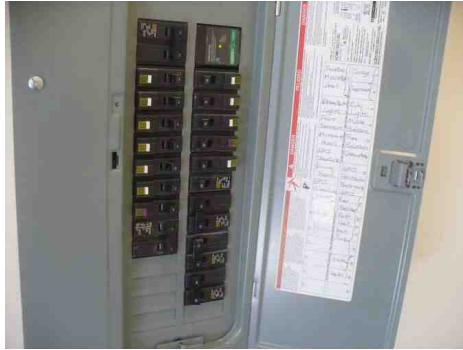
Unit 2 Electrical Panel
