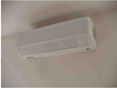
Unit 1 Heat Pump
