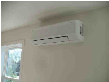
Unit 3 Heat Pump
