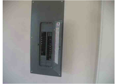
Unit 1 Electrical Panel
