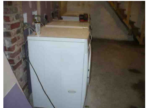
Basement Common Laundry
