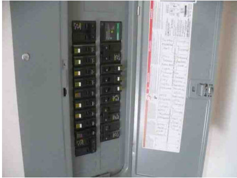
Unit 3 Electrical Panel
