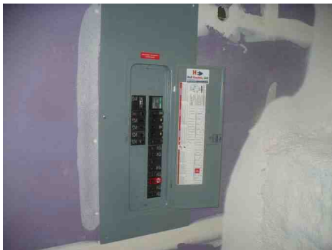
Electrical Panel (House)
