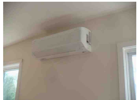
Unit 2 Heat Pump
