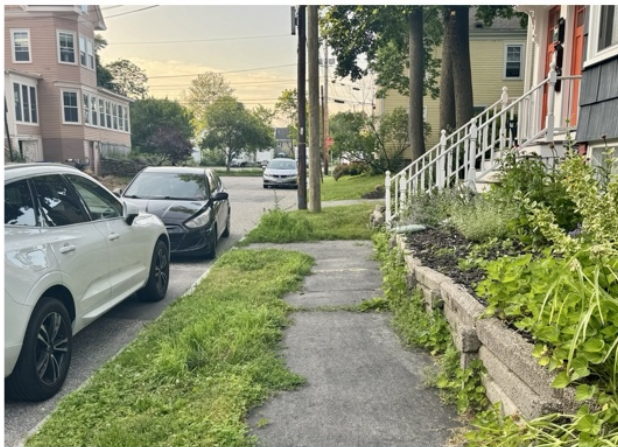
BROKEN / NARROW ASPHALT PATH
