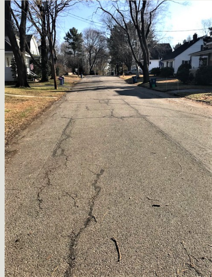
Grafton Street – PCI = 76; ranked Fair 1.5" overlay treatment recommendation
