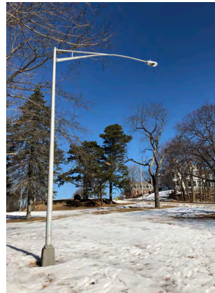
(top) Existing street lighting and walkway lighting
