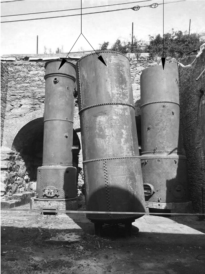
BLDG 15: WATER TANK AND BOILERS
