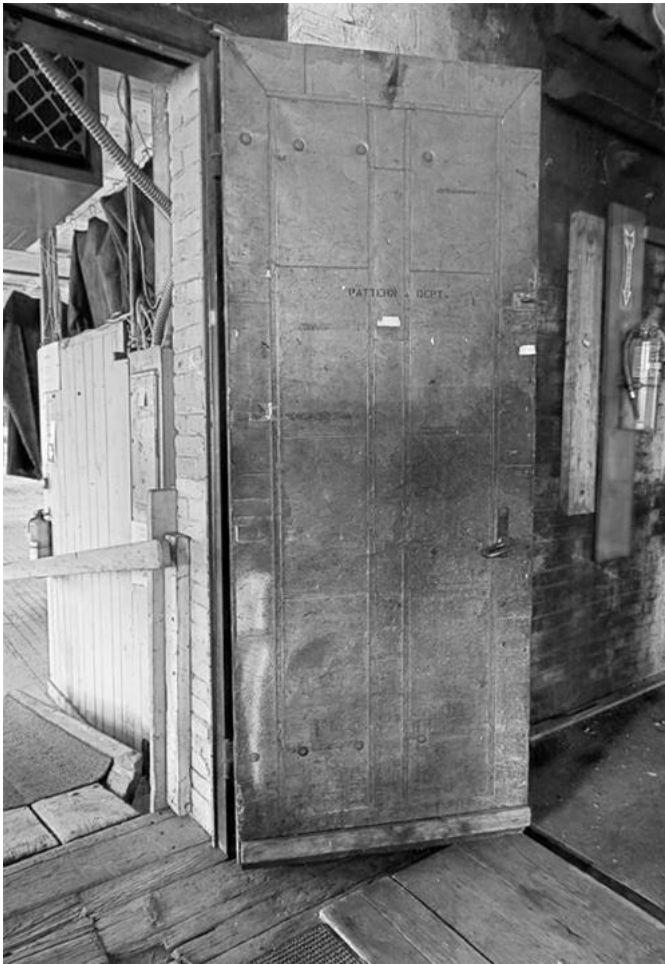
BLDG 2/3: STEEL SWING DOOR SECOND FLOOR
