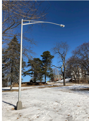
(top) Existing street lighting and walkway lighting
